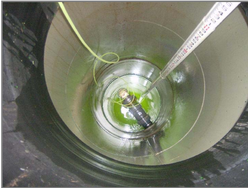
Water level paused at the leaky connection.
