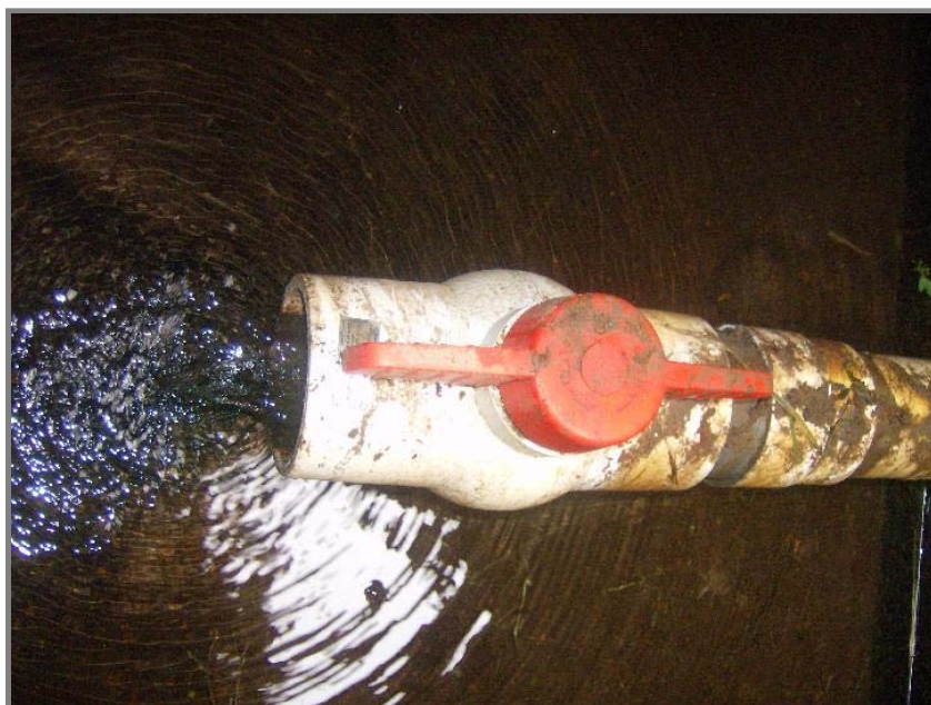
First pipe inside the vault, looking for green water. No green water.
