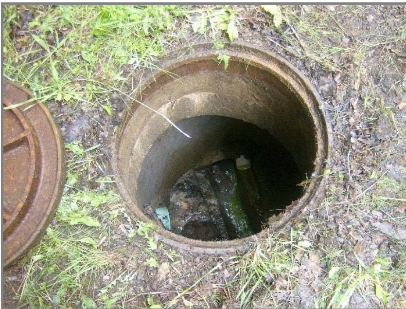
From the surface. Even standing over the manhole the green dye can be seen.
