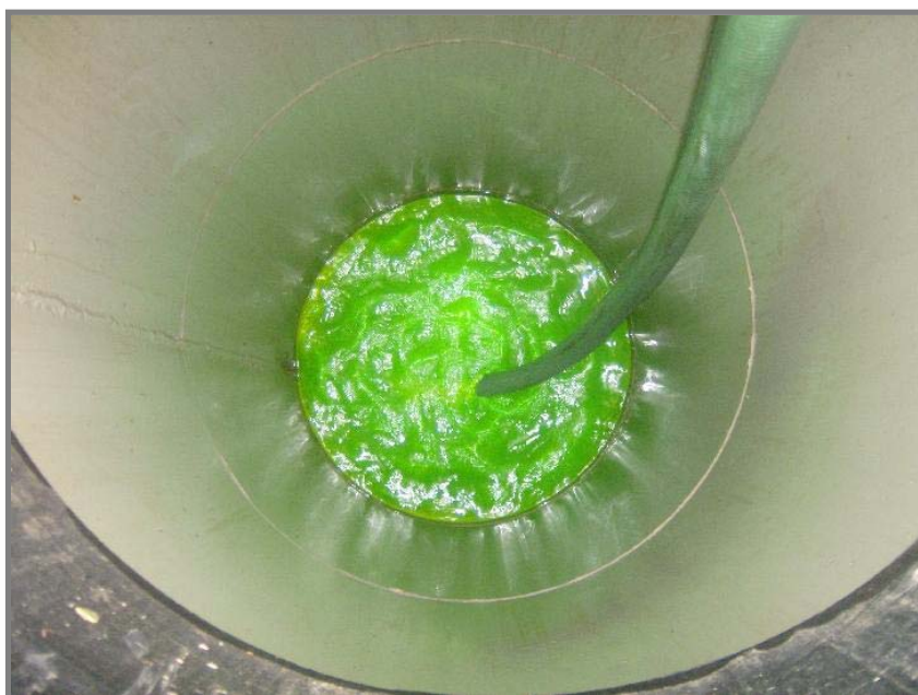
Looking into the manway riser almost pumped down makes for a surreal image.
