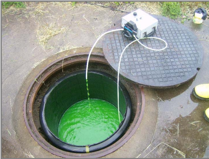
Manway riser and peristaltic pump
