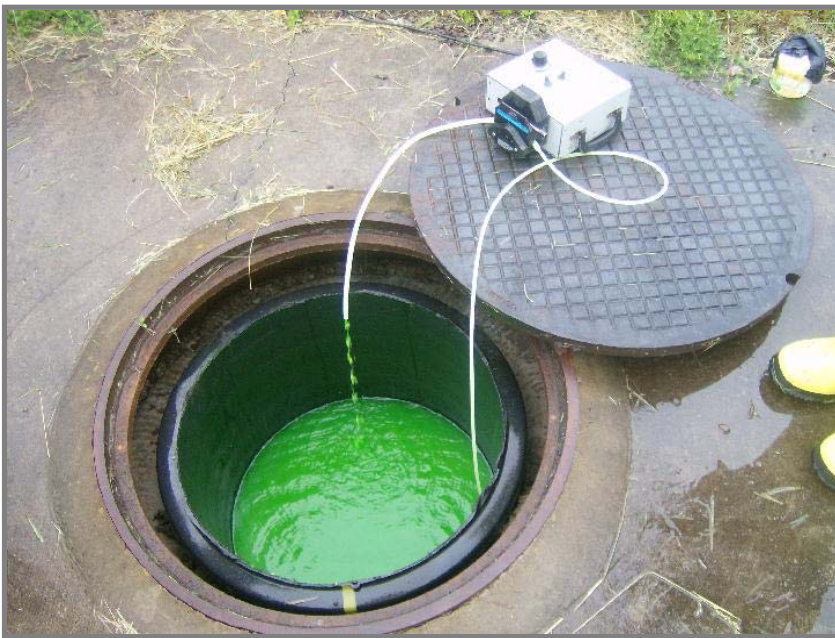
Manway riser and peristaltic pump
