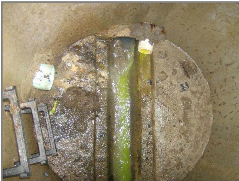
Green finally in the sewer. We had pumped some leachate into one of the leachate clean-out stickups behind the tank and the valve access manholes. About 1/2 hour later we saw the green dye.
