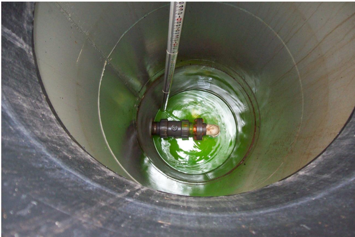
Photo 4: Inlet pipe manway and control valve.
