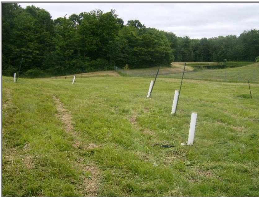
Groundwater and leachate cleanout stickups behind the tank.
