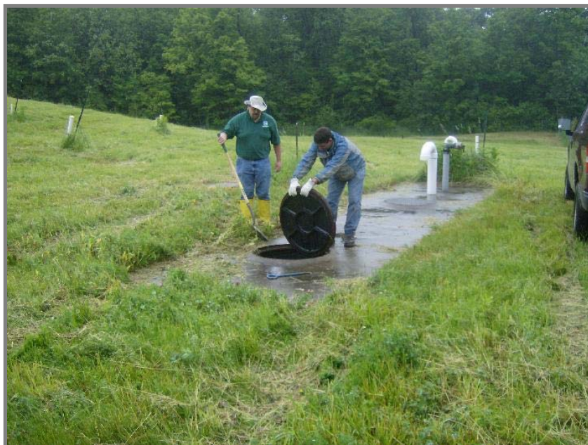
Jeremy and Payson are opening the manhole covers in the leachate tank area.
