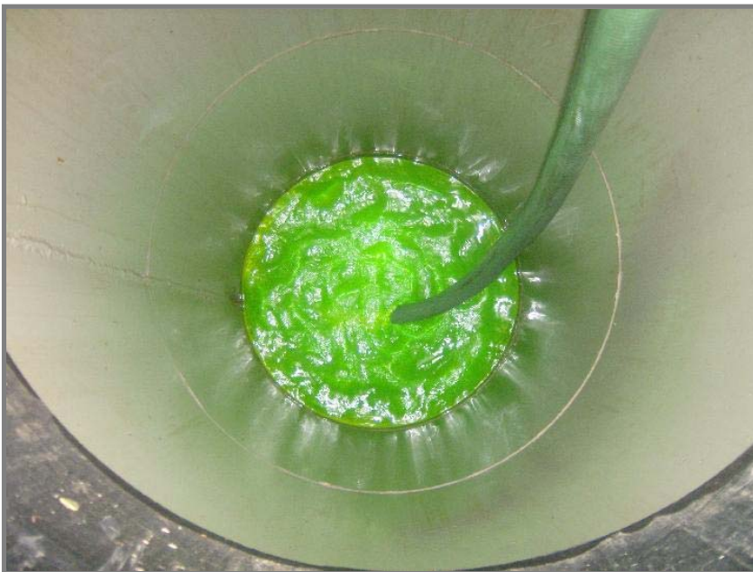
Looking into the manway riser almost pumped down makes for a surreal image.
