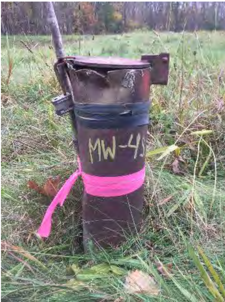
MW-4S with evidence of historic mower damage to protective casing
