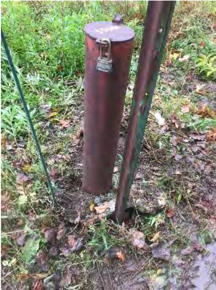
MW-1S – Concrete collar shows frost heaving
