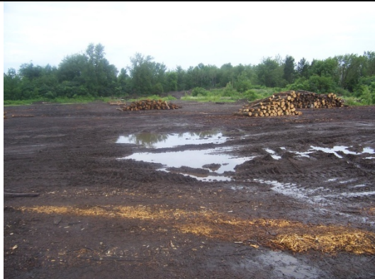
The stone cover is less than the shovel blade down the synthetic liner. The Capped area needs to be regraded.
