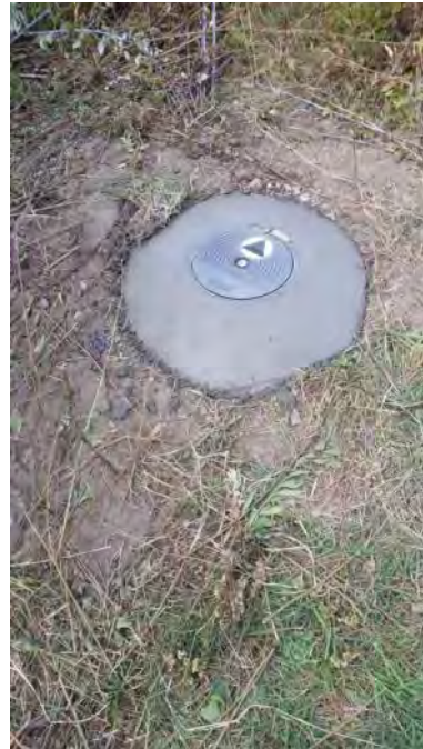
MW-4 new flush-mount and concrete pad
