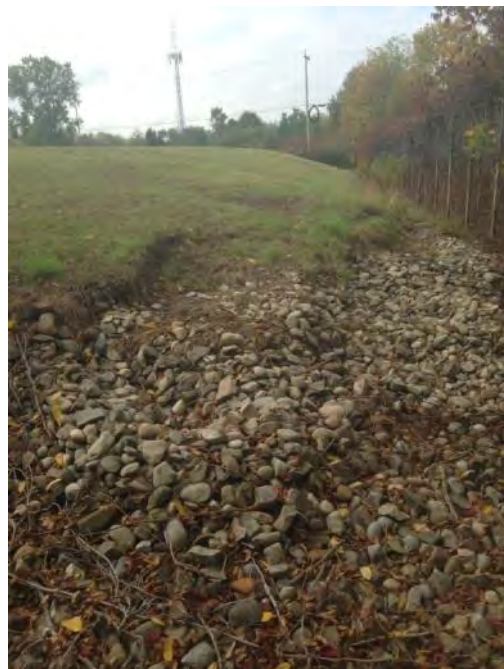
Northeast corner of landfill – facing west (10/1/14) Ruts visible from mower.
