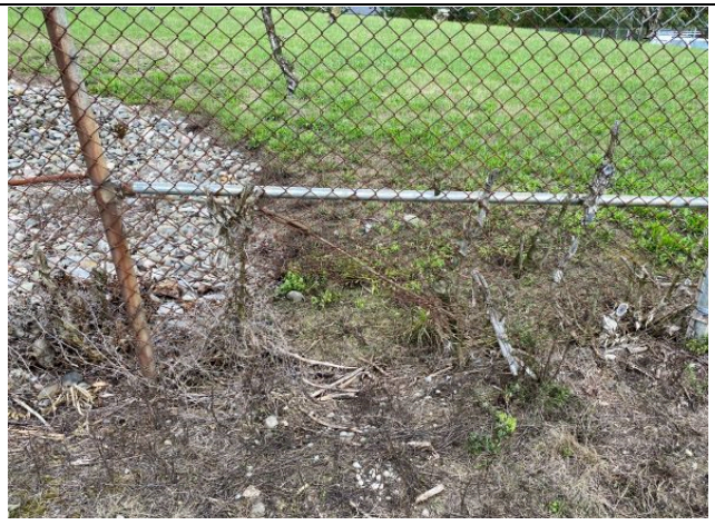
Photo 6: Photograph of the hole in the fencing located along the southern Site boundary.
