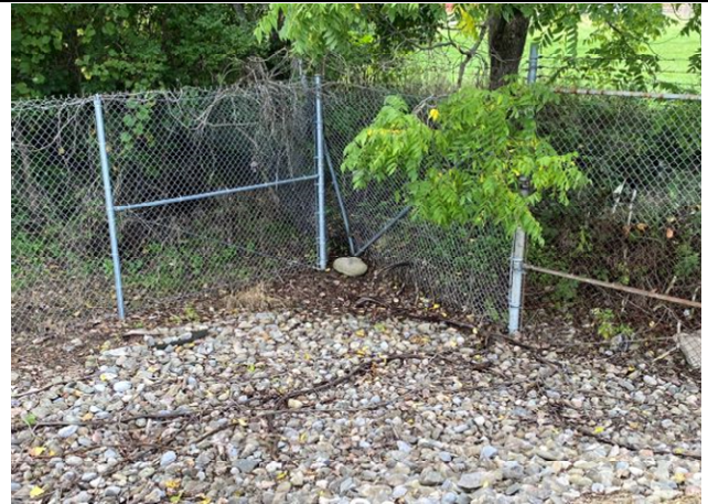
Photo 4: View of the damaged area of the site fencing located at the northeast corner.
