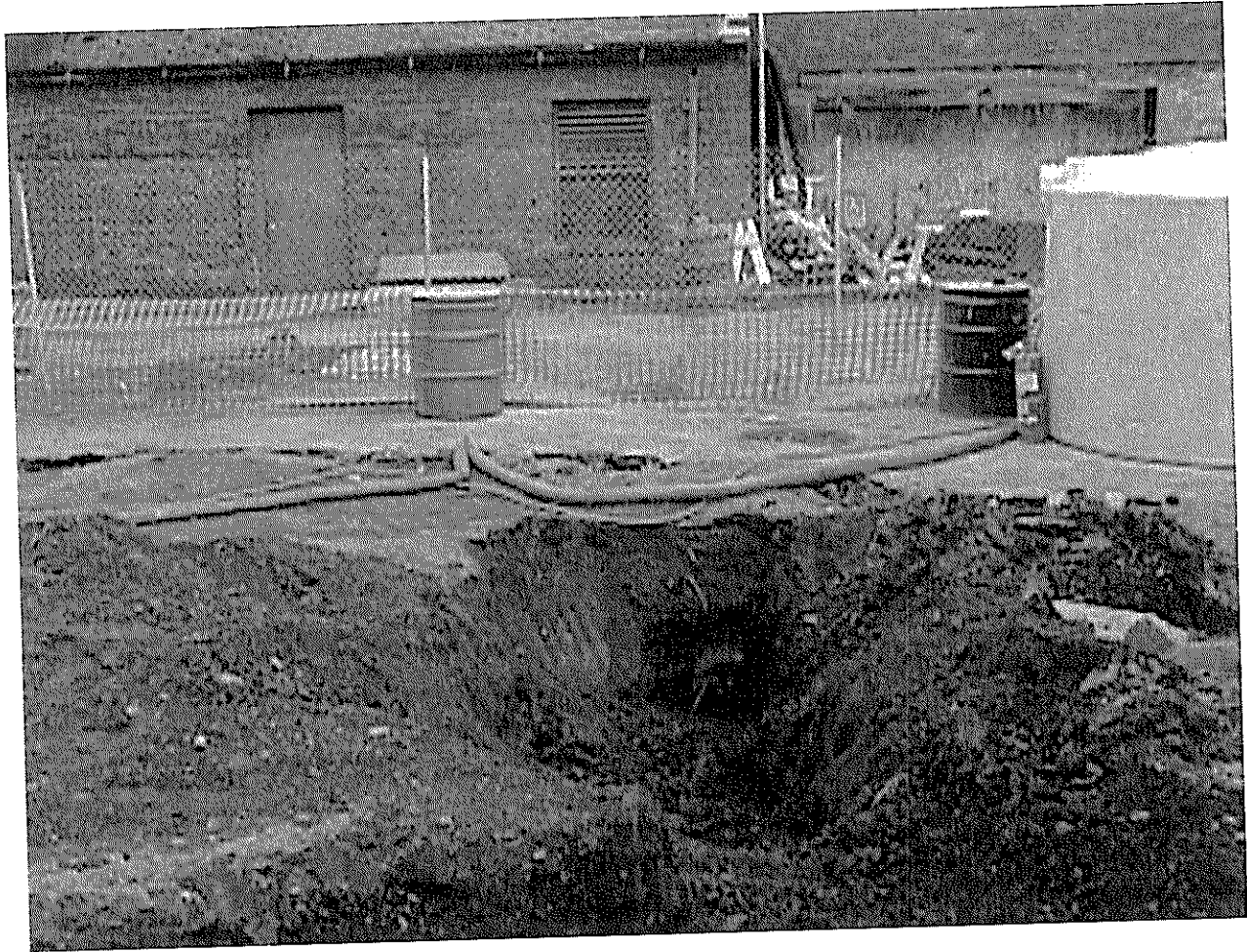
ITHACA COURT STREET FORMER MANUFACTURED GAS PLANT 2000 REMEDIATION PROJECT PHOTO NUMBER 13 FEBRUARY 2000
