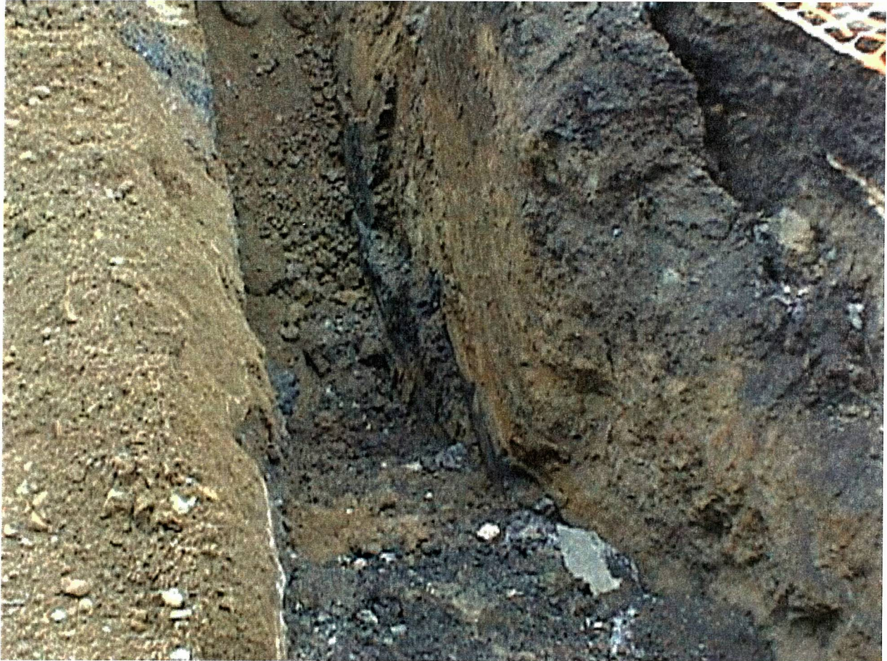
ITHACA COURT STREET FORMER MANUFACTURED GAS PLANT 2000 REMEDIATION PROJECT PHOTO NUMBER 15 FEBRUARY 2000
