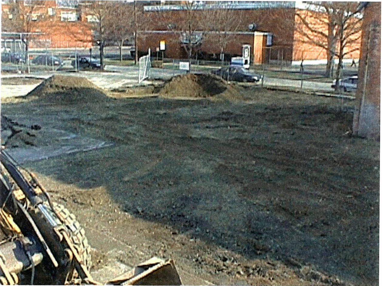
ITHACA COURT STREET FORMER MANUFACTURED GAS PLANT 2000 REMEDIATION PROJECT PHOTO NUMBER 17 MARCH 2000
