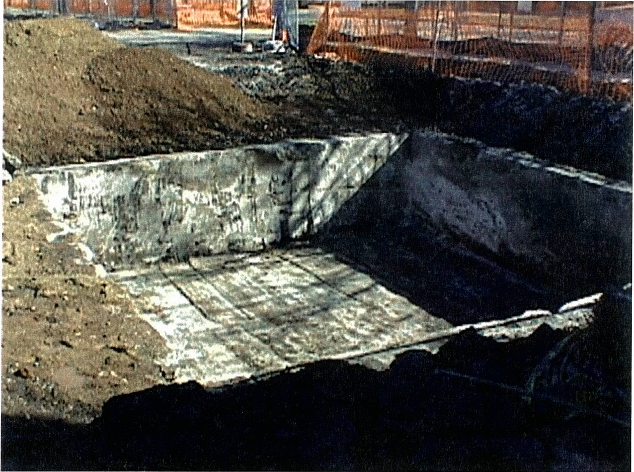
ITHACA COURT STREET FORMER MANUFACTURED GAS PLANT 2000 REMEDIATION PROJECT PHOTO NUMBER 10 FEBRUARY 2000
