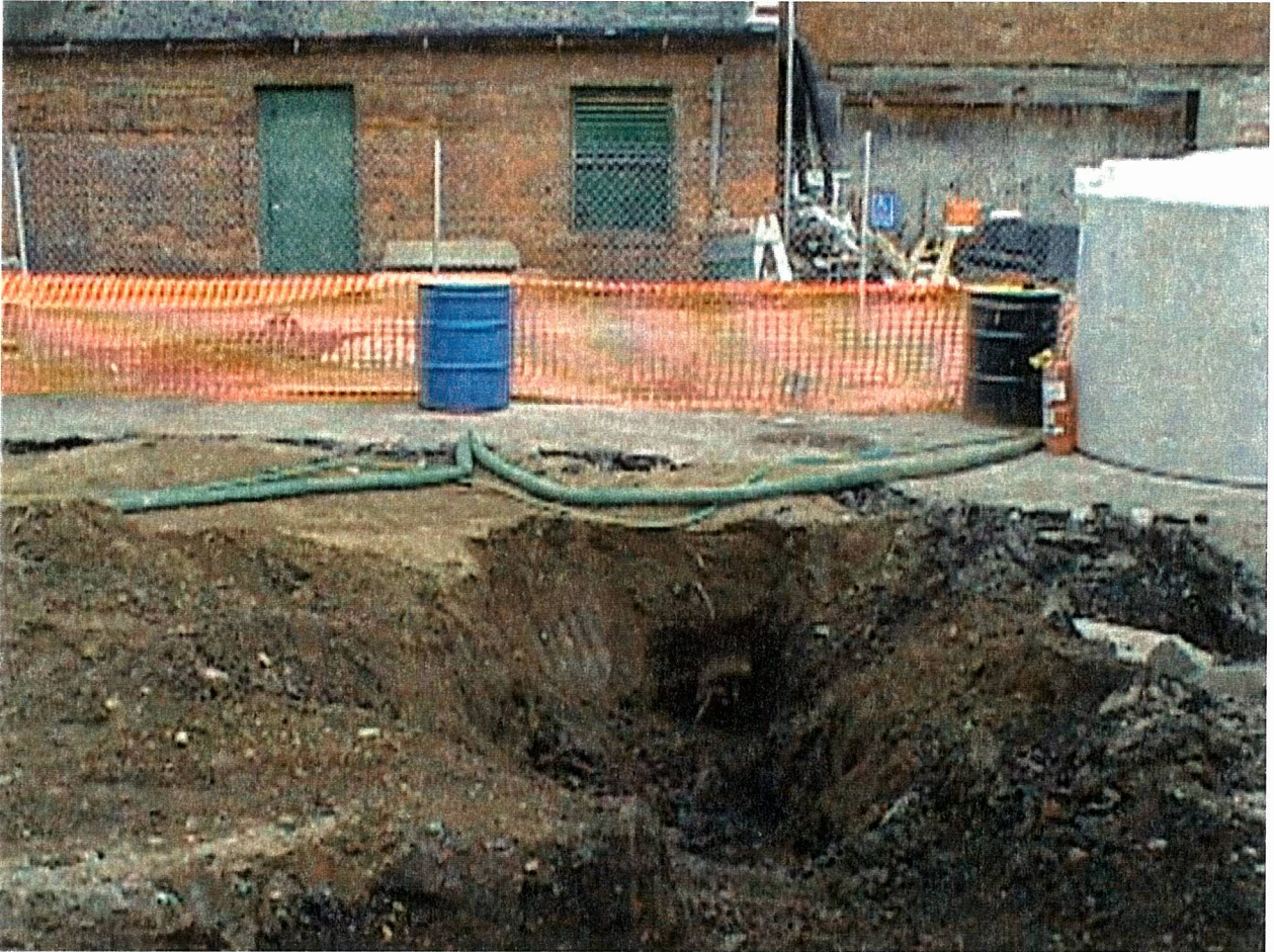
ITHACA COURT STREET FORMER MANUFACTURED GAS PLANT 2000 REMEDIATION PROJECT PHOTO NUMBER 13 FEBRUARY 2000
