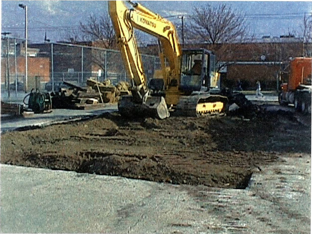
ITHACA COURT STREET FORMER MANUFACTURED GAS PLANT 2000 REMEDIATION PROJECT PHOTO NUMBER 16 MARCH 2000
