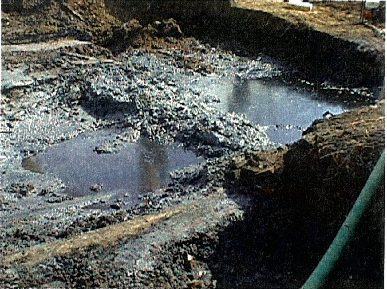
ITHACA COURT STREET FORMER MANUFACTURED GAS PLANT 2000 REMEDIATION PROJECT PHOTO NUMBER 12 FEBRUARY 2000
