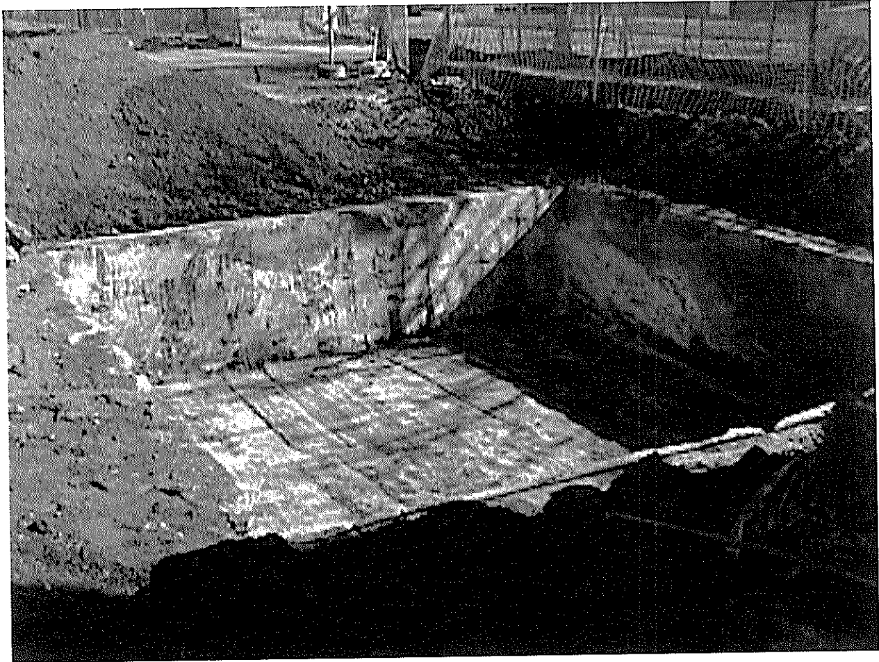
ITHACA COURT STREET FORMER MANUFACTURED GAS PLANT 2000 REMEDIATION PROJECT PHOTO NUMBER 10 FEBRUARY 2000
