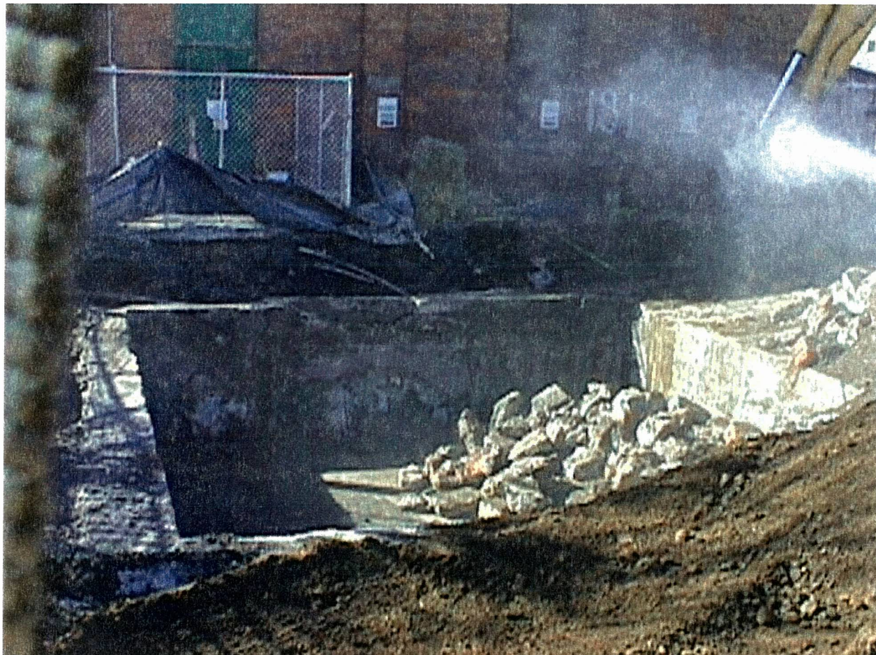
ITHACA COURT STREET FORMER MANUFACTURED GAS PLANT 2000 REMEDIATION PROJECT PHOTO NUMBER 11 FEBRUARY 2000
