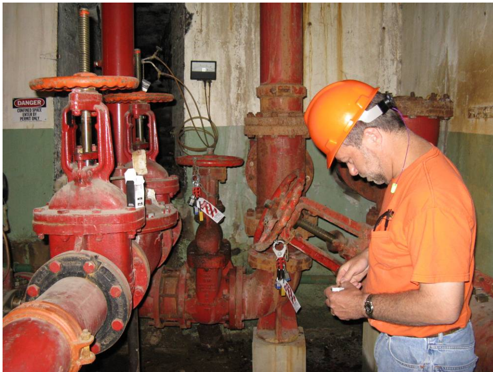
Suction Pump Lock-Out Tag-Out Prior to Confined Space Entry
