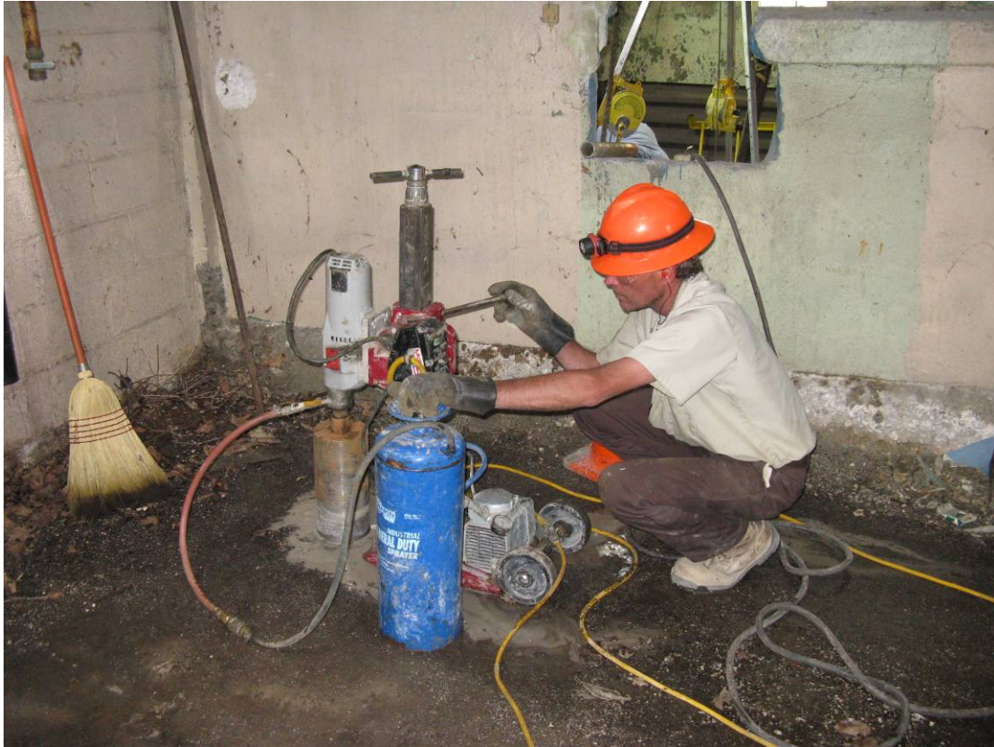
Coring on top of fire water reservoir at Monitoring Point 2 along west wall
