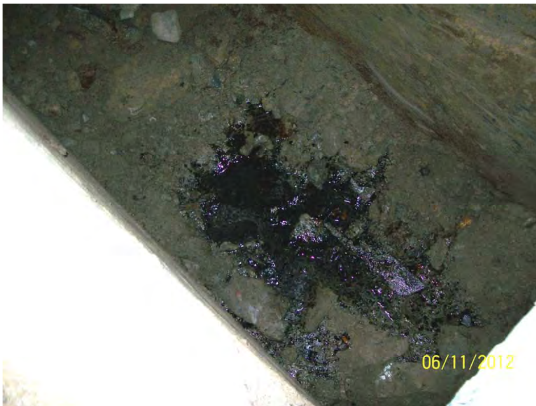
Photo 18: Petroleum Product in the Conveyor Trench adjacent to column – Building 4
