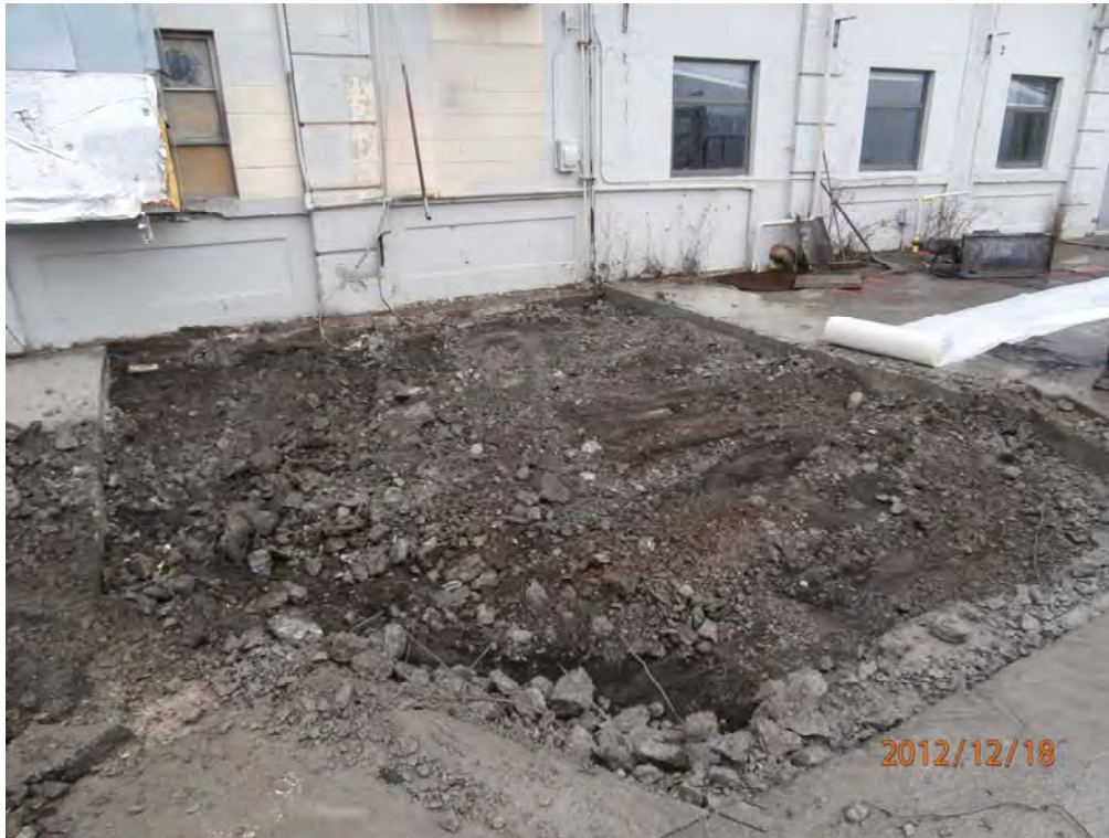
Photo 33: Exposed Soil Surface at the Base of the Concrete
