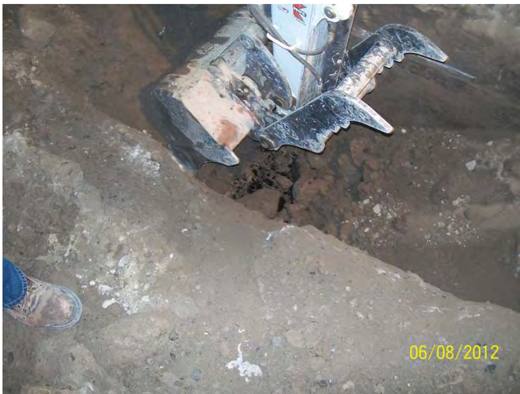
Photo 11: Discovery of Petroleum Product in the Conveyor Trench at Column – Building 3
