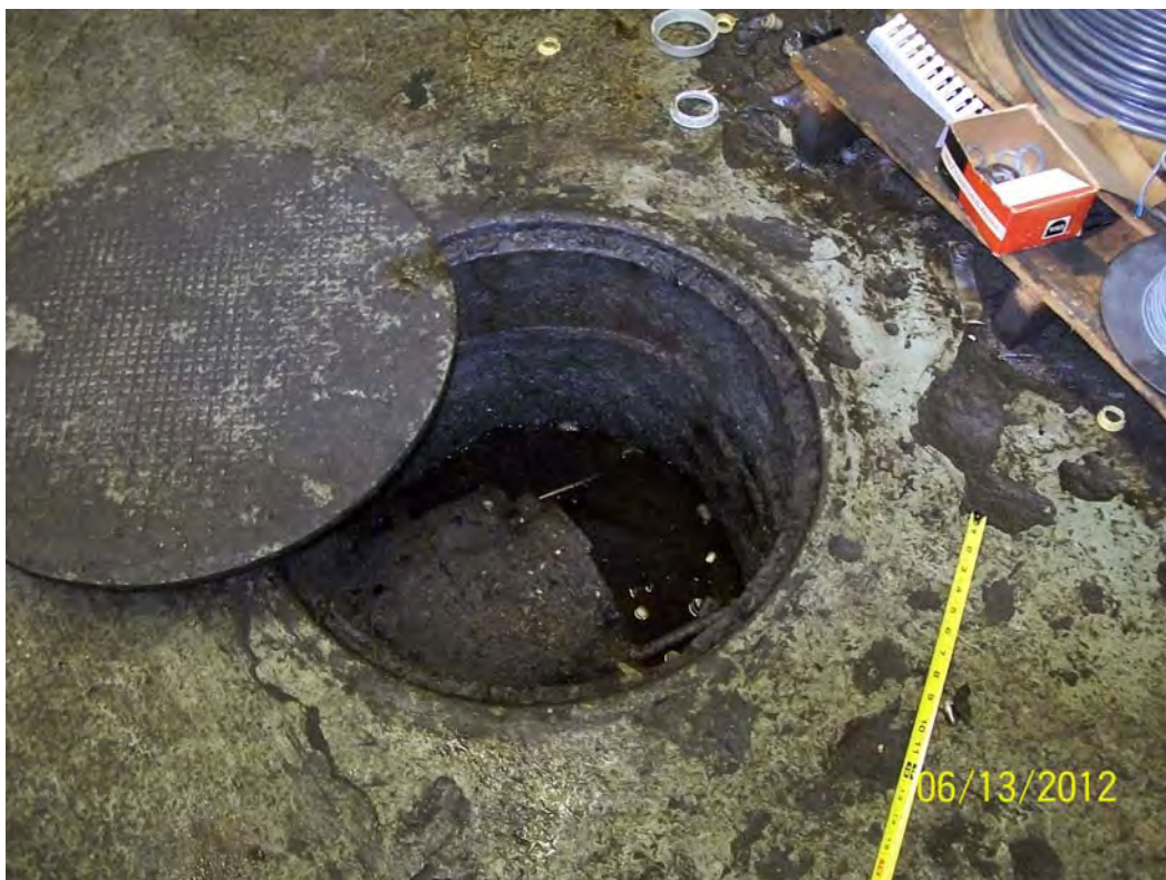
Photo 22: Manhole with Containing Petroleum Product – Building 2
