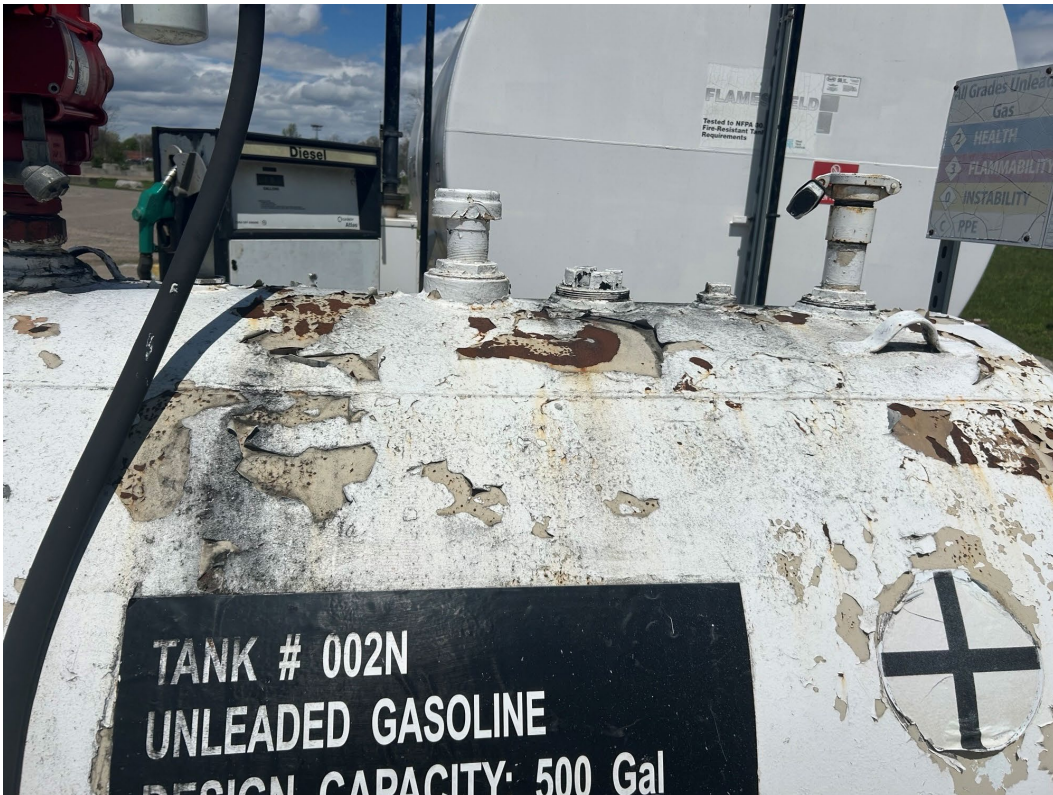
Tank 002N – Tank exterior needs repainting (loose & peeling paint)
