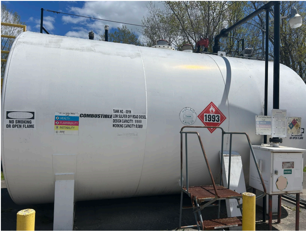
Tank 001N 0 9,988 gallon off road diesel tank
