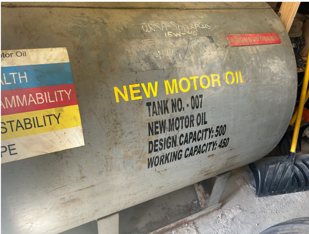
Tank 007 – 500 gallon mew motor oil tank
