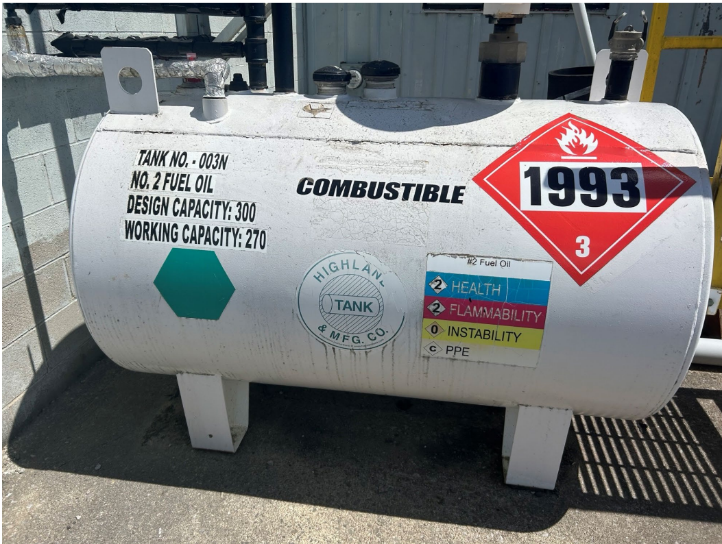
Tank 003N – 300 gallon #2 FO Tank.
