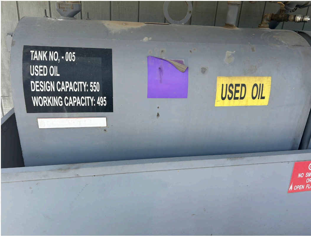
Tank 005 – 550 gallon Used Oil tank
