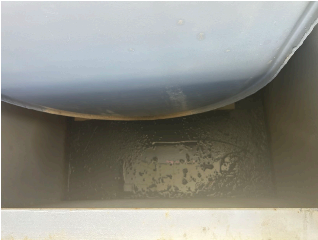
Tank 005 Secondary Containment (dike) – accumulation of liquids & debris noted
