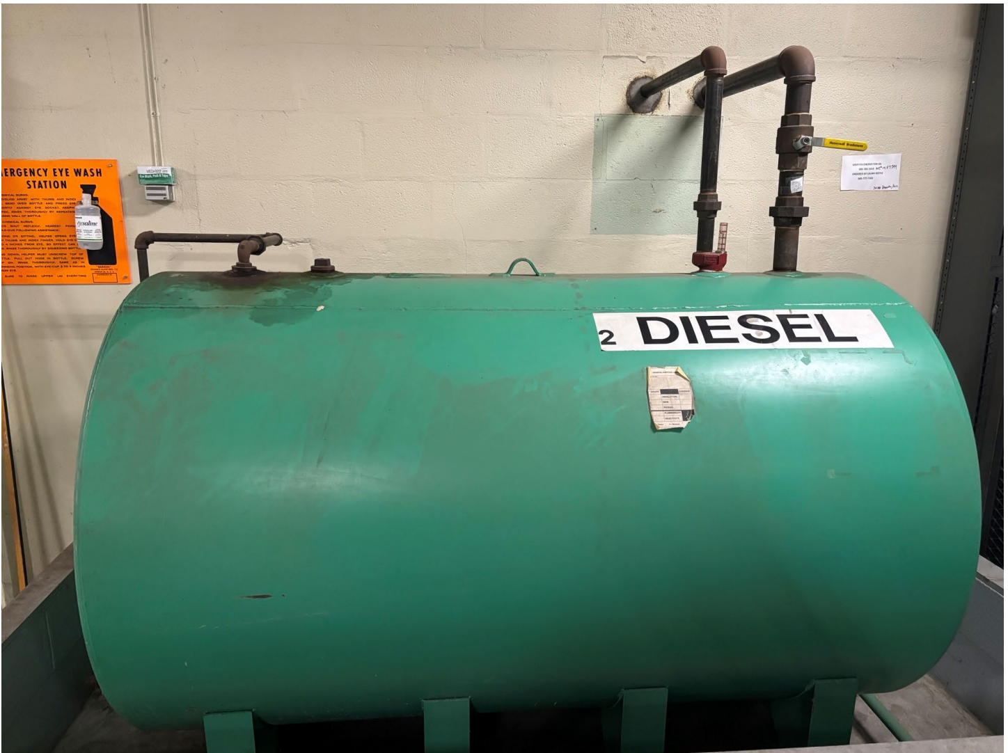
500 gallon AST storing diesel fuel for emergency power generator located in the basement of the building.
