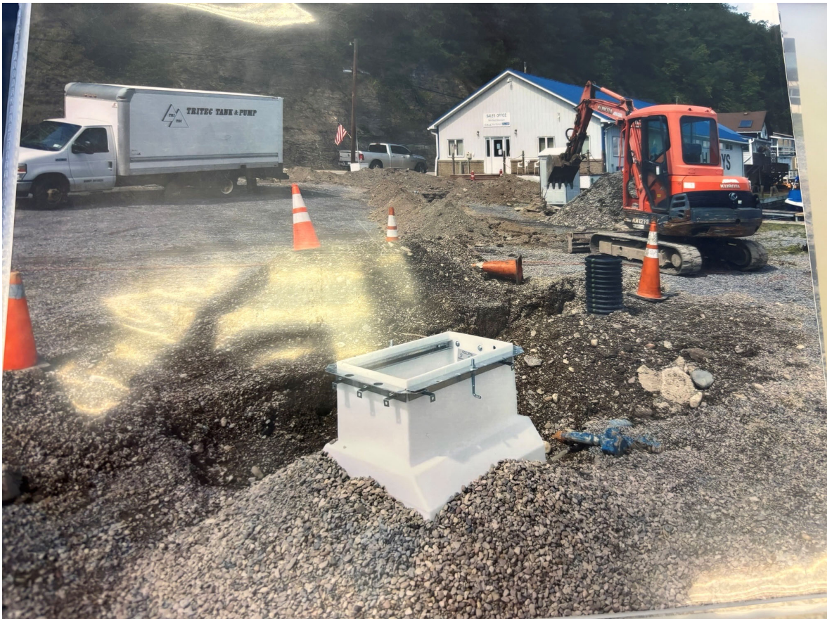
Photo of new UDC and conduit for piping (taken Sept 2023)
