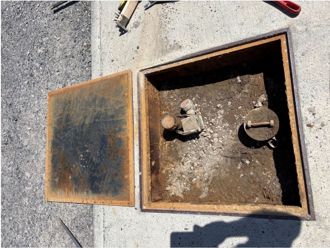
Tank interstitial port (left)
