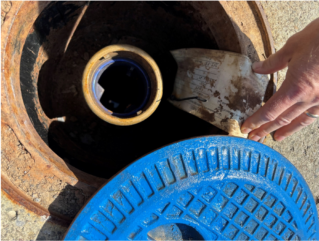
Fill port color coding, tank ID tag, spill bucket and drop tube with ASO.
