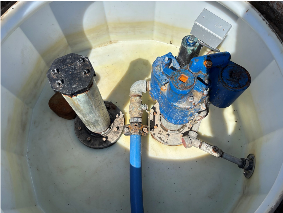
Tank top sump with submersible pump for pressurized dispensing, new double walled flexible piping and Automatic Line Leak Detector (ALLD)
