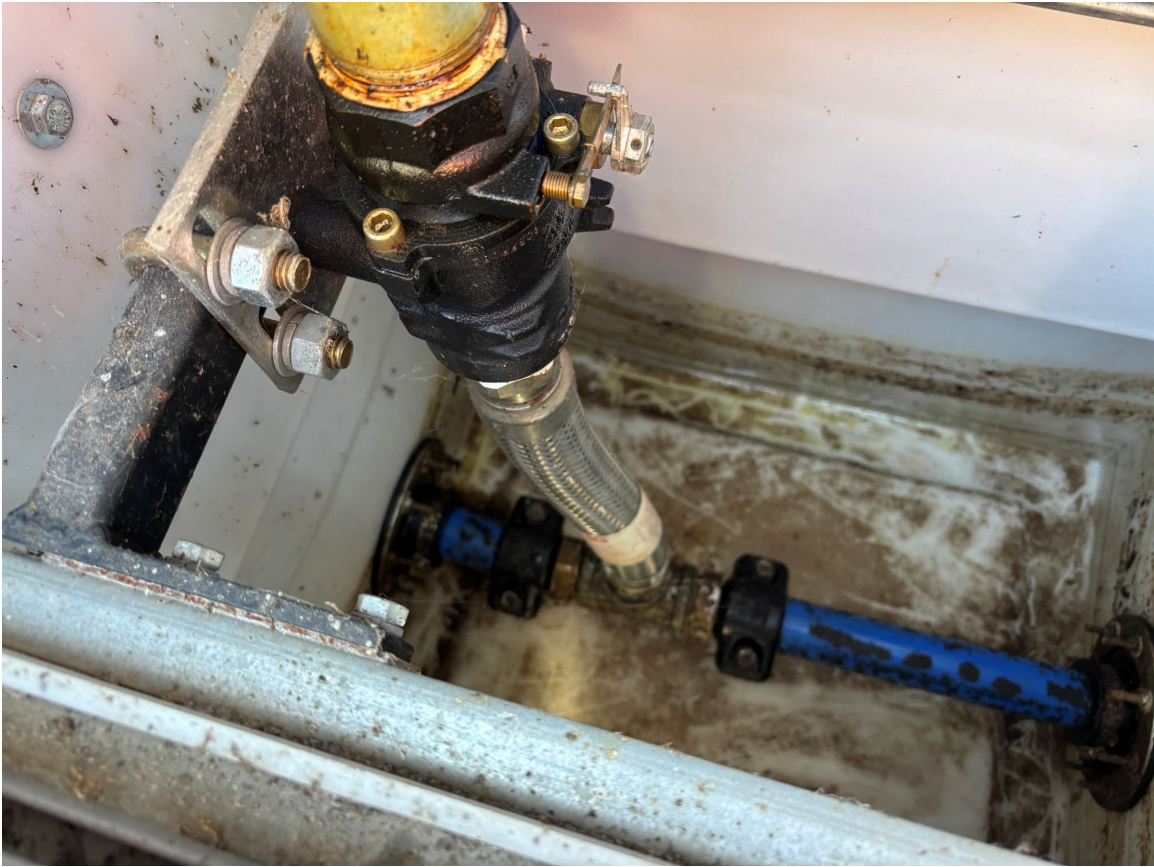
Under Dispenser Containment (UDC) sump and shear valve
