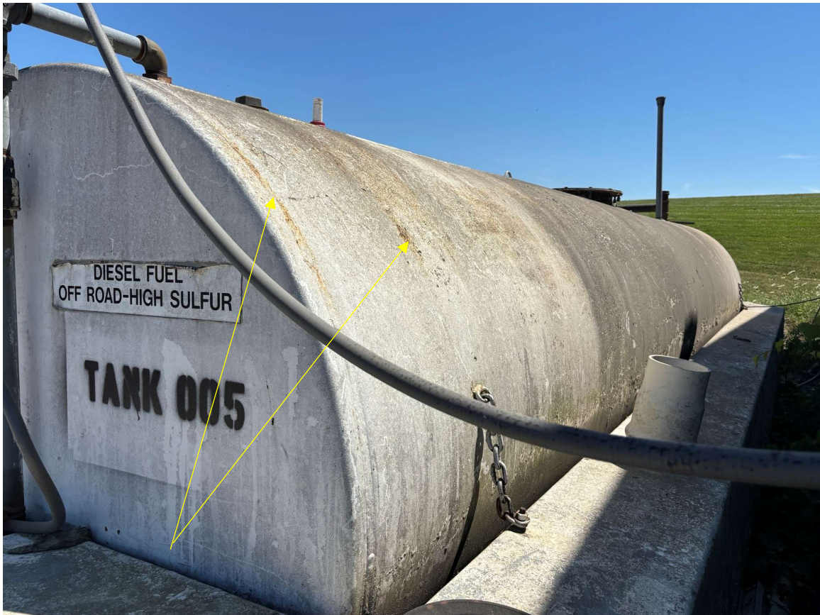
Tank 005 – Areas of corrosion observed.
