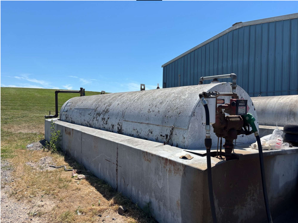
Tank 006 – 4,000 gallon diesel tank. Areas of loose / peeling paint observed.
