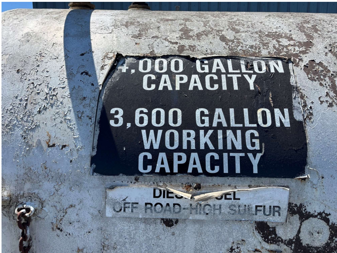
Tank 006 labeling. Note: Tank # is on end of tank.
