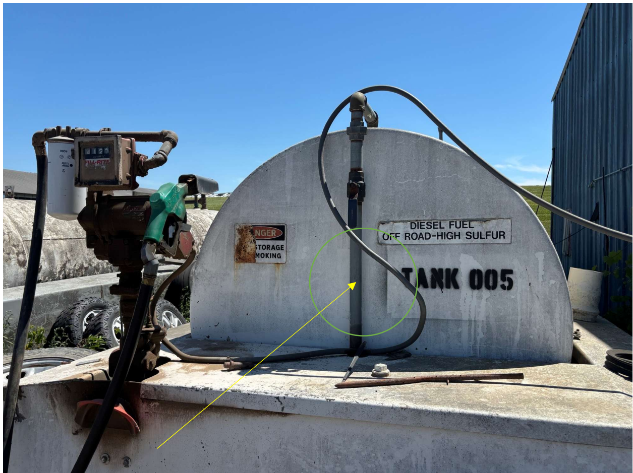
No solenoid (anti-siphon) valve immediately downgradient of the operational valve.
