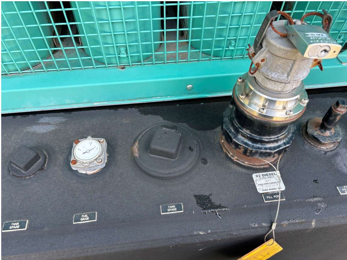
Tank #5 fill port and product level gauge (typ)
