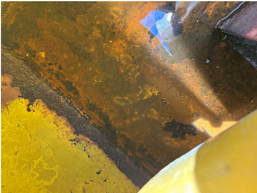
Tank #9 secondary containment (steel dike). Violation for accumulation of liquid / debris and corrosion. Recommended repainting after draining liquids and removing debris.
