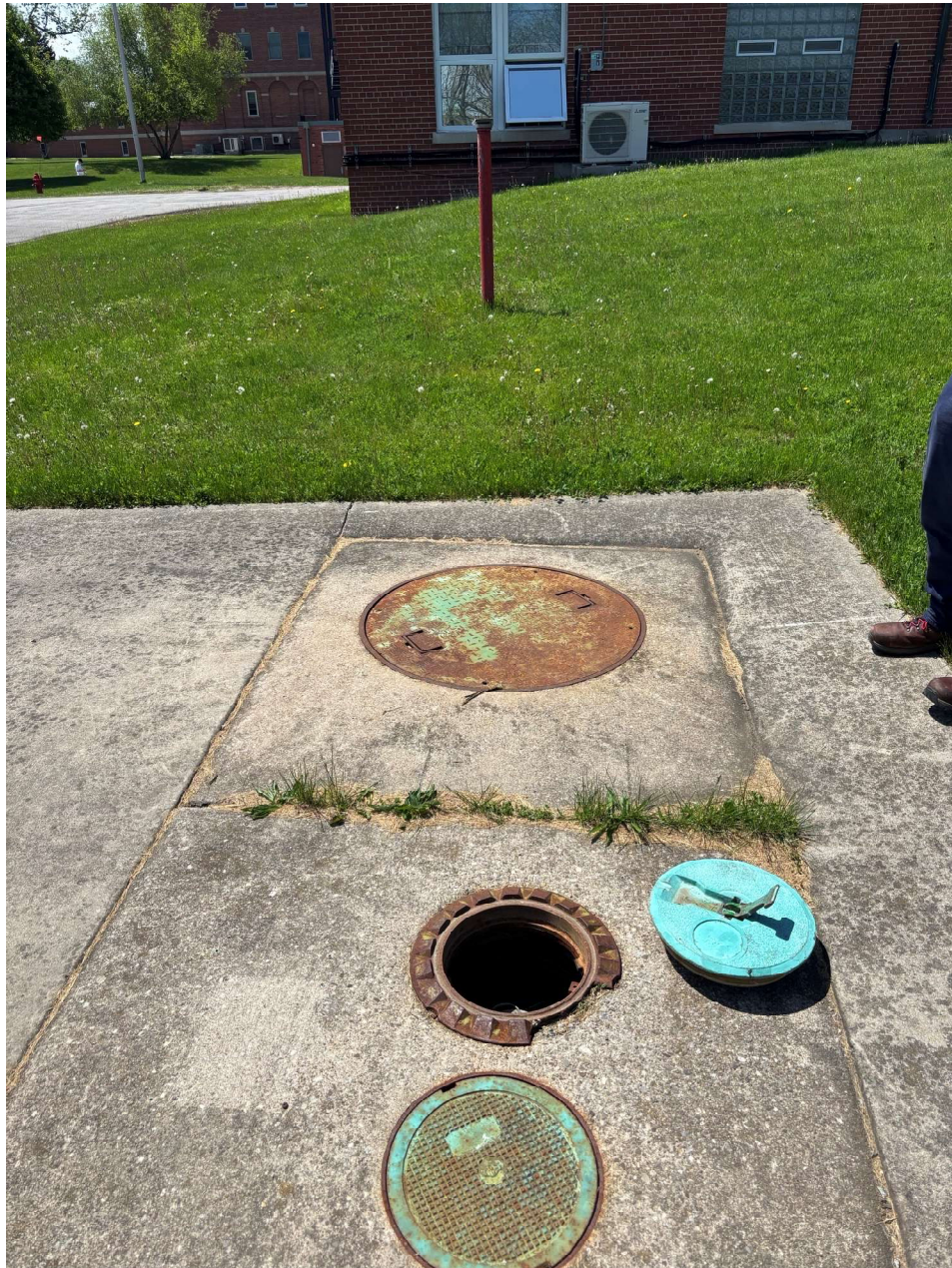
Tank #2 – 20,000 gallon single walled FRP tank storing #2 FO
