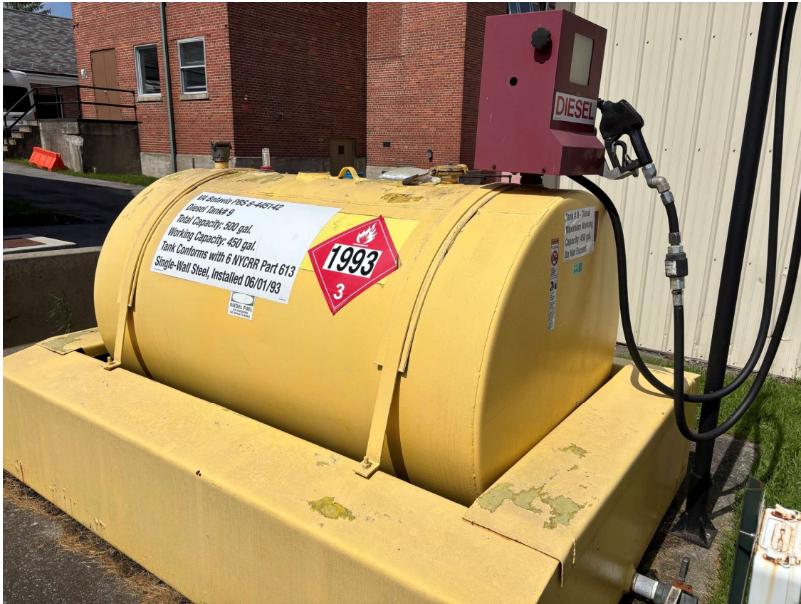
Tank #9 – 500 gallon diesel tank installed in 2006. Small areas of corrosion starting to develop. Recommended removing tank from dike (when empty) to properly clean, inspect and repaint entire tank exterior. If corrosion AND pitting of the steel on bottom of tank is observed, the tank should be permanently closed and replaced.
