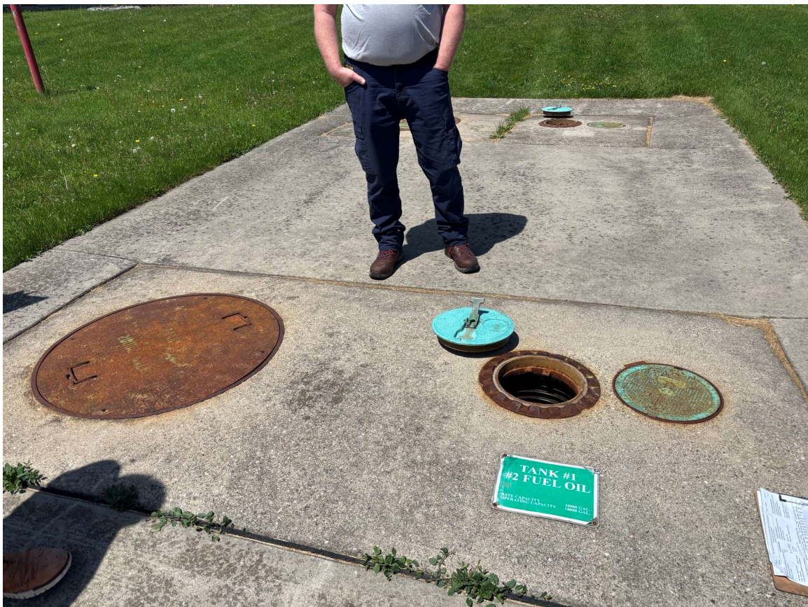
Tank #1 – 20,000 gallon single walled FRP tank storing #2 FO
