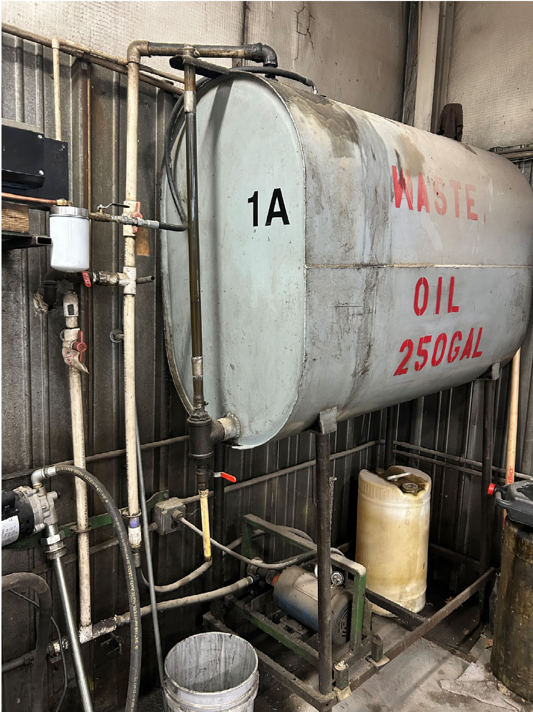
Tank 1A – 275 Gallon Used Oil AST (working capacity 250 gallon)
