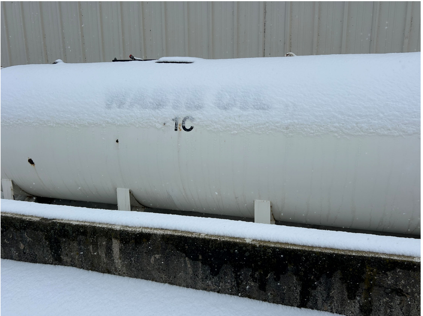
Tank 1C – 1,000 gallon used oil tank manifolded to tank 1A. Areas of corrosion need to be sanded down to bare steel and recoated. Tank labeling missing design and working capacities.
