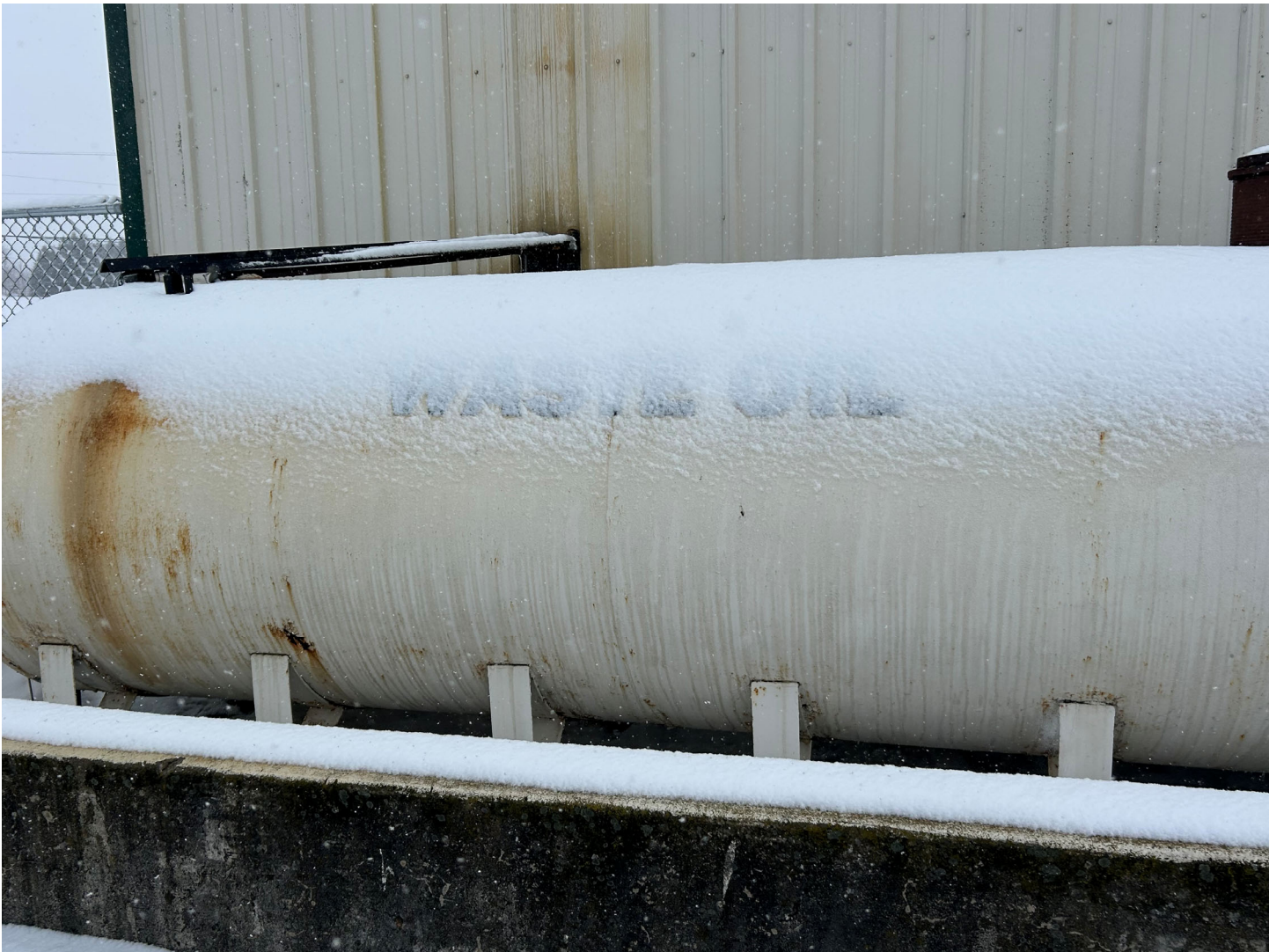
Tank 1B – Side view showing areas of corrosion
