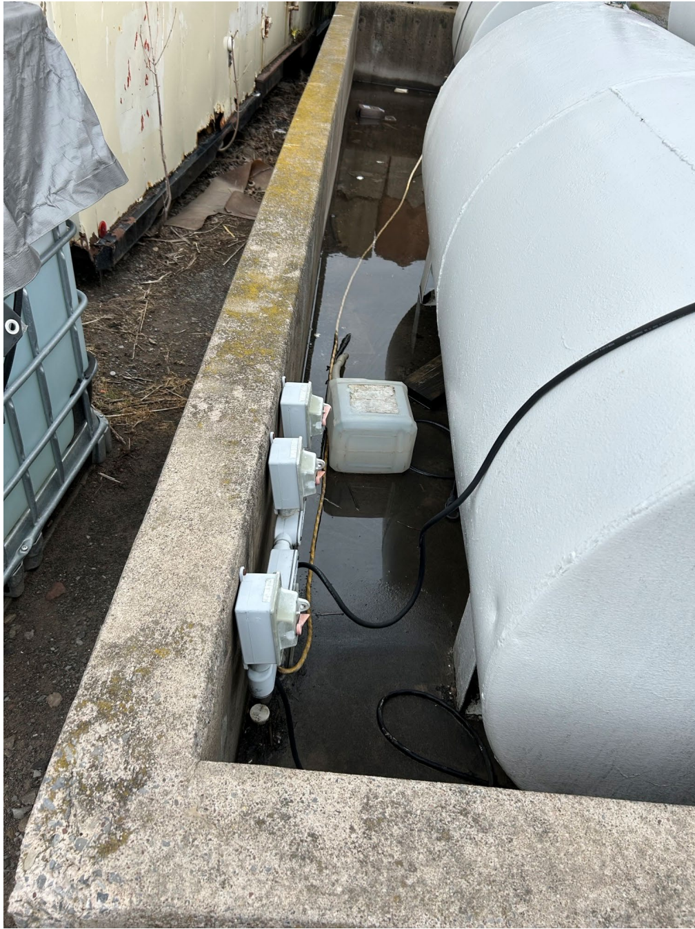
Accumulation of snow / ice melt in secondary containment (no sheen observed) – needs to be pumped empty.
