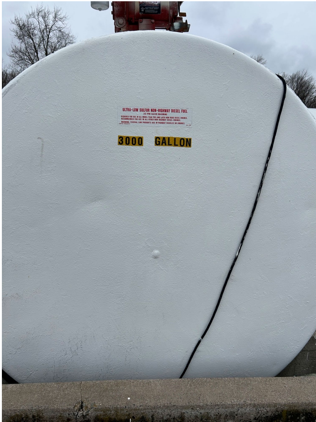
3000 gallon diesel tank – Need to be labeled with the tank ID # (30D), and working capacity (2700 gallons)
