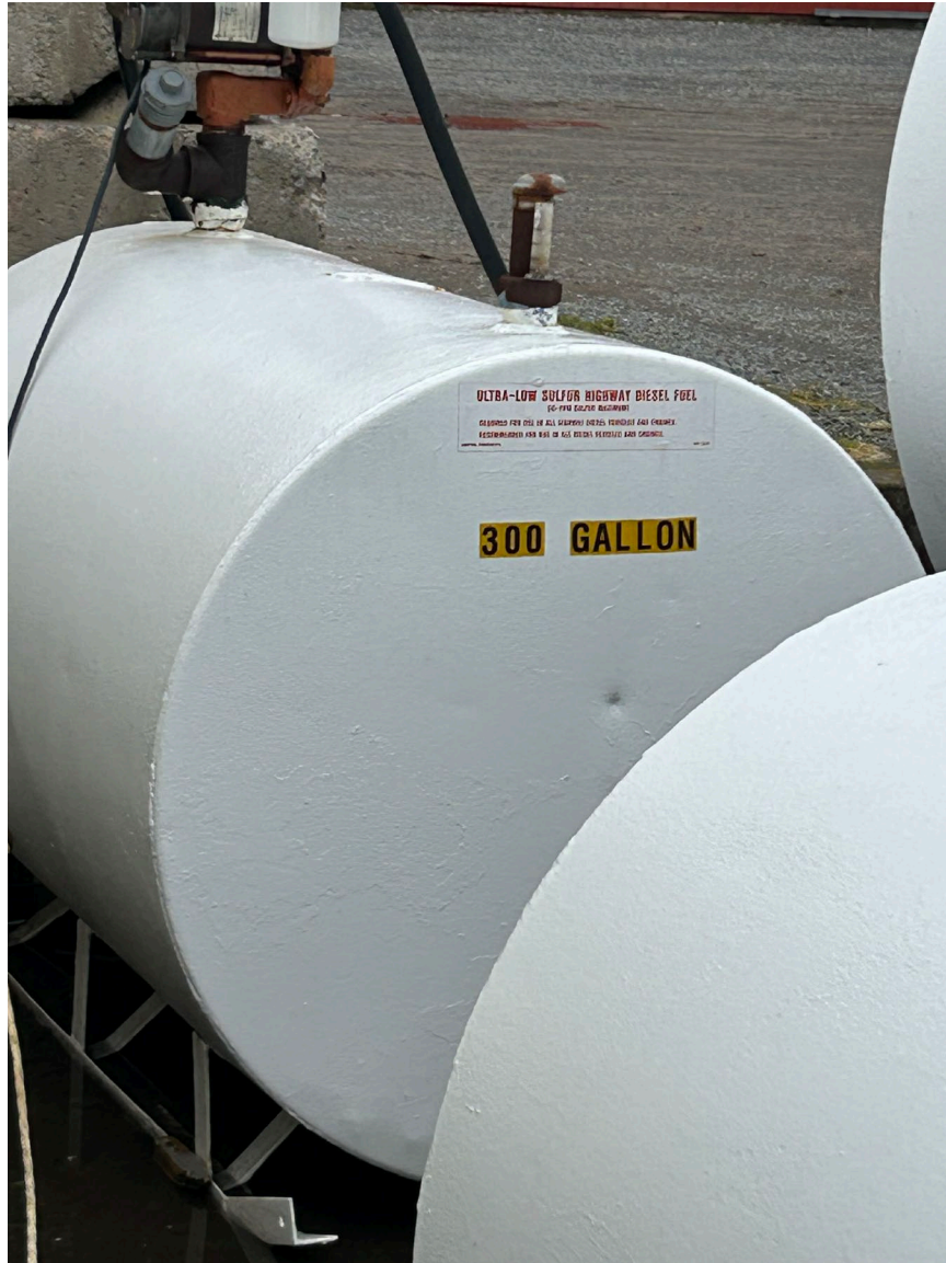
300 gallon diesel tank – Need to be labeled with the tank ID # (3D), and working capacity (270 gallons)
