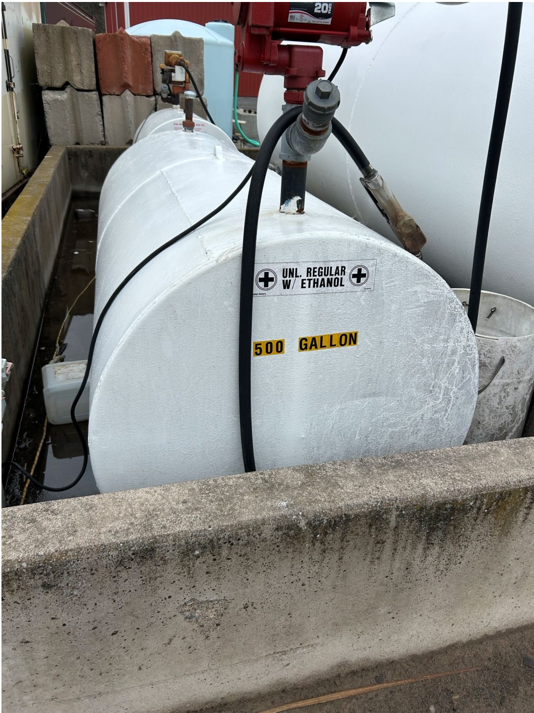
500 gallon gasoline tank – Needs to be labeled with the tank ID # (5G, and working capacity (450 gallons)
