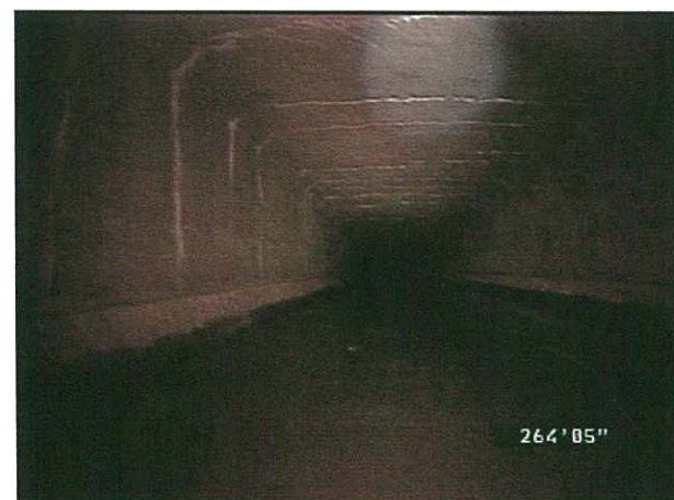
IMAGE: 7a, TAPE #: 01, 00:00:00 264.4FT, Multiple Cracks, from 08 to 04 o'clock
