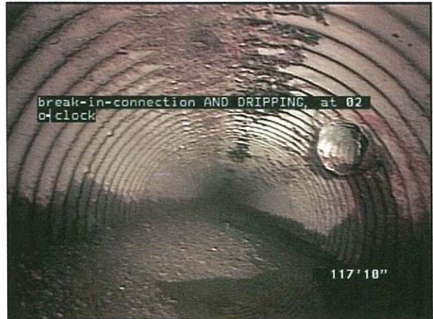
IMAGE: 28a, TAPE #: 01, 00:00:00 117.8FT, break-in-connection AND DRIPPING, at 02 o'clock
