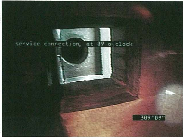
IMAGE: 8a, TAPE #: 01, 00:00:00 309.75FT, service connection, at 09 o'clock
