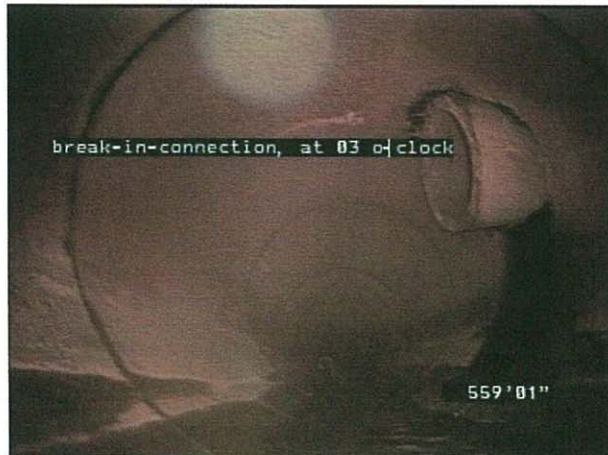
IMAGE: 15a, TAPE #: 01, 00:00:00 559.1FT, break-in-connection, at 03 o'clock
