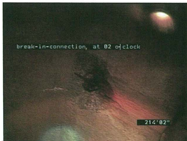
IMAGE: 6a, TAPE #: 01, 00:00:00 214.2FT, break-in-connection, at 02 o'clock
