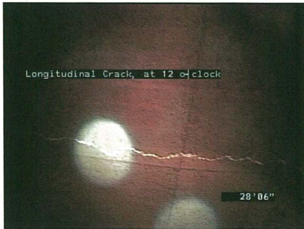
IMAGE: 3a, TAPE #: 01, 00:00:00 28.5FT, Longitudinal Crack, at 12 o'clock
