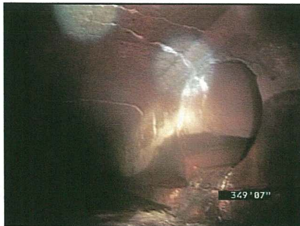
IMAGE: 9b, TAPE #: 01, 00:00:00 349.5FT, service connection, at 03 o'clock
