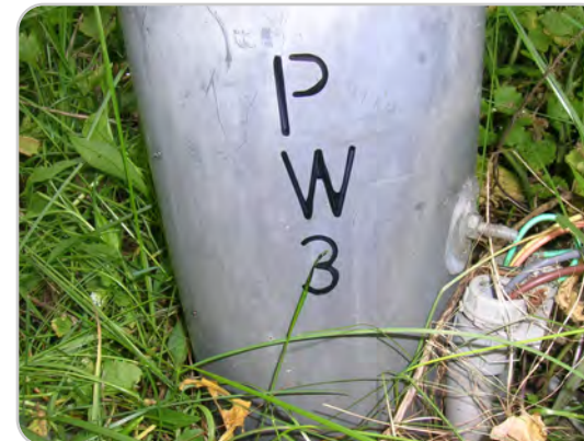
Shot 11: Pumping Well PW-3 Date: May 24, 2012
