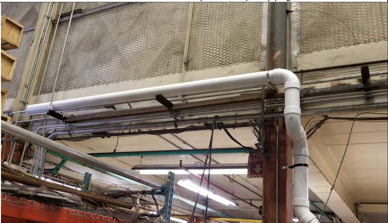
Photo 8 – SSD system piping in the PCore Building.
