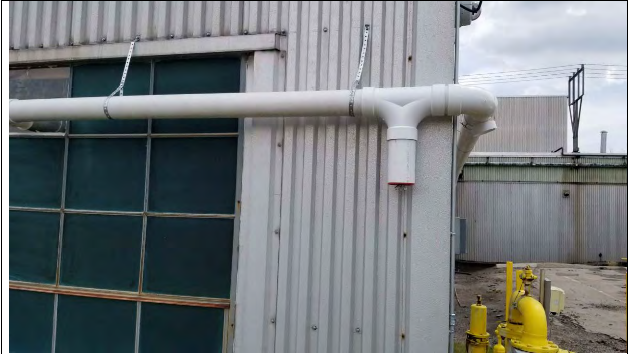
Photo 13 – Tee in PCore building SSD system for draining water from the piping.
