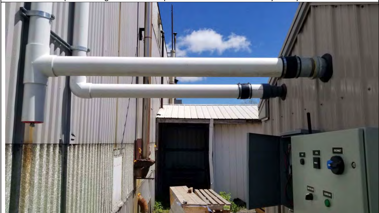
Photo 10 – SSD system piping connecting from the PCore Building to the SSD system sheds.
