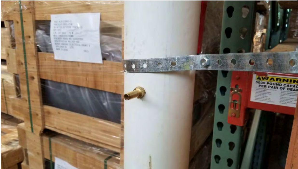
Photo 5 – Typical sampling port at an SSD system extraction point.
