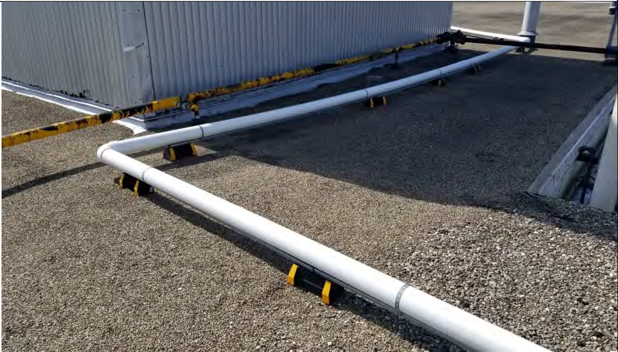
Photo 6 – SSD system piping on the roof of the PCore Building.
