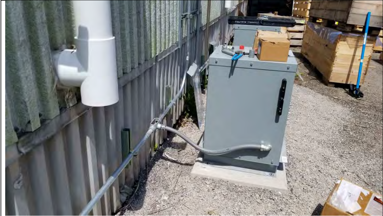
Photo 15 – PCore Building SSD system transformer.
