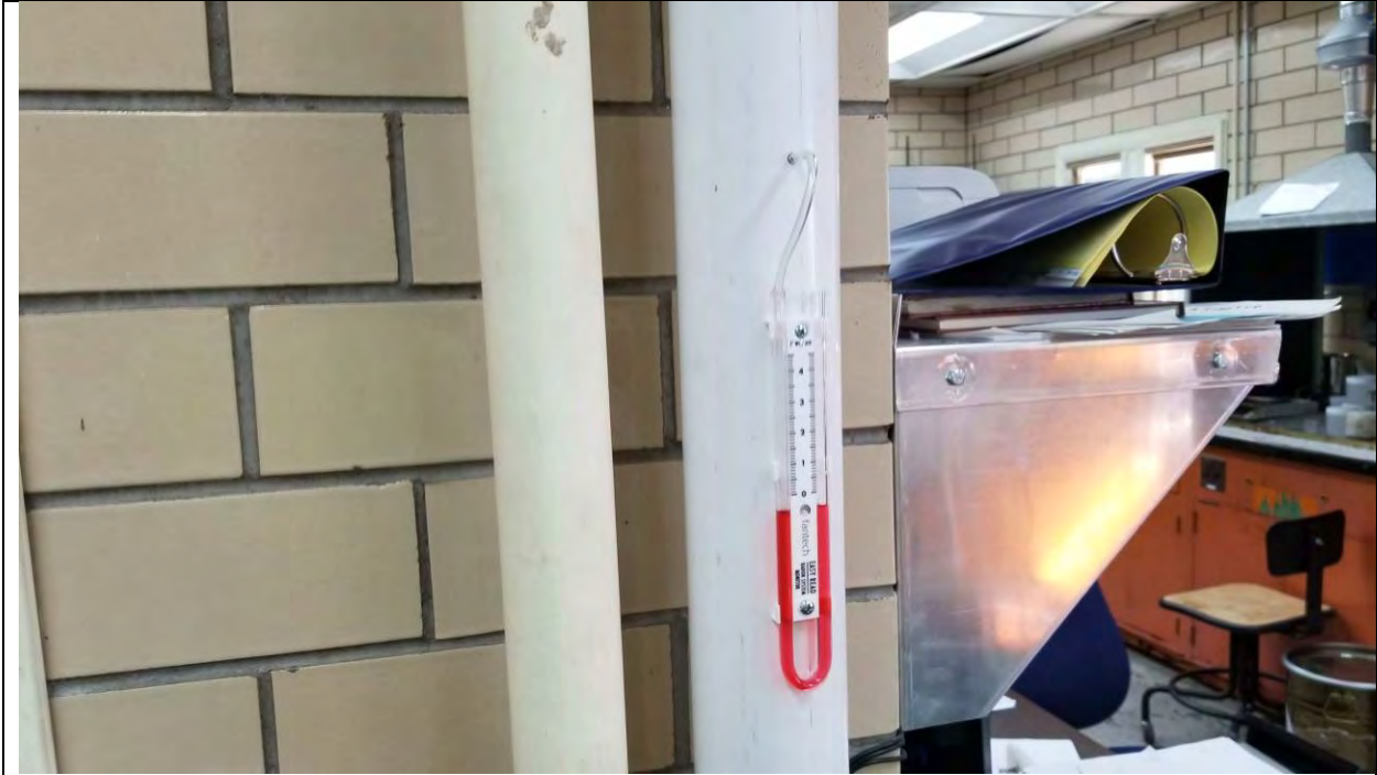
Photo 7 – A manometer tube on the PCore Laboratory extraction point piping.
