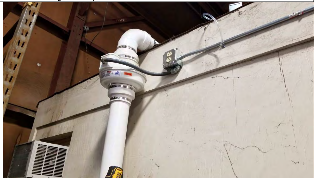
Photo 12 – Radon-style SSD system fan in Building B31.
