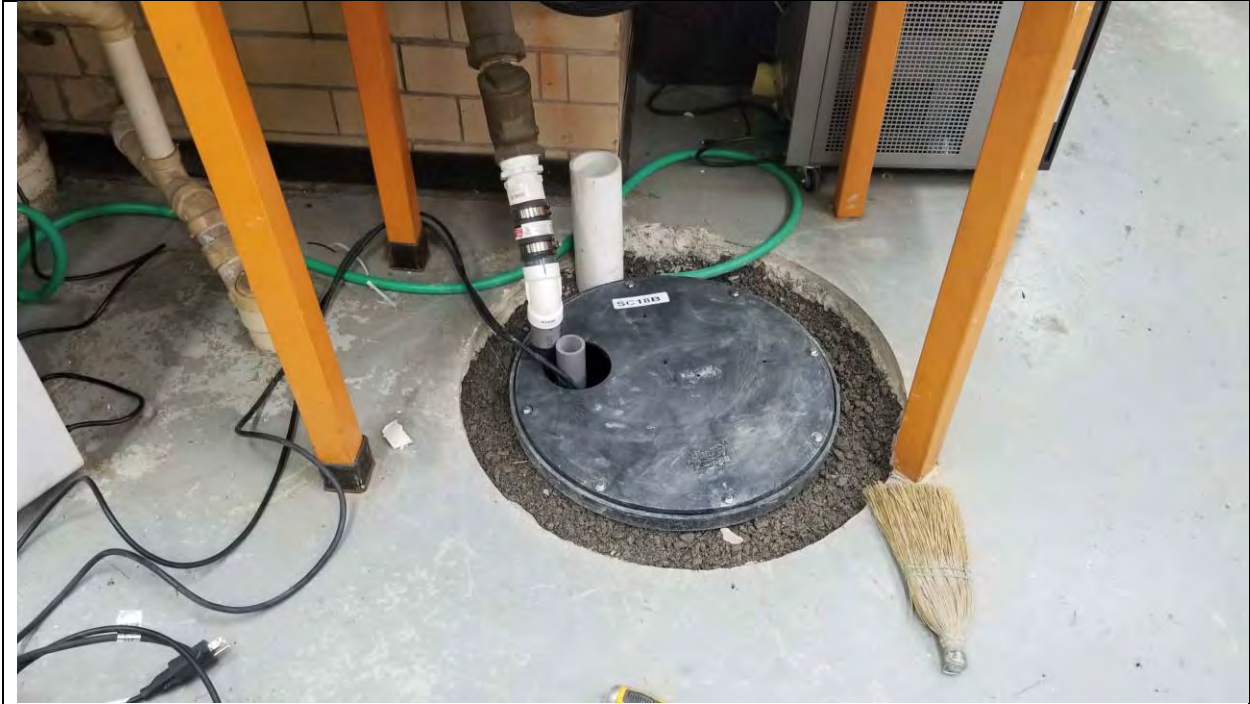
Photo 9 – A sump containing the extraction point for the PCore Laboratory SSD system.
