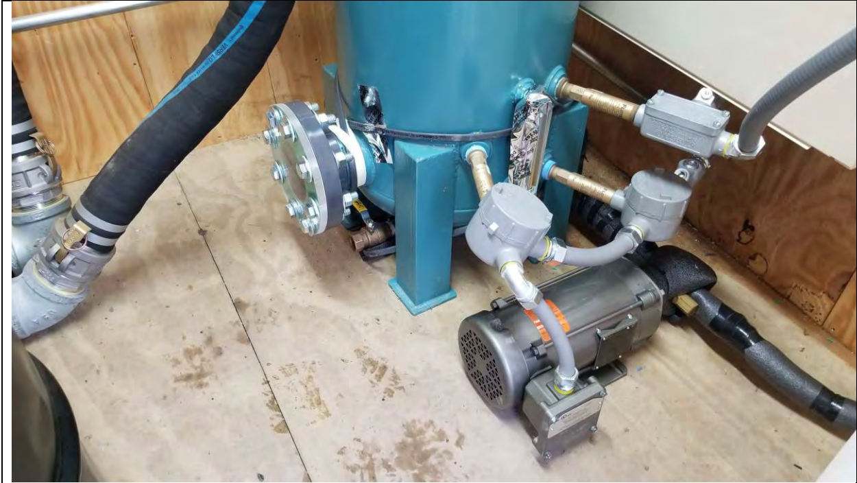
Photo 1 – SSD system transfer pump and knockout tank.
