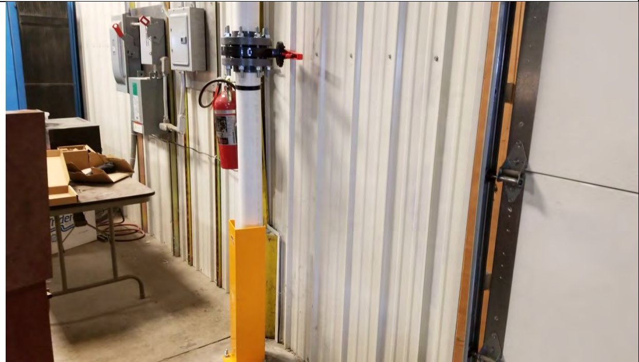
Photo 3 – SSD system extraction point with butterfly valve and pipe guard in Building B35.
