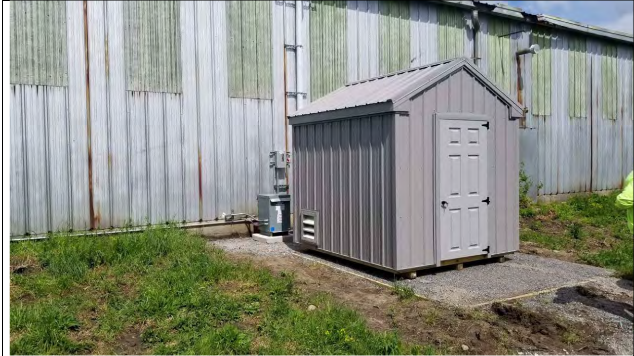
Photo 11 – Building B35 SSD system shed.
