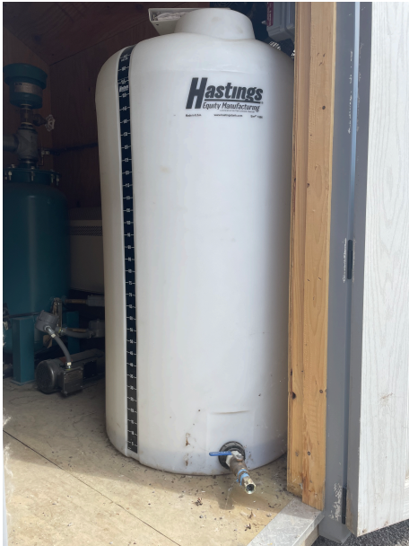
PCORE-01 KO storage tank upon arrival.
