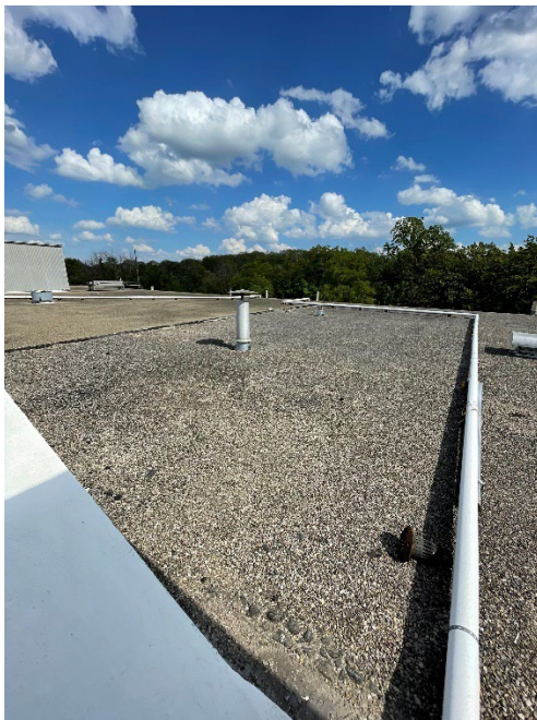
Piping on roof of PCORE building.
