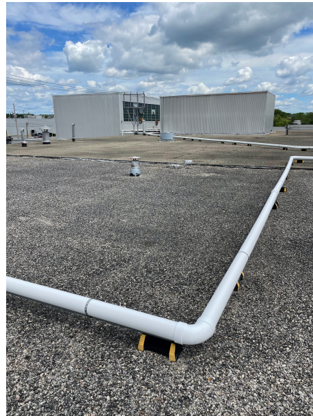
Piping on roof of PCORE building.
