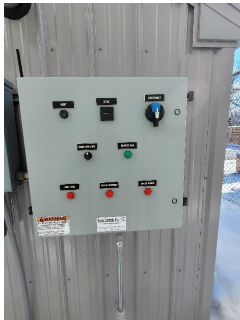
Motor Overtemp alarm activated when restarting
