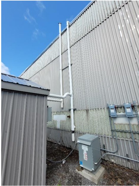
Vertical piping behind PCORE-01.
