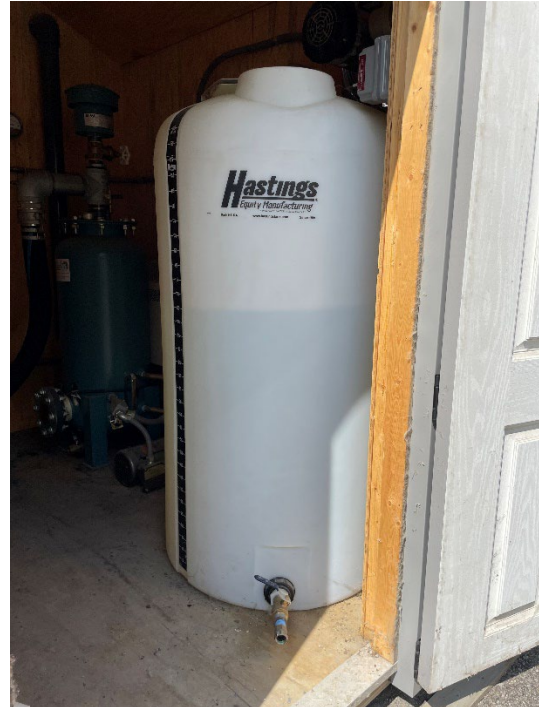
Knock out tank in right shed (SSDS-2)
