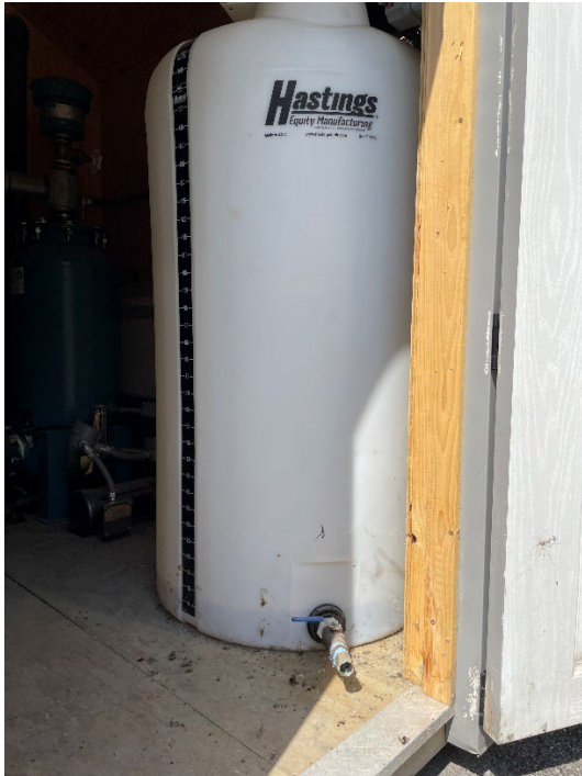
Knock out tank in left shed (SSDS-1)
