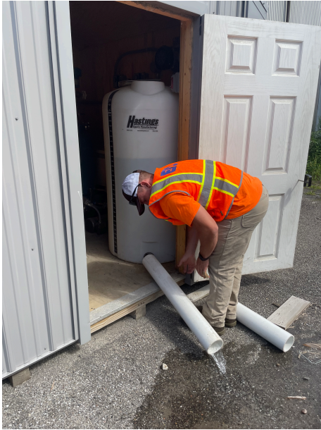
EA draining KO storage tank in PCORE-02.
