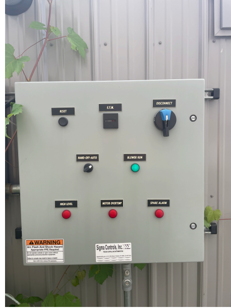
Electrical Panels for PCORE-02.
