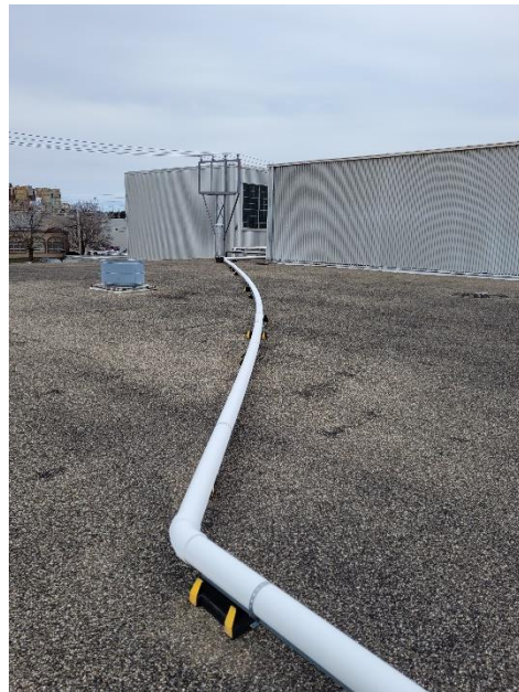
Piping on roof of PCORE building prior to being straightened.
