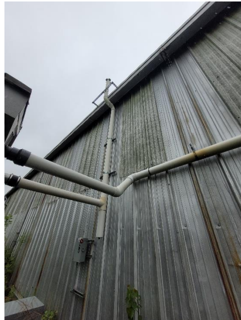
Vertical piping behind PCORE-01.
