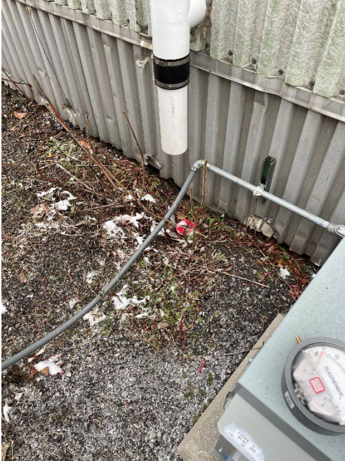
Fallen J-Plug on PCORE Shed 1
