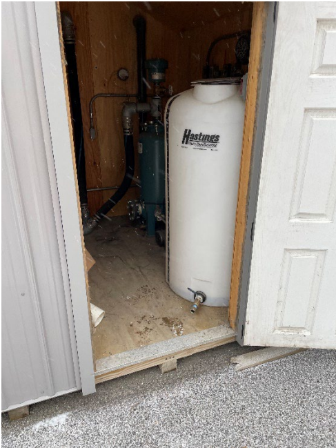
Knockout tank PCORE Shed 2
