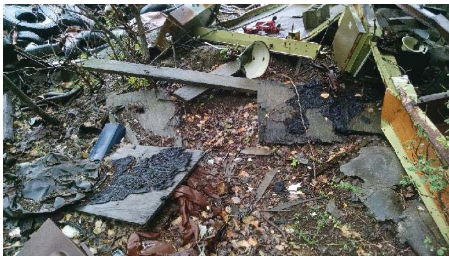
Photo 15. Homogeneous area P11-2; Black roofing tar and paper material; Trace Amount Asbestos Detected.
