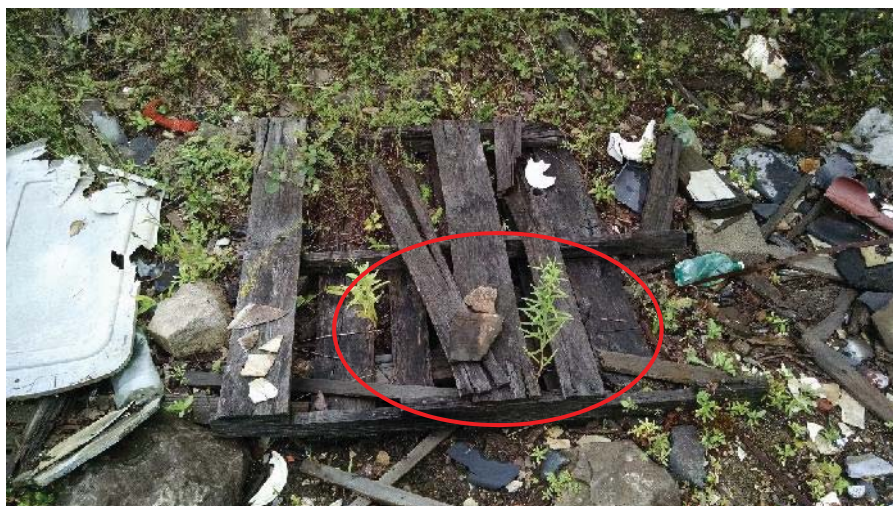
Photo 11. Homogeneous area P7-5; Gray composite (transite) subfloor; 19 % Chrysotile Detected.
