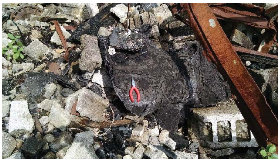
Photo 4. Homogeneous area P2-1; Black tar roofing material; Trace Amount of Asbestos Detected.
