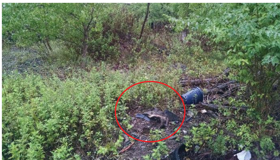
Photo 18. Homogeneous area P12-1; White matting insulation and general setting in P12; Trace Amount Asbestos Detected.
