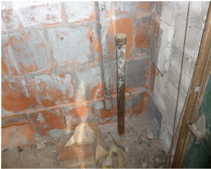
Suspect pipe in northwest interior corner of Vacant Garage.
