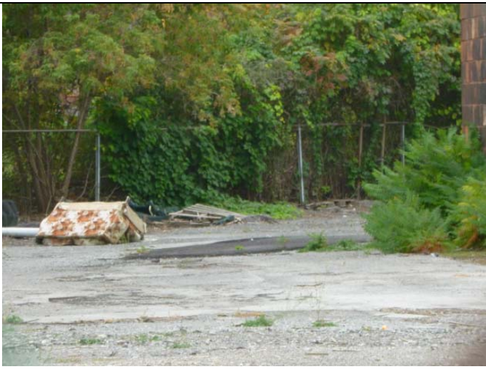
Suspect patch southeast of the Vacant Garage.
