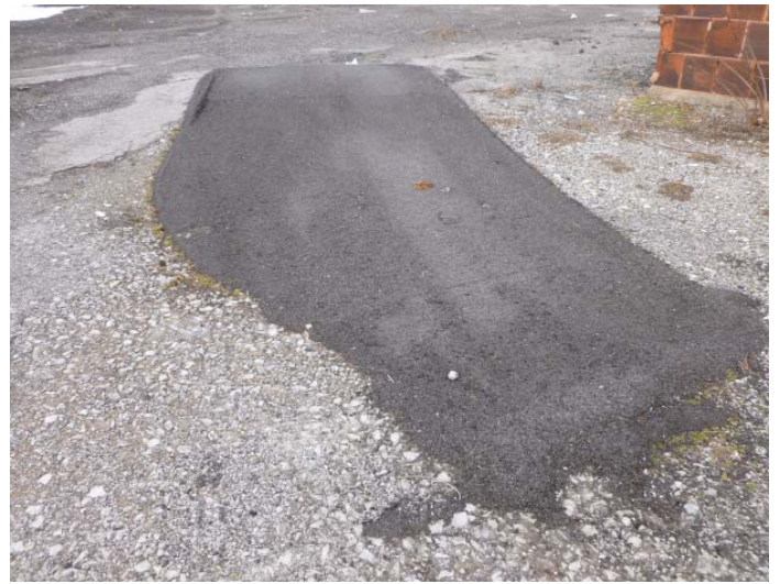
Area of unknown patching southeast of Vacant Garage.
