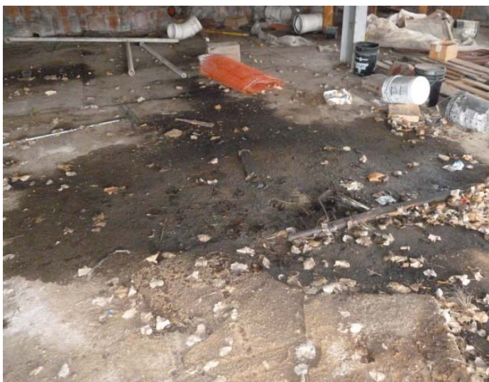
Staining noted to the concrete floor in Vacant Garage.
