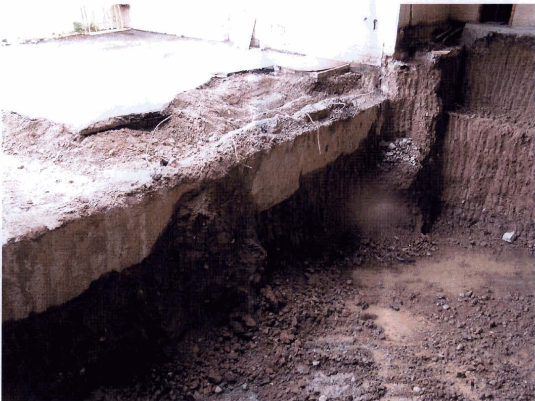
Photo #8. South wall of the excavation showing existing wall footer, bench on west wall, and appearance of groundwater at base of excavation at approx. 14 feet.
