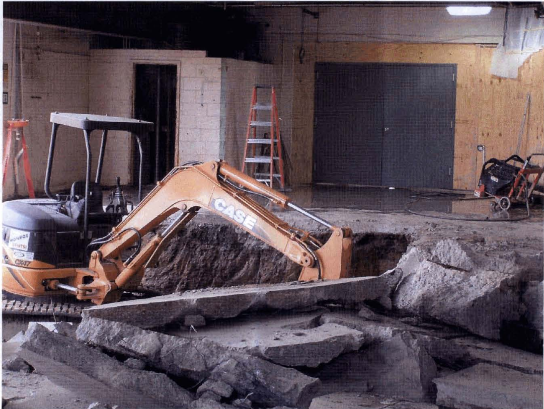
Photo #3. Concrete and soil removal activities in the western portion of the excavation.
