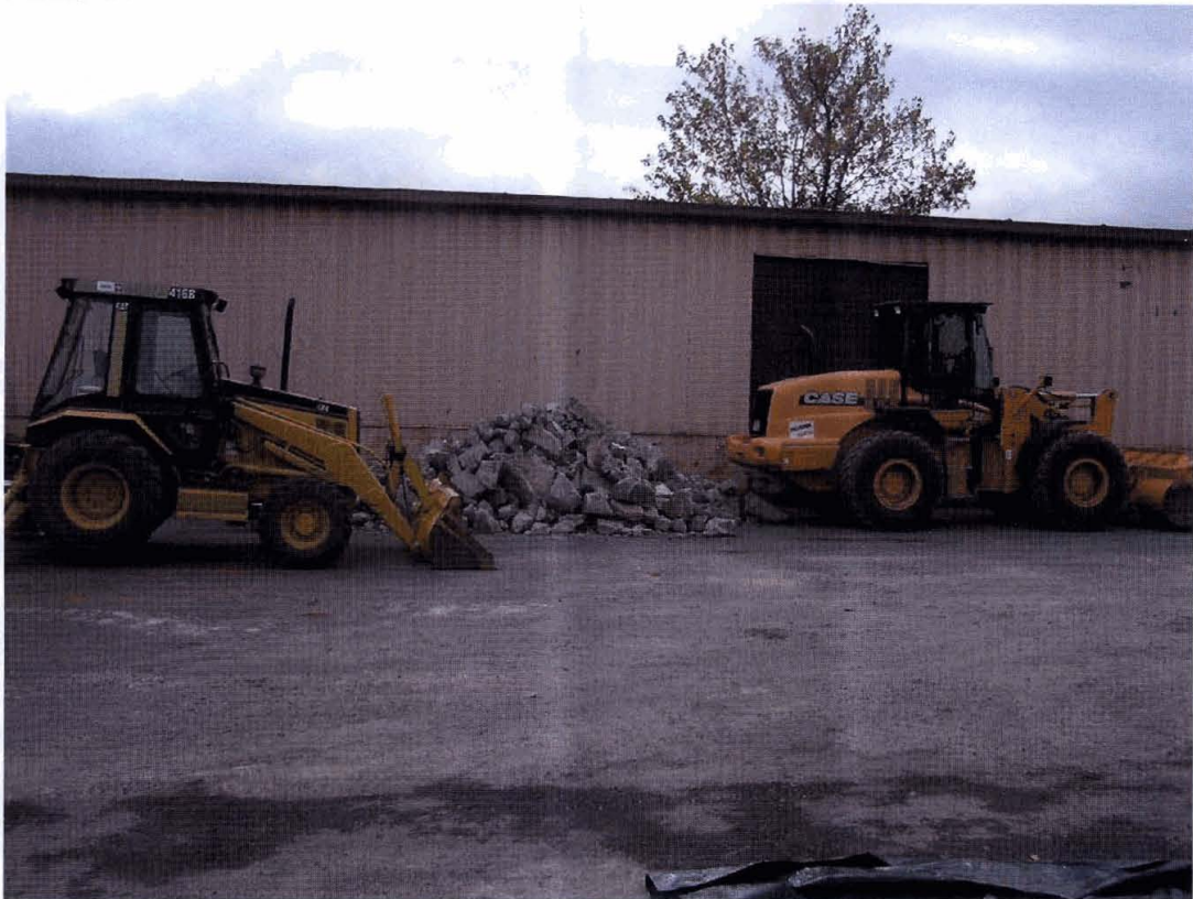
Photo #1. Concrete and general C&D debris staging area on the west side of the storage building.
