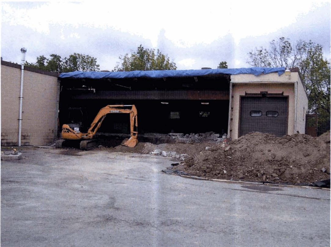
Photo #2. Interior soil removal activities and soil staging on plastic liner outside of the building east wing.
