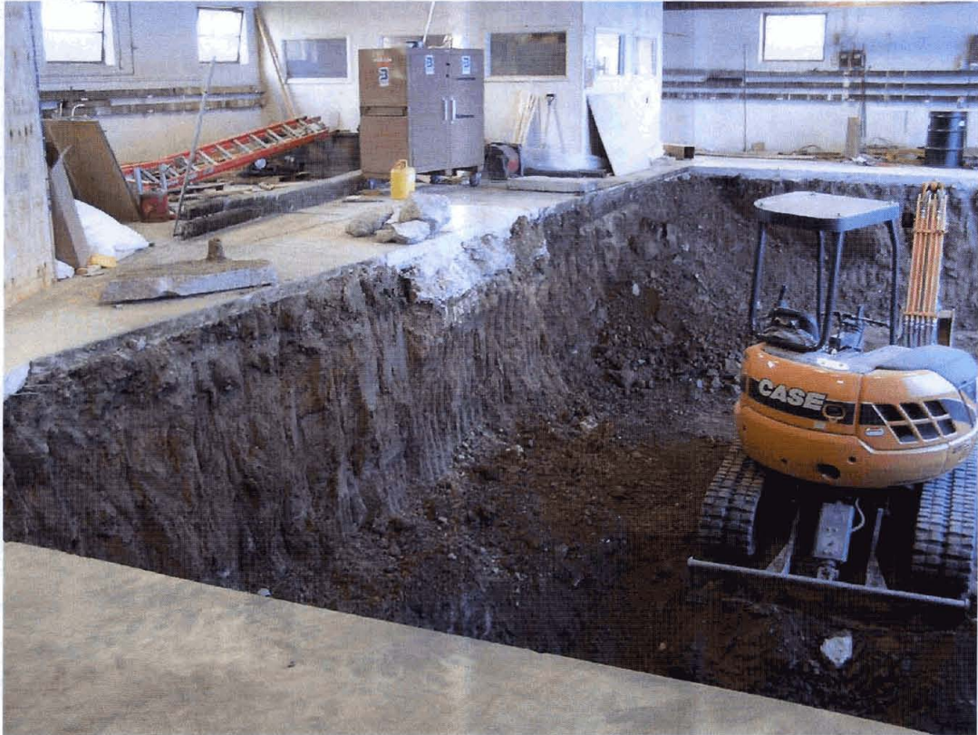
Photo #5. Working on northern half of excavation. Note deep excavation in the foreground (western portion) and the bench along the north wall.
