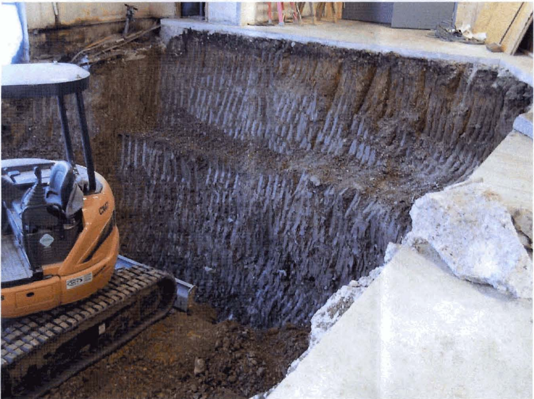
Photo #6. West side of excavation down to approximately 14 feet below floor. Note benched excavation wall.
