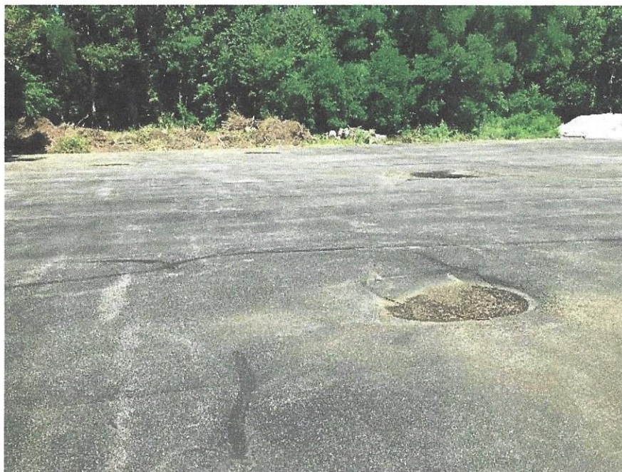
Photo 3 – Owner fill along Northwest edge of property (note settlement areas of asphalt)
