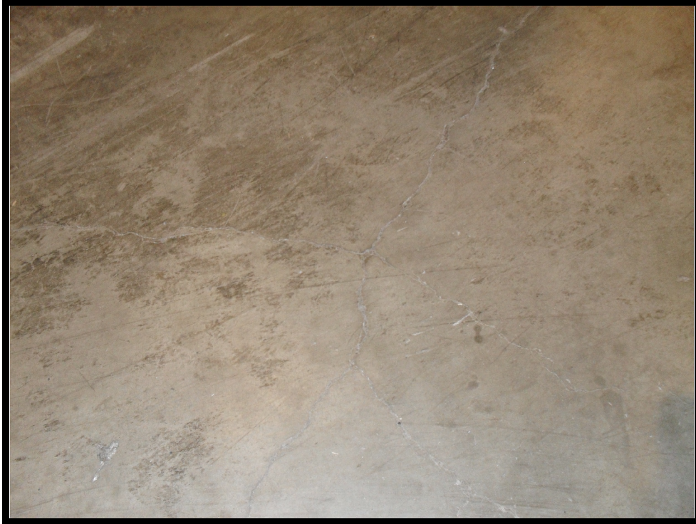
Location #27 – Floor crack
