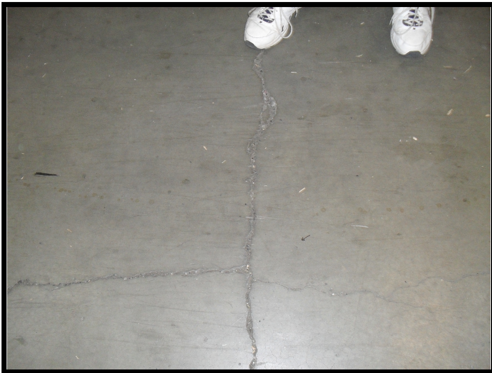
Location #29 – Floor crack
