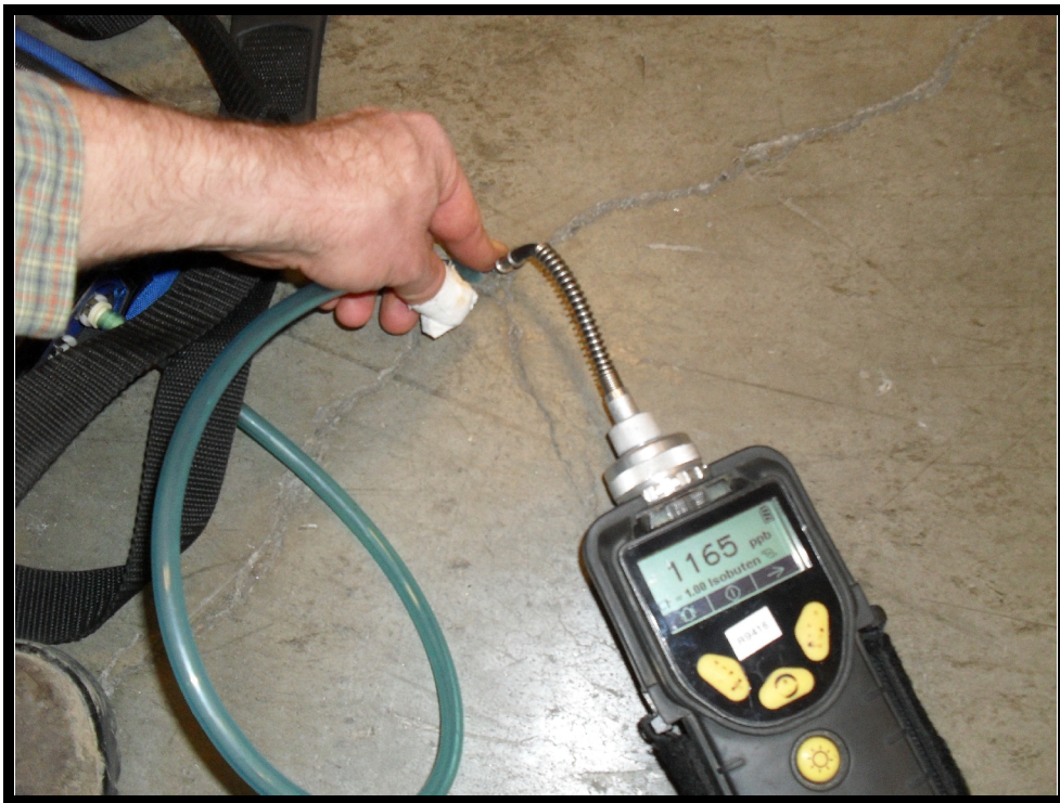
Location #25 – Floor crack
