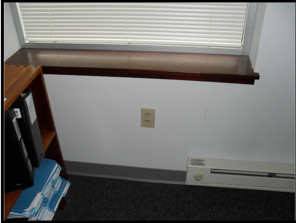
Location #17 – Electrical outlet
