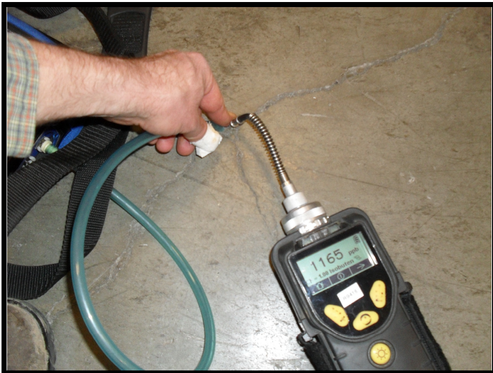
Location #25 – Floor crack
