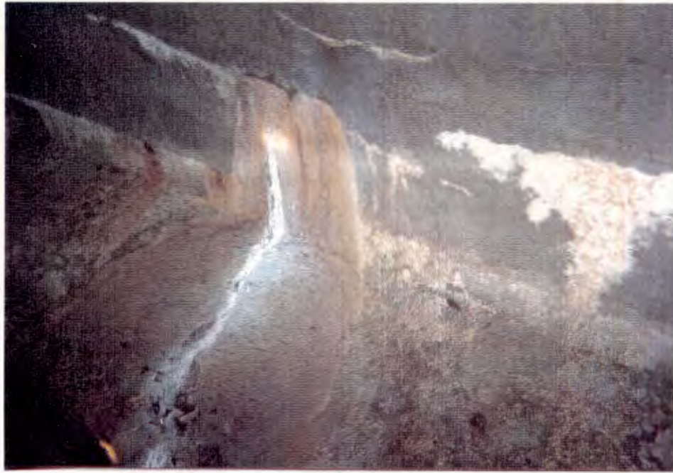
7. Same seep at 225' East of shaft, south side of tunnel (seep located approx. at Tunnel Station 75+15).
