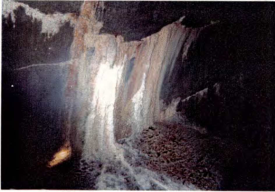
11. Same seep at 462 ft. East of shaft, north side.
