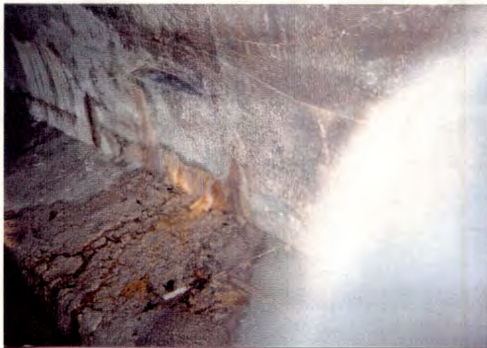
19. Seep at base of south wall of Tunnel 134 ft. west of shaft--No oil observed--No sample collected. (Tunnel Station 71+56).
