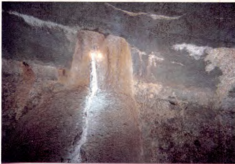
6. Seep in south wall of Tunnel 225 ft. east of shaft. Note accumulation of mineral deposits. Sample of groundwater collected here. (Tunnel Station = 75+15).
