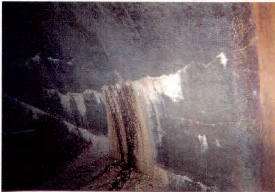
8. Seep in south wall of Tunnel 440 ft. East of shaft (seep located approx. at Tunnel Station 77+30). Dark material appeared to be oily but was determined not to be so upon examination at the project laboratory.
