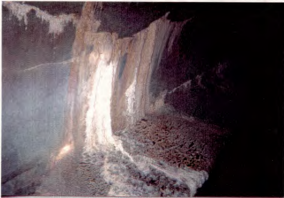
10. Seep on north side of Tunnel 462 ft. East of shaft (at Tunnel Station 77+52)--No oil observed. Groundwater sample collected.
