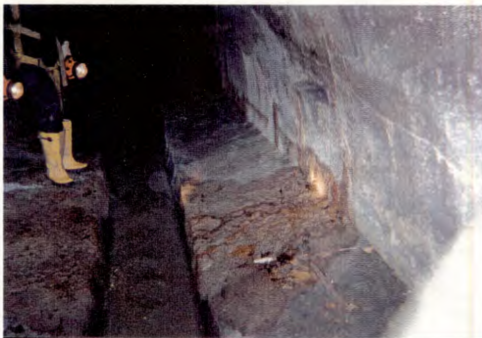
20. Same seep at 134 ft. west of shaft.
