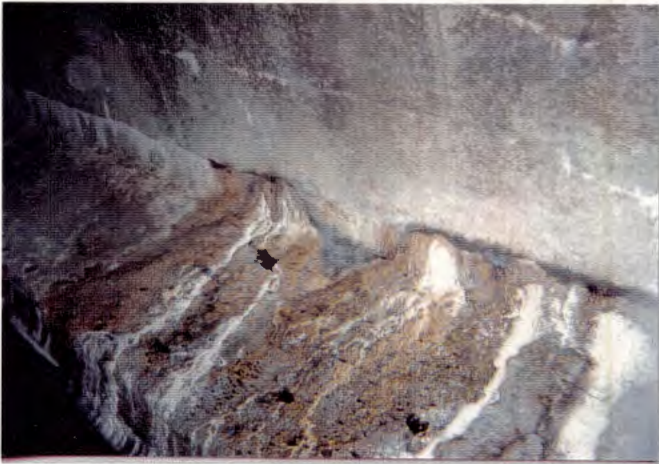
18. Same seep in south wall 20 ft. west of shaft.
