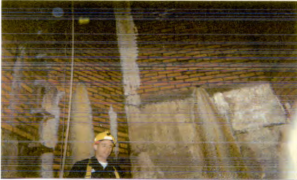
1. Shaft at Tunnel Station 72+90. The east wall of the tunnel is the concrete and brick wall in the right half of the picture. Person is standing on shelf 3'10' above the tunnel invert--Seeps above his head and at the top of the concrete are from built-in weep holes.
