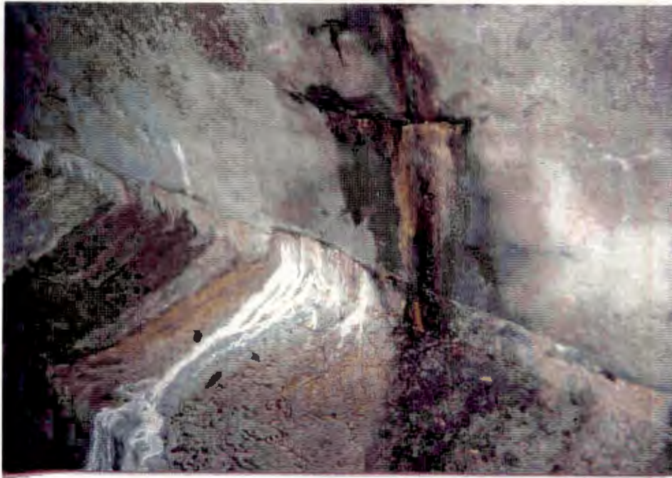
15. Oil seep in south wall of Tunnel 101 ft. East of shaft. Sampled oily mineral deposits at this location. No freely flowing oil or water observed from oily section. (Tunnel Section = 73+91).
