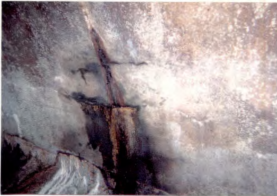
16. Same oily seep on south wall 101 ft. East of shaft.
