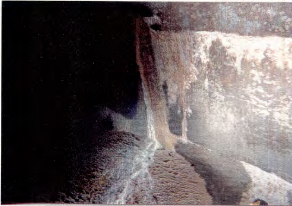
12. Seep in north wall of Tunnel 163 ft. East of shaft (approx. Tunnel Station = 74+53)--No oil observed. GW sample collected here.
