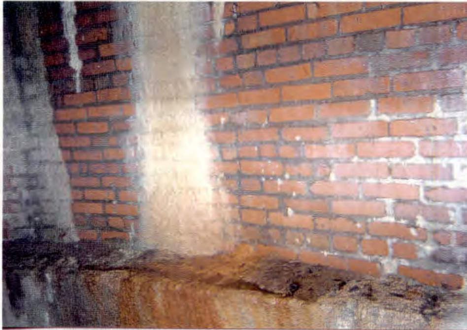
5. Rusty-orange stain from groundwater seep to base of south wall of shaft, top of shelf 3'10" above invert. Light brown mineral deposits are from a weep hole seep above.
