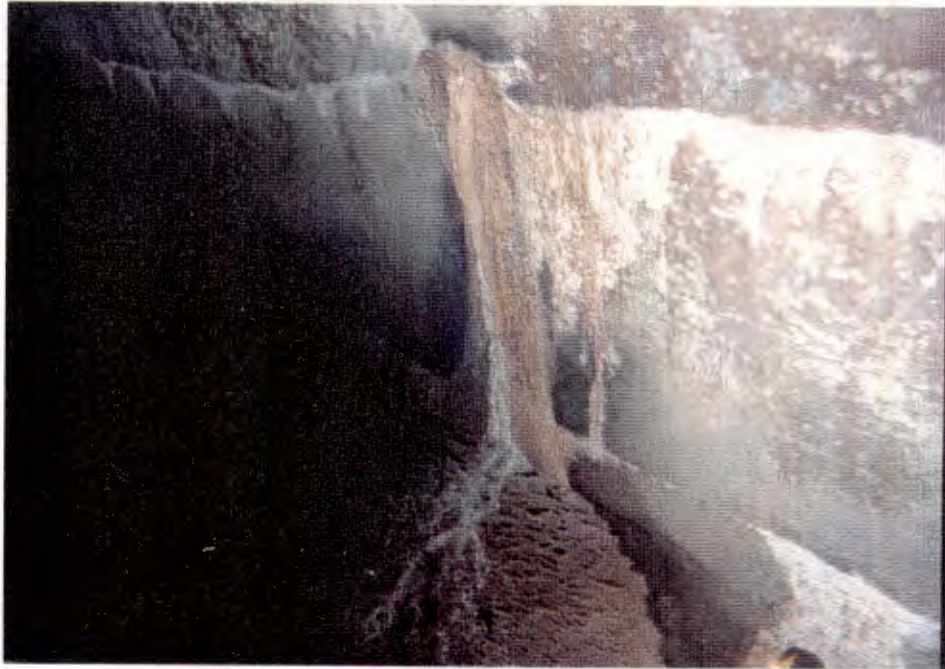
13. Same seep at 163 ft. East of shaft, north side.
