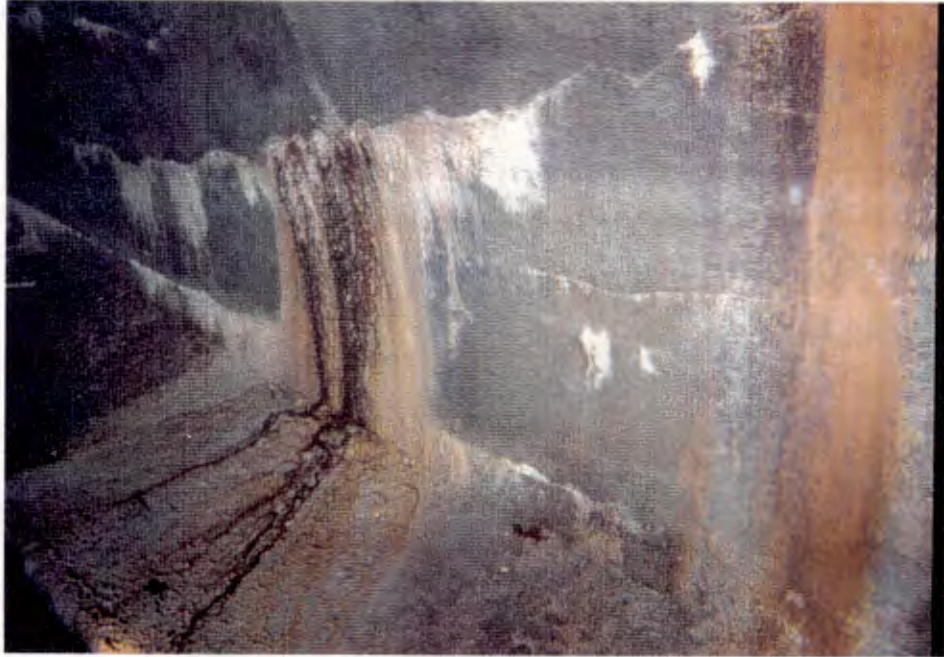
9. Seep 440 Ft. East of shaft (same as previous picture).
