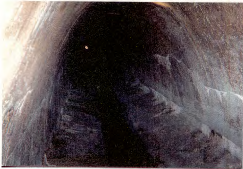
14. Looking west towards shaft at Station 72+90 from seep at Station 74+53; showing numerous inactive or very minor seeps along joint 6" above floor.
