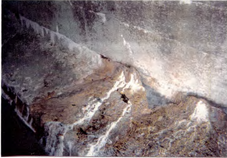
17. Seep at base of south wall 20 ft. West of 72+90 shaft, possible oil puddled on floor in accumulation of mineral material -No samples collected (Tunnel Station = 72+70).
