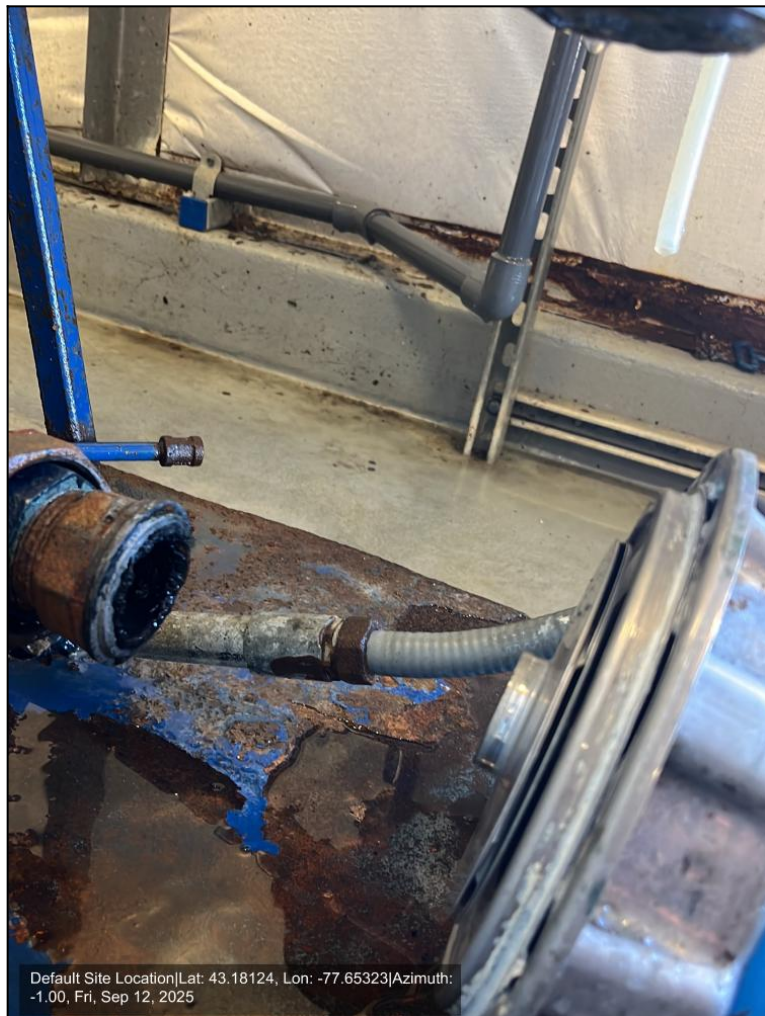
Photo Number: 4 After cleaning EWTA, for air stripper discharge pump
