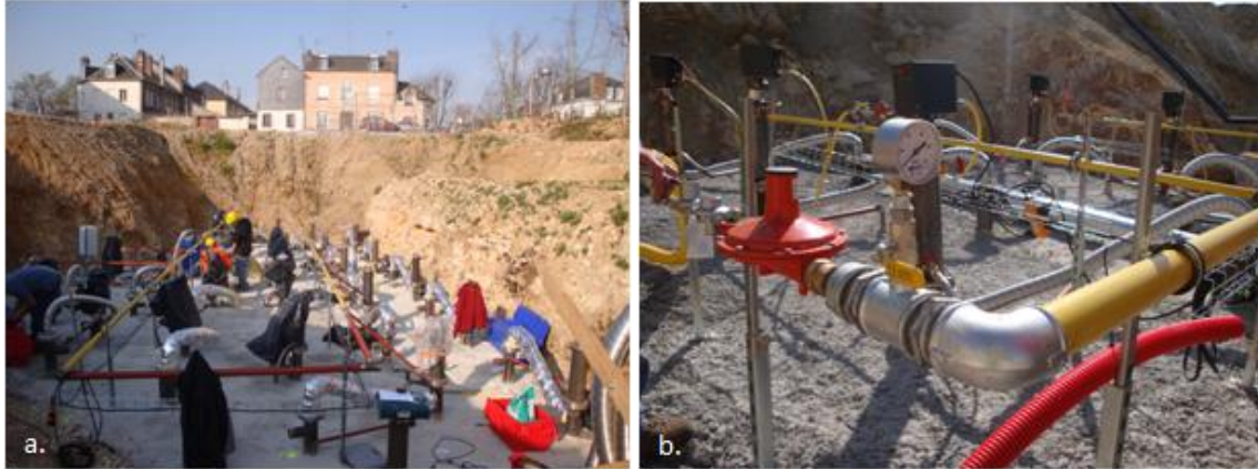
Figure 4.a). Gas distribution system being assembled to feed heaters. b). Dual redundant pressure regulators placed in series.
