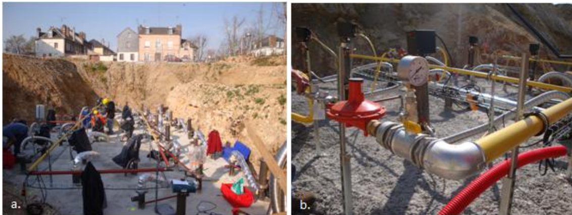
Figure 3.a). Gas distribution system being assembled to feed heaters. b). Dual redundant pressure regulators placed in series.
