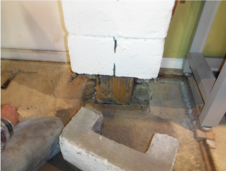
Sealing floor cracks and cracked chimney in tool room – August 2015
