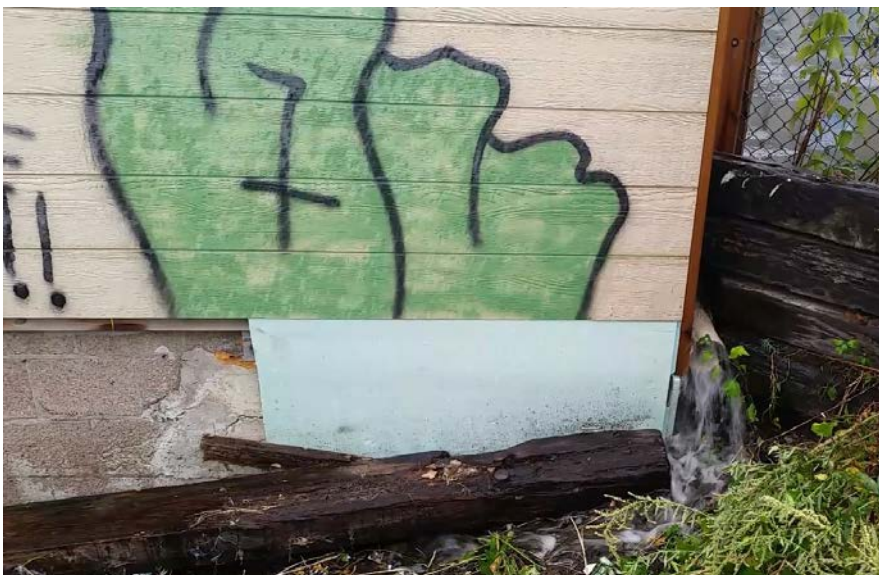
Two-inch insulation board over sealed area. Rain water shown coming off parking lot and around corner. – September 2015
