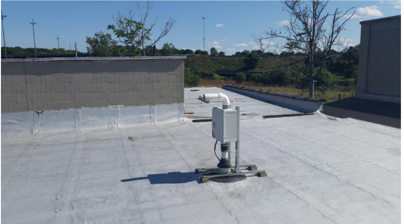
New High Pressure Fan – Obar – 76 UD on roof, looking east September 2015
