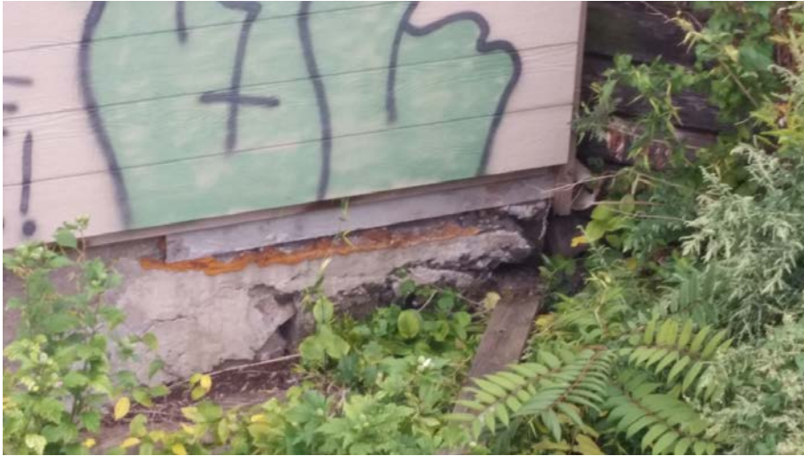
Cracked Foundation – NE corner -2015
