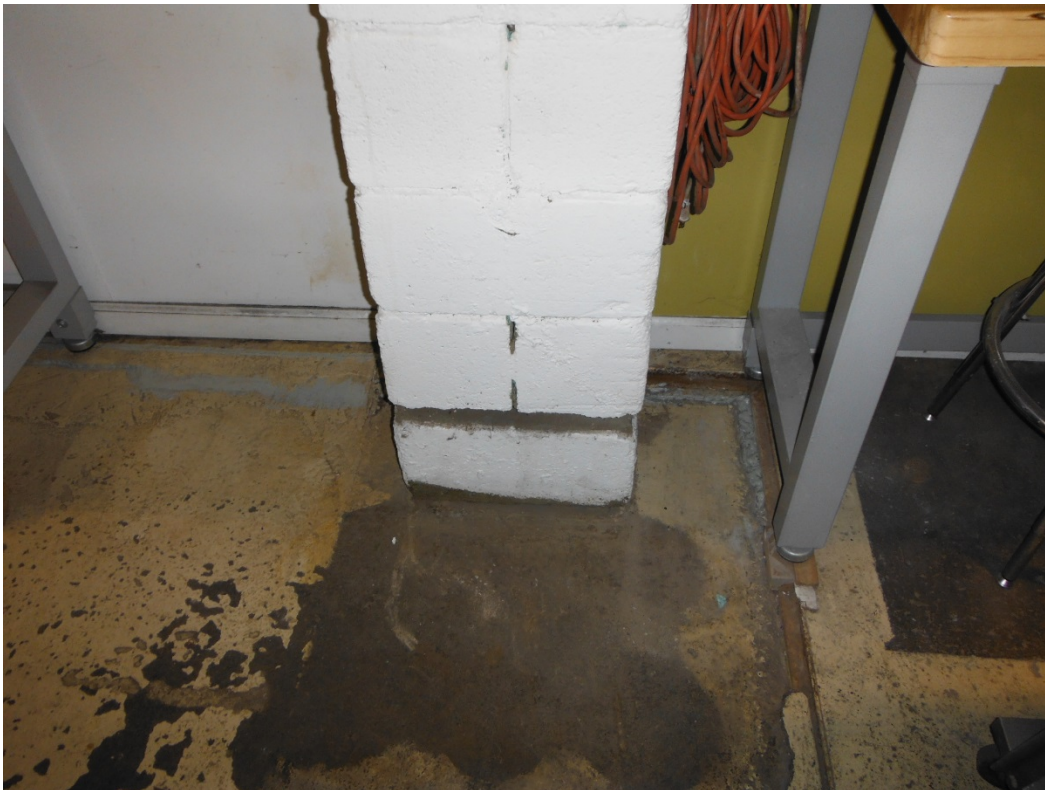
Floor Cracks and Chimney Sealed- August 2015
