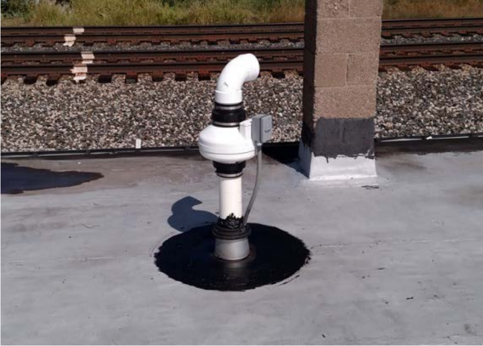
New Fan – RadonAway – RP365 – on roof, looking north - September 2015
