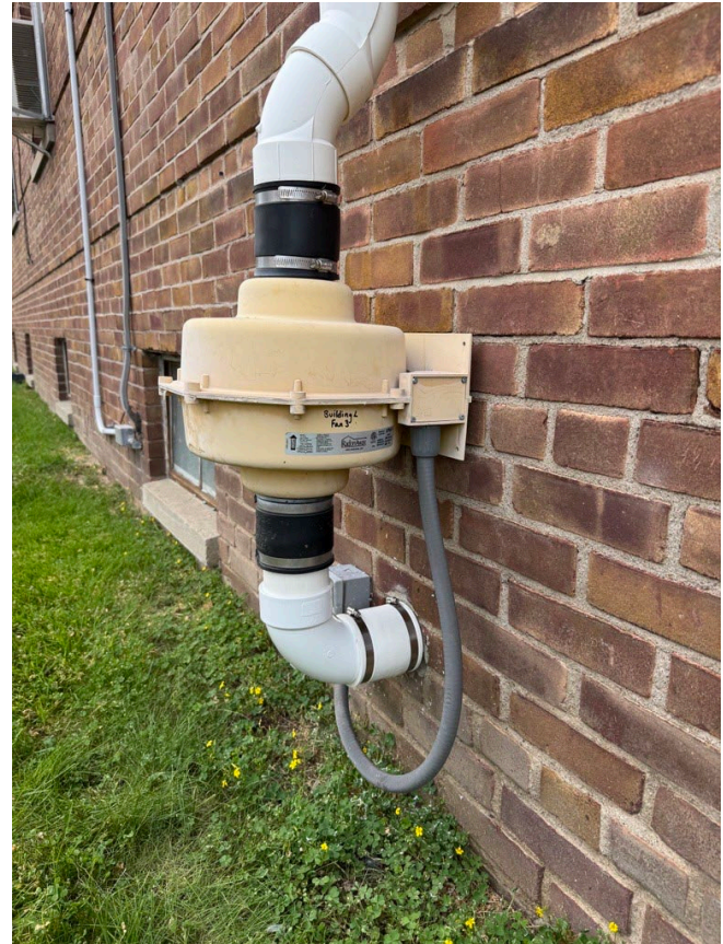
Above – Image of repairs made to exterior PVC of Building 2 Fan 3. The PVC had been cracked where the piping enters into the building.
