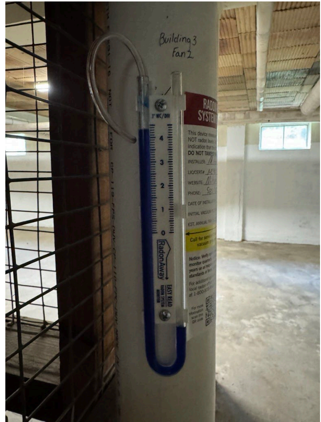
Above – Image of gauge after replacement on interior piping of Building 3 Fan 2.
