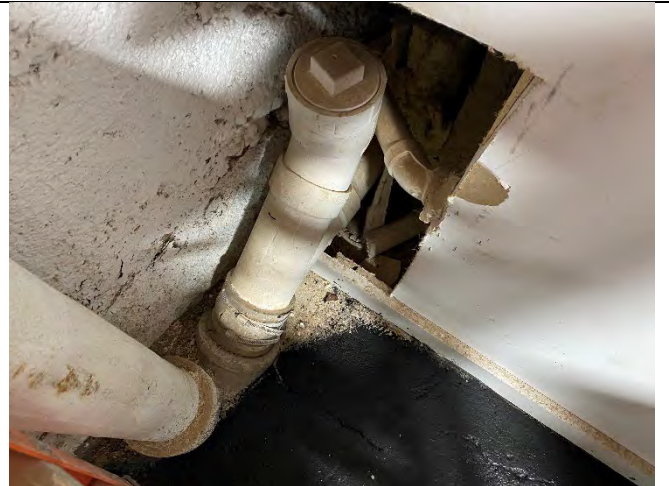
Photo 26: Piping to discharge purge water inside woodworking tenant
