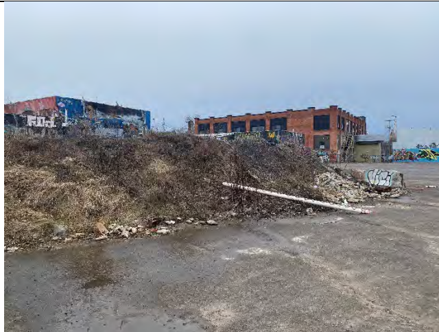
Photo 13: Pile of debris and brush in the middle of the site that has been asked to be removed
