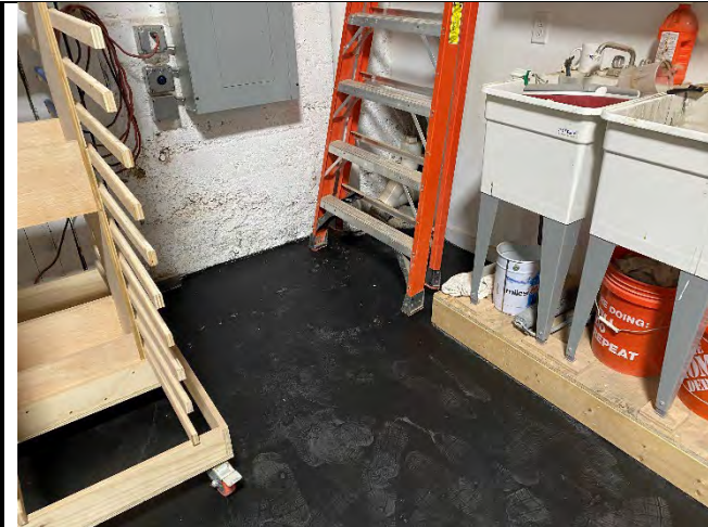
Photo 25: Piping to discharge purge water inside woodworking tenant
