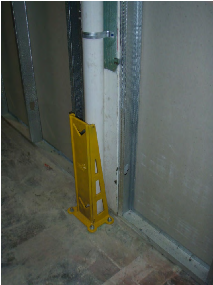
SSDS suction pipe at floor
