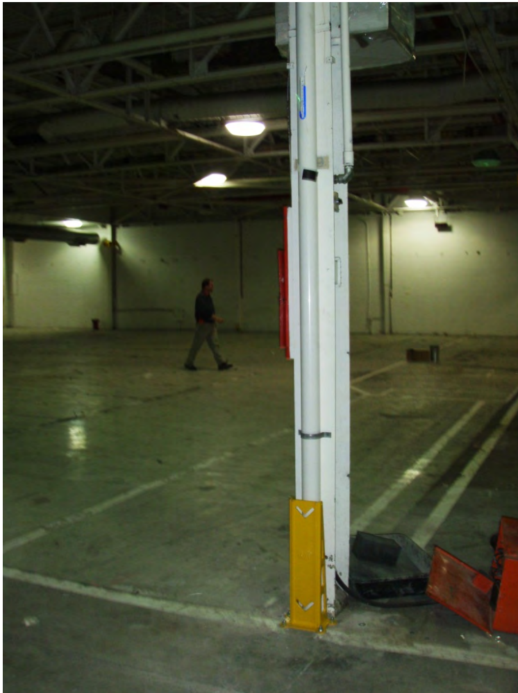
Suction pipe at column Q-19
