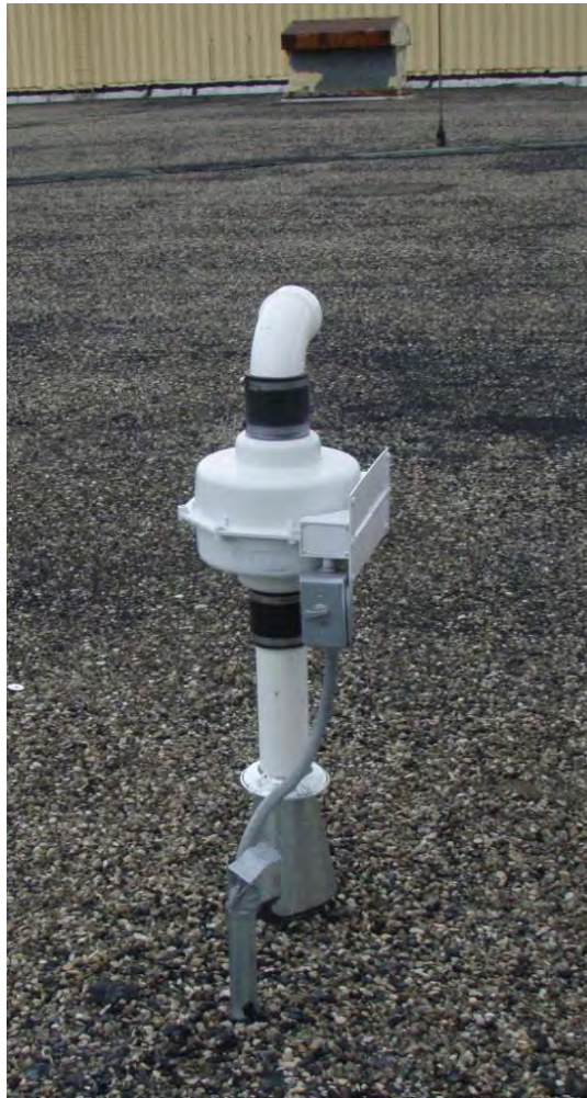
SSDS fan showing electrical switch
