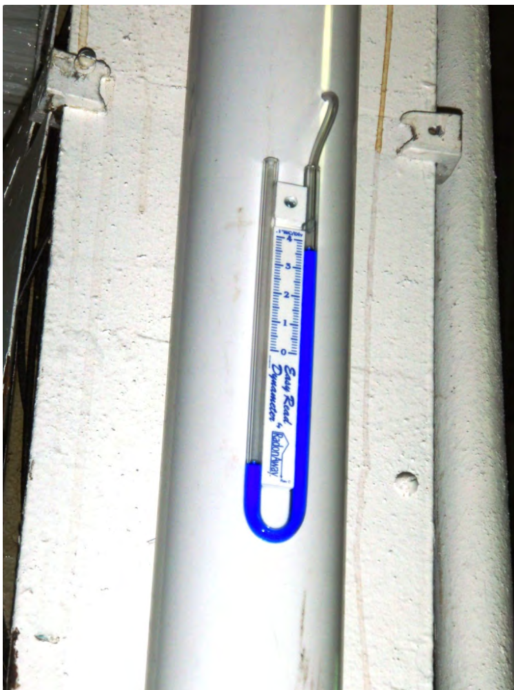
Manometer on suction pipe at column Q-19
