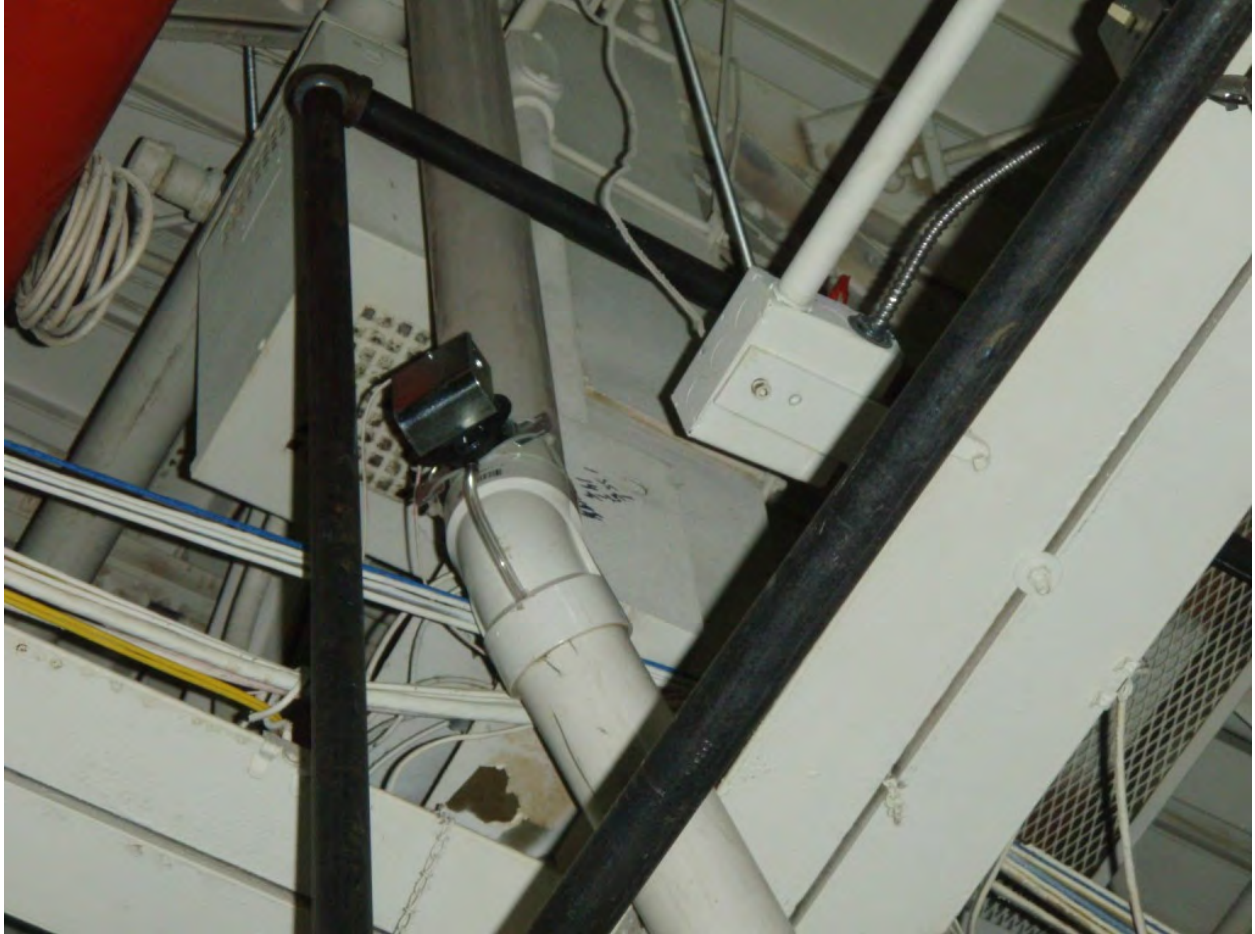
Alarm system sensor relay on suction pipe at column Q-19
