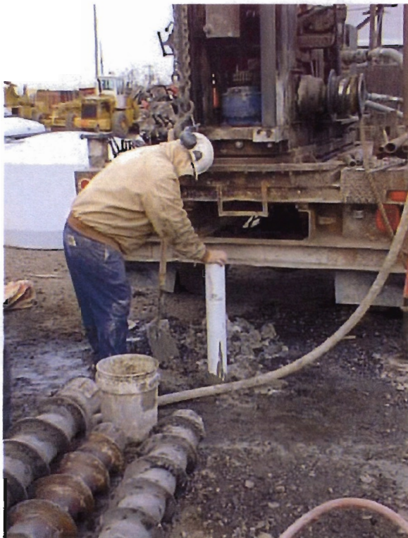
Photograph No. 7 - After removal of the hollow stem augers (foreground), the annulus between the well casing and boring wall was filled to grade with grout (MW-2D).
