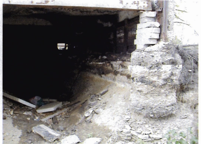
Photograph No. 4 - Access to the basement of Building C is available at the southeast corner of the building. Surface soil sample SS-3 was collected from this area of the basement.
