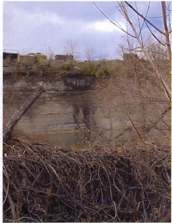
Photograph No. 2 - View of staining on the gorge wall at the Raeco Site from across the Genesee River.
