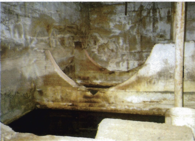
Photograph No. 3 - Standing water was present in the basement of Building B at the time of the investigation near former tank cradles. Surface water sample SW-1 and surface soil sample SS-1 were collected from this area of the basement.
