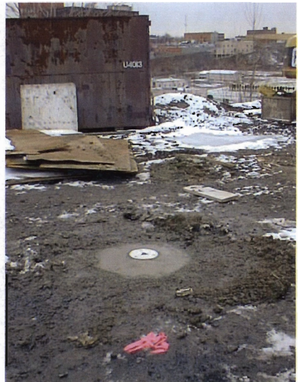
Photograph No. 8 - The monitoring wells are protected with flush-mounted steel manhole covers (MW-2D).
