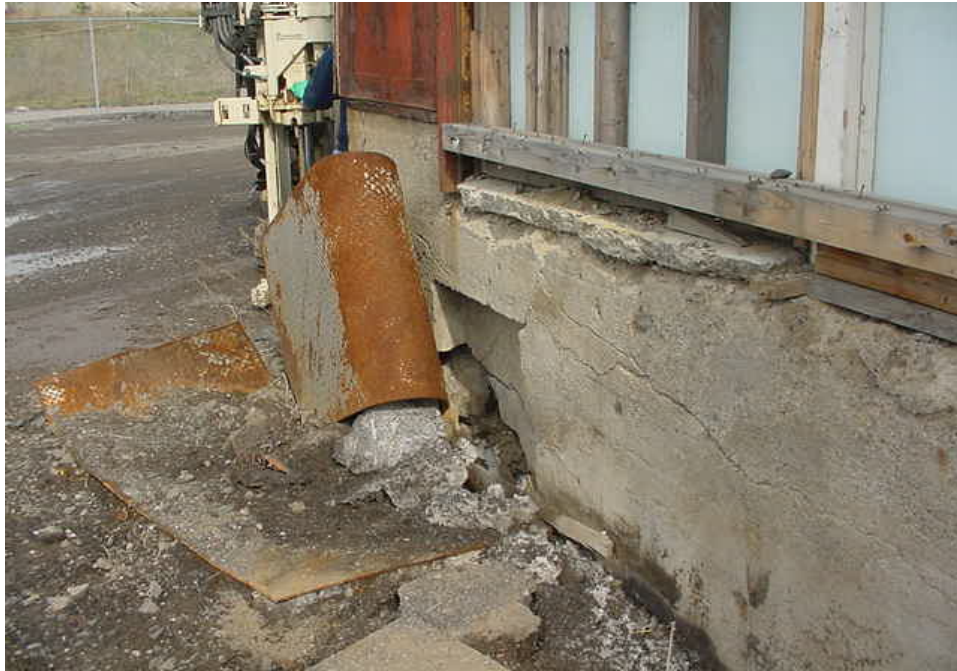
Photo 1: View looking west of steel plate covering abandoned UST access hatch/fill port on the south end of Building D.
