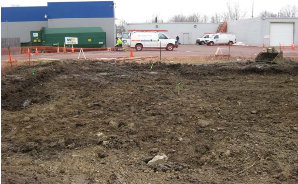
Photo #9, view to the south: depicting Area 2C upon completion of initial excavation activities.
