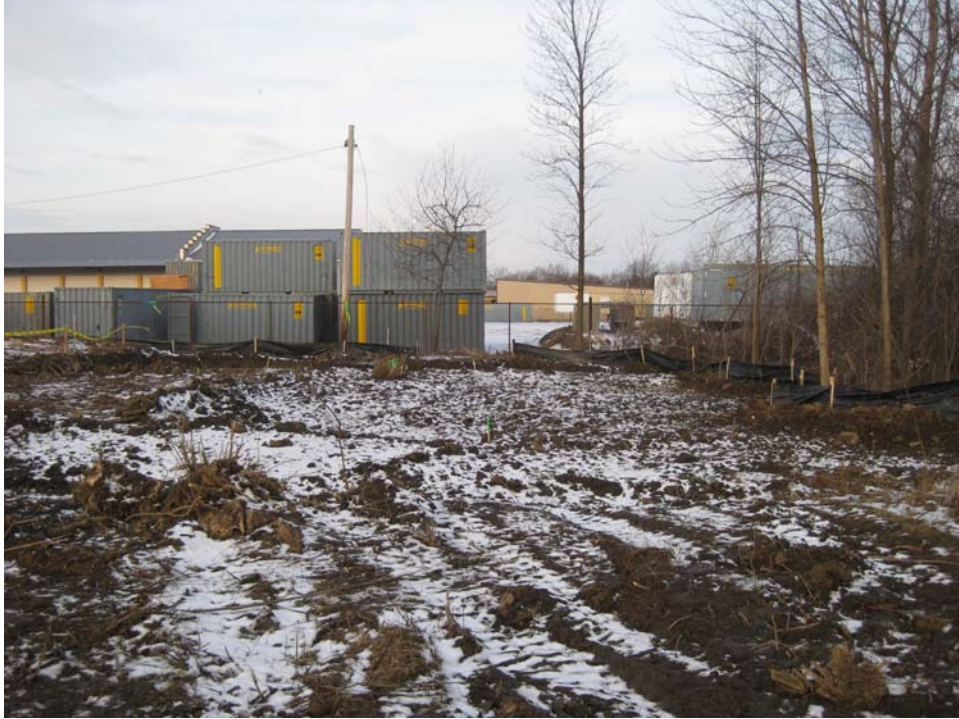
Photo #1, view to the west: depicting the northern portion of Areas 2A and 2B upon completion of initial excavation activities.
