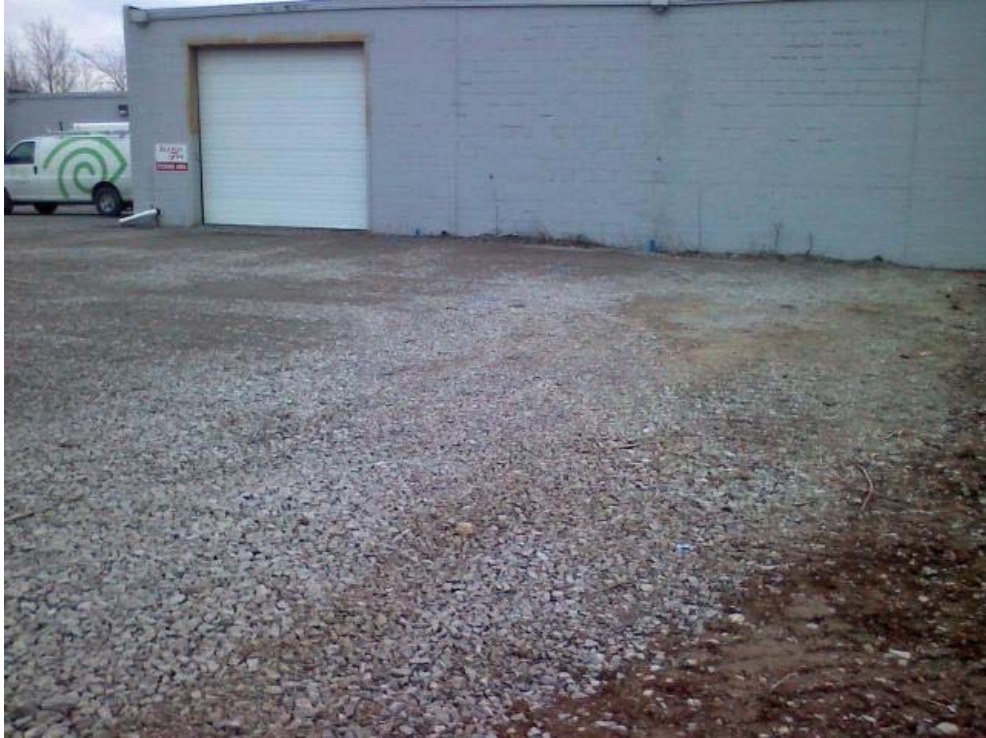
Photo #25, view to the southeast: depicting Area 1A upon completion of backfilling and grading activities.
