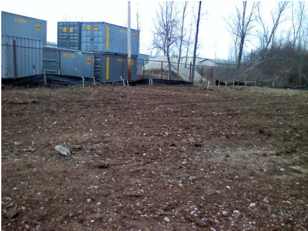
Photo #23, view to the northwest: depicting Areas 1C, 2A, and 2B upon completion of backfilling and grading activities.
