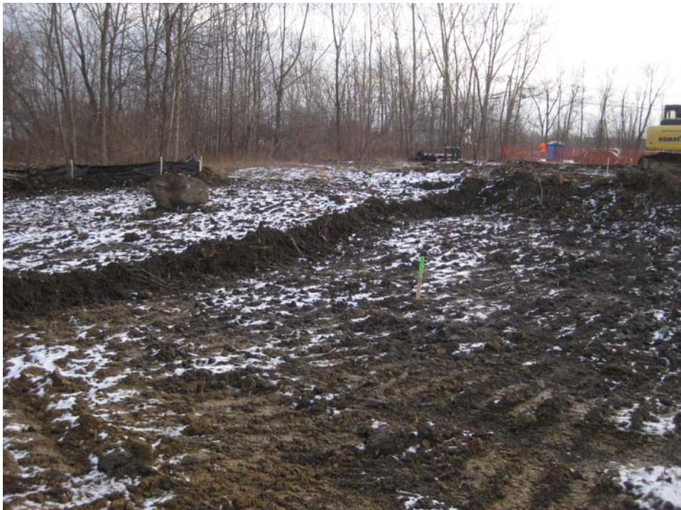
Photo #2, view to the northeast: depicting the southern portion of Areas 2A and 2B upon completion of initial excavation activities.
