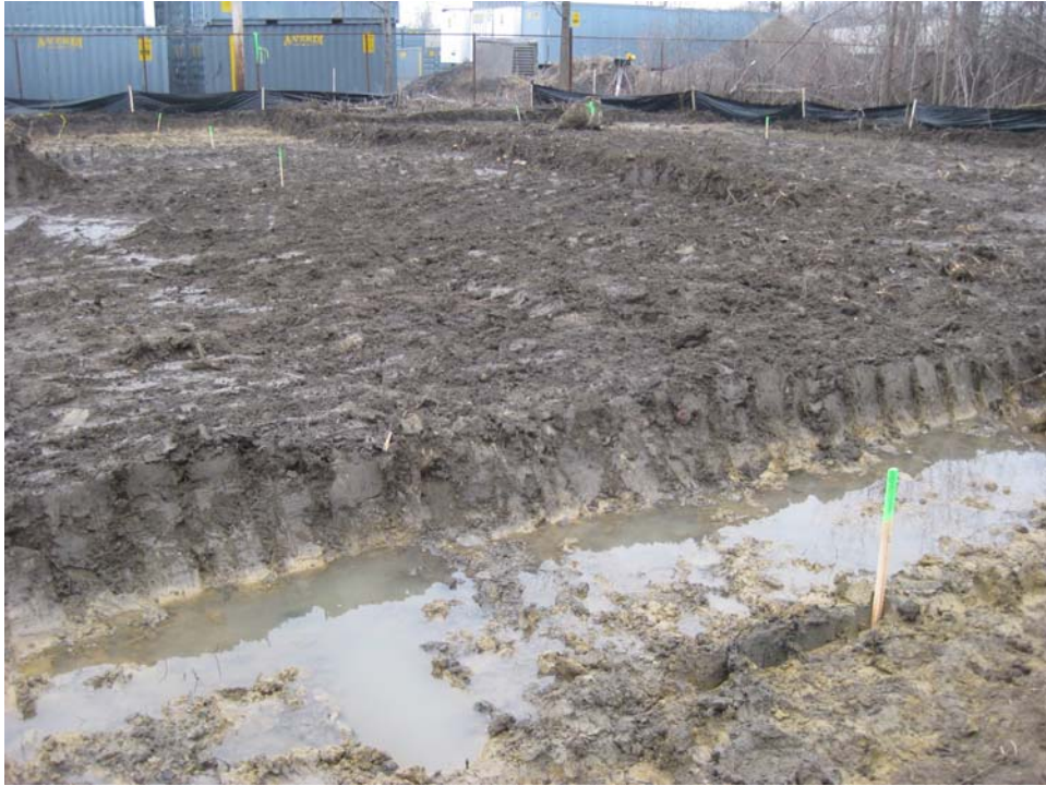
Photo #7, view to the northwest: depicting Areas 2A and 2B upon completion of initial excavation activities.
