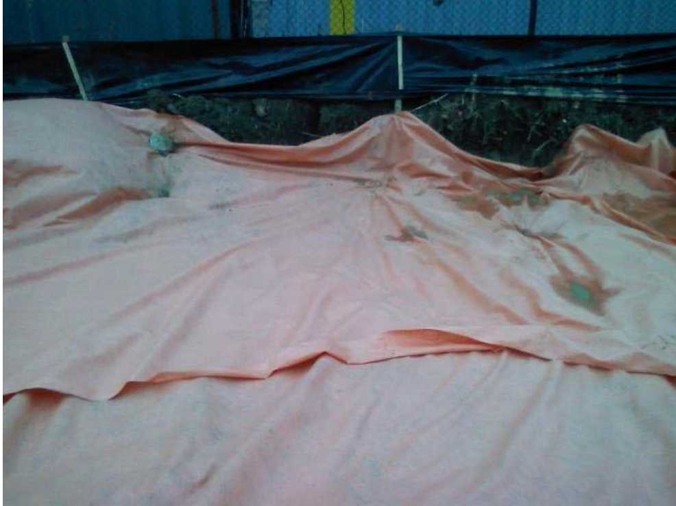
Photo #17, view to the west: depicting placement of orange demarcation fabric prior to backfilling in Area 1B.
