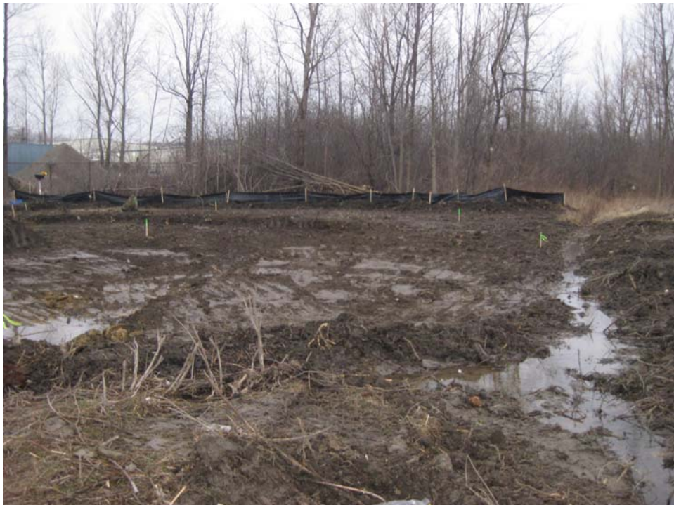
Photo #4, view to the north: depicting Areas 2A and 2B upon completion of initial excavation activities.
