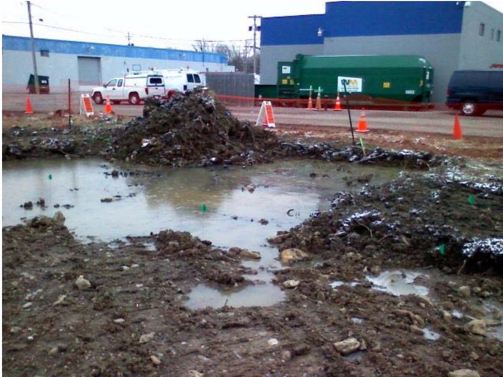
Photo #15, view to the southeast: depicting the southern portions of Area 1C upon completion of over-excavation activities.
