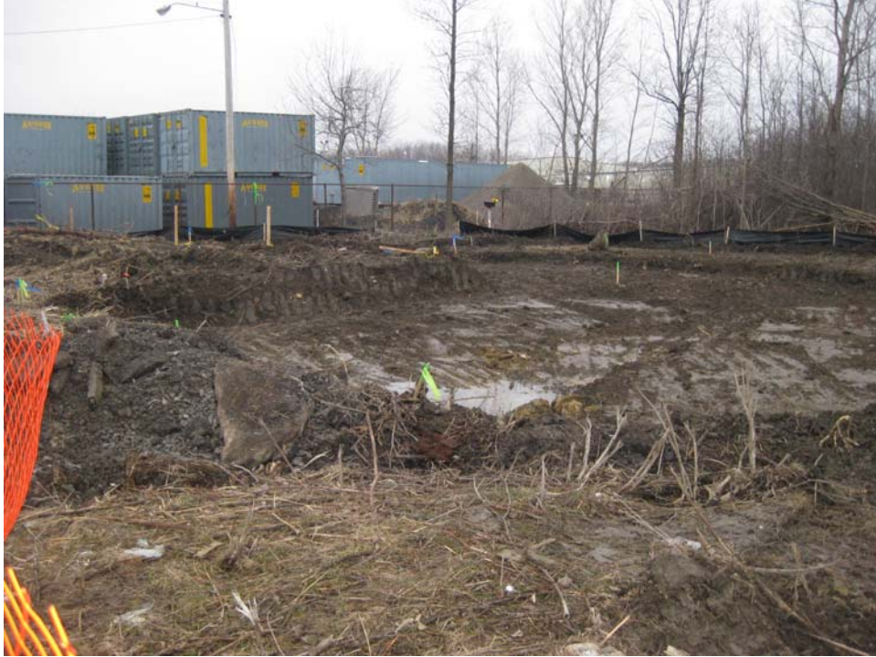
Photo #3, view to the northwest: depicting the Areas 2A and 2B upon completion of initial excavation activities.
