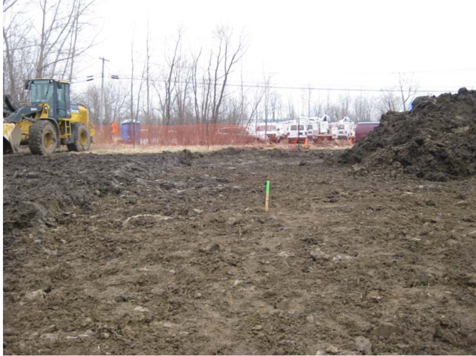
Photo #5, view to the east: depicting Area 2C during initial excavation activities.
