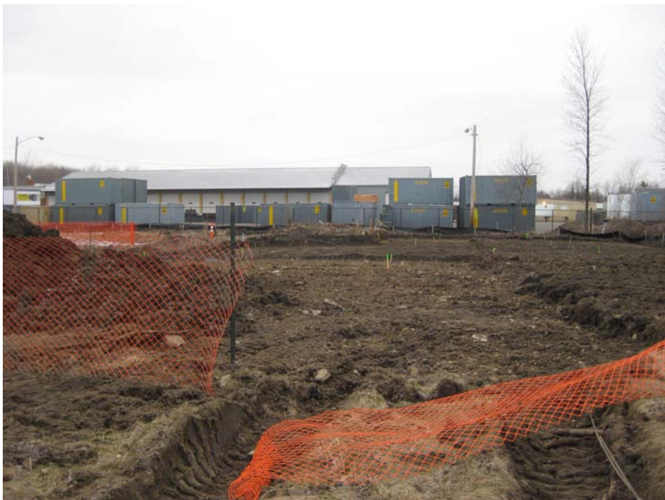
Photo #8, view to the west: depicting Areas 2A, 2B, and 2C upon completion of initial excavation activities.
