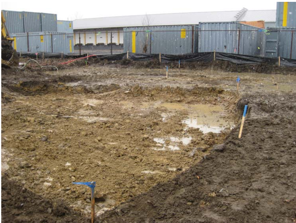
Photo #10, view to the southwest: depicting Area 1C upon completion of initial excavation activities.
