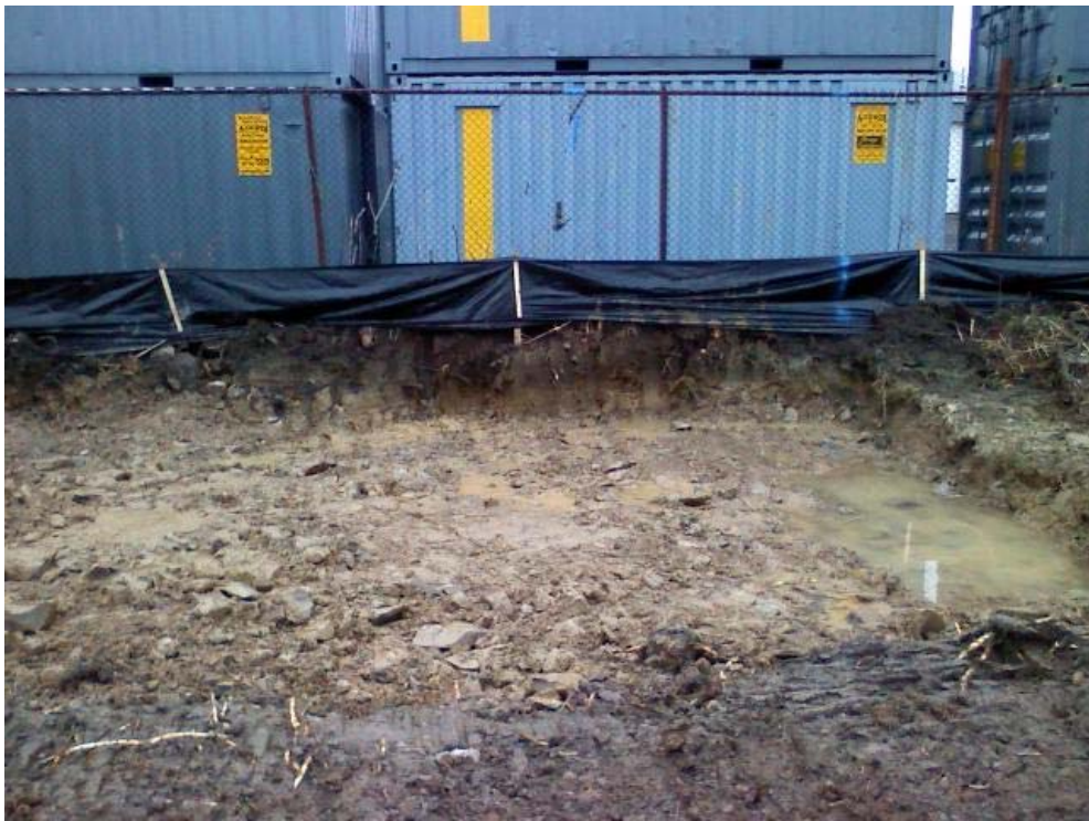
Photo #16, view to the west: depicting Area 1B upon completion of over-excavation activities.
