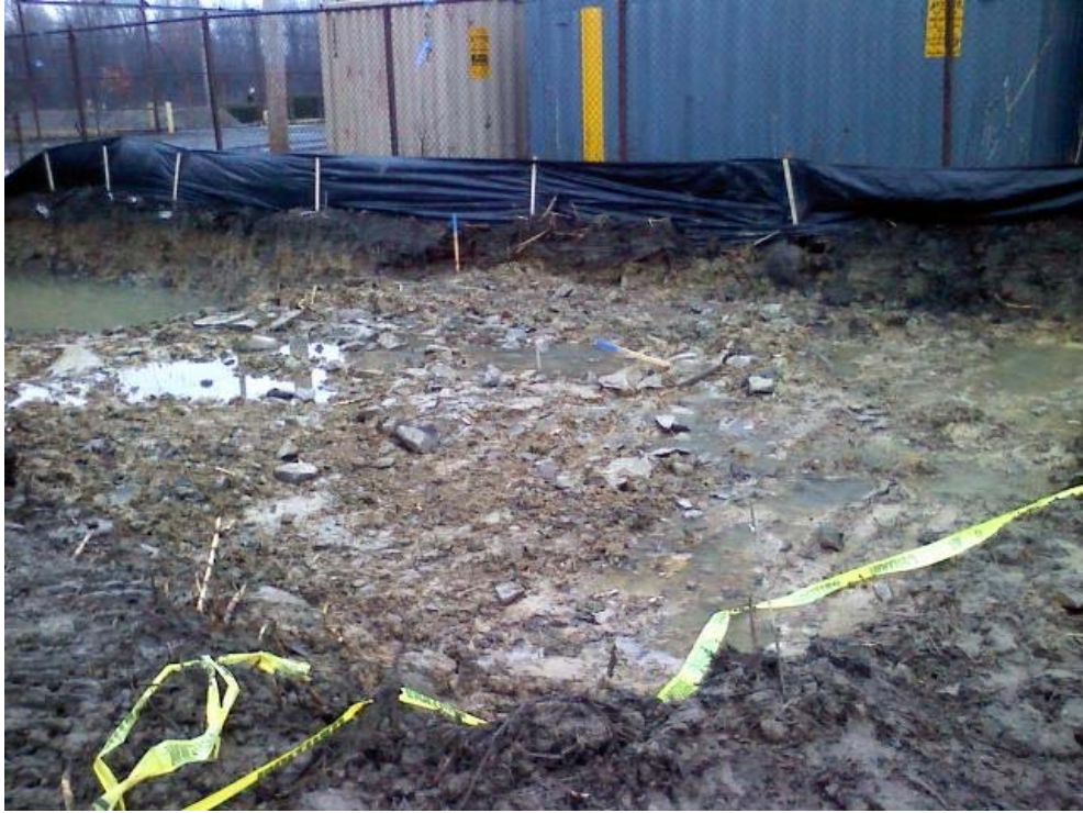
Photo #13, view to the southwest: depicting the northern portion of Area 1B during initial excavation activities.
