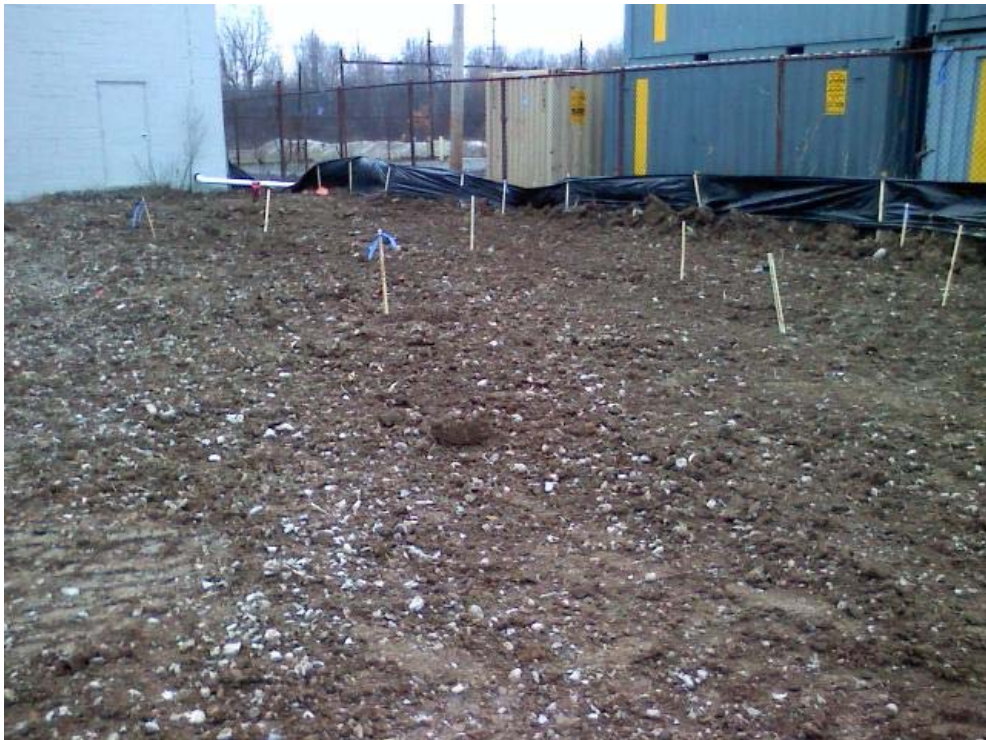
Photo #24, view to the southwest: depicting Area 1B upon completion of backfilling and grading activities.
