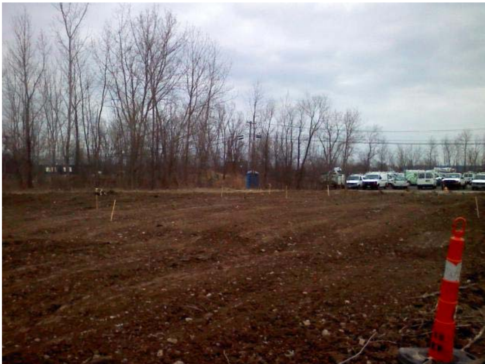
Photo #22, view to the northeast: depicting Areas 1C, 2A, 2B, and 2C upon completion of backfilling and grading activities.
