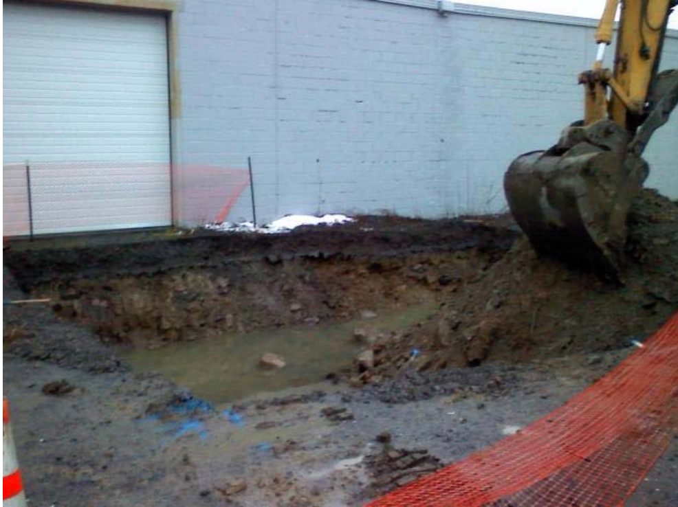
Photo #11, view to the southwest: depicting Area 1A during initial excavation activities.
