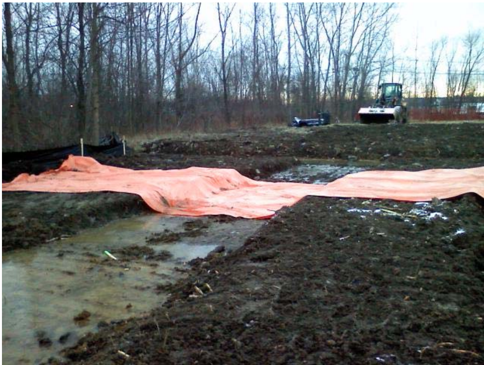
Photo #14, view to the east: depicting the northern portions of Area 1A and 1B. Upon completion of over-excavation activities, orange demarcation fabric was placed prior to backfilling.
