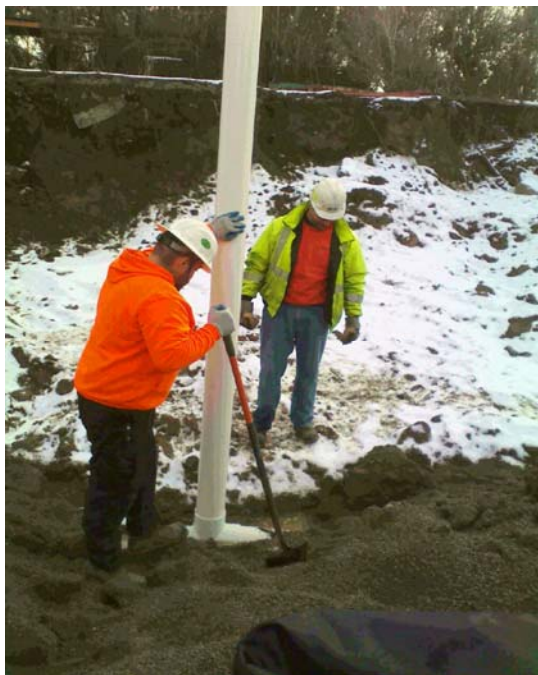
Construction of Injection Well INJ-1 within Operable Unit 01A (Former Drum Storage Area) excavation.
