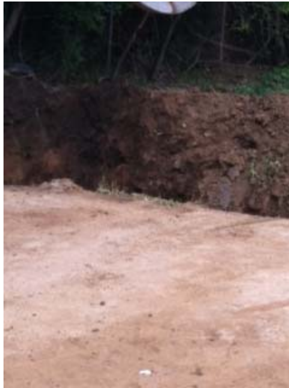
View of Operable Unit 01C (Outside Disposal Area) extended excavation in September 2012, looking at the southwestern corner.
