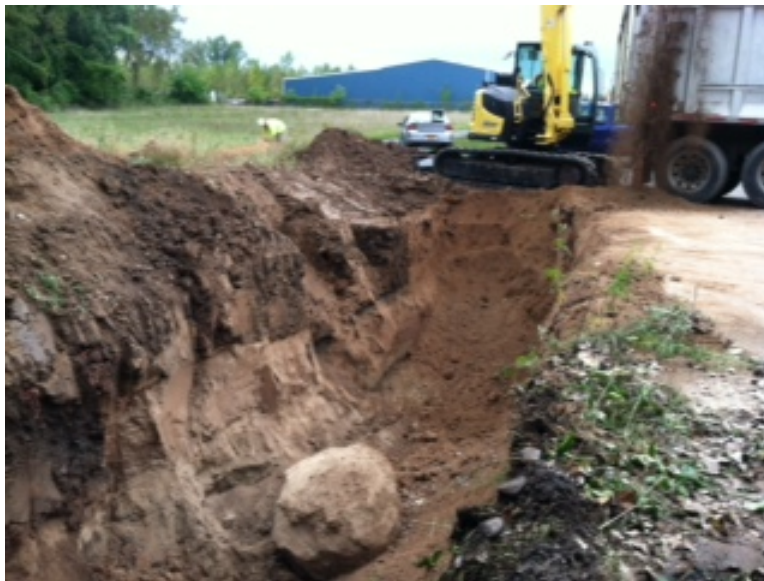
View of Operable Unit 01C (Outside Disposal Area) extended excavation in September 2012, looking at the northern wall.
