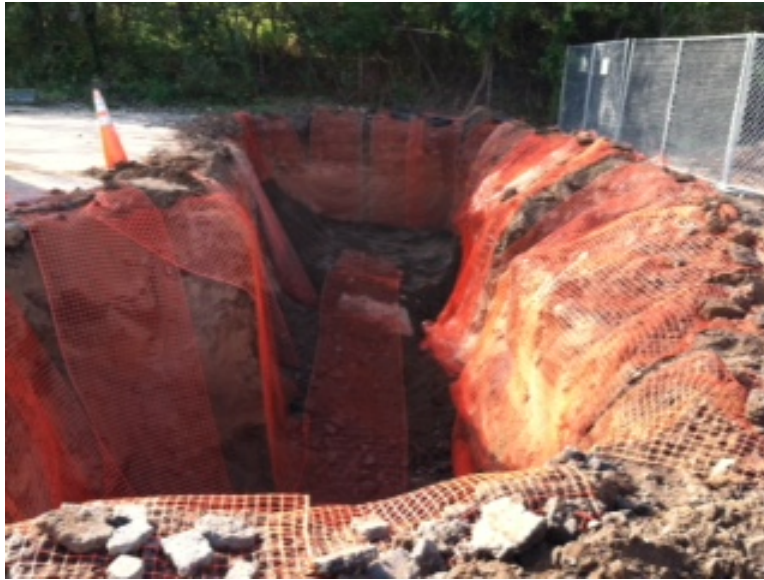
View of Operable Unit 01C (Outside Disposal Area) extended excavation in September 2012, looking south, with demarcation barrier placed.
