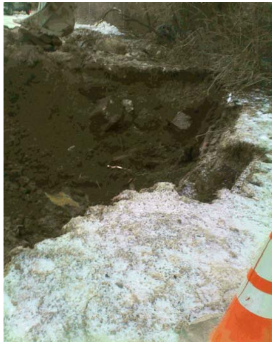
View of northern portion of Operable Unit 01C (Outside Disposal Area) excavation.
