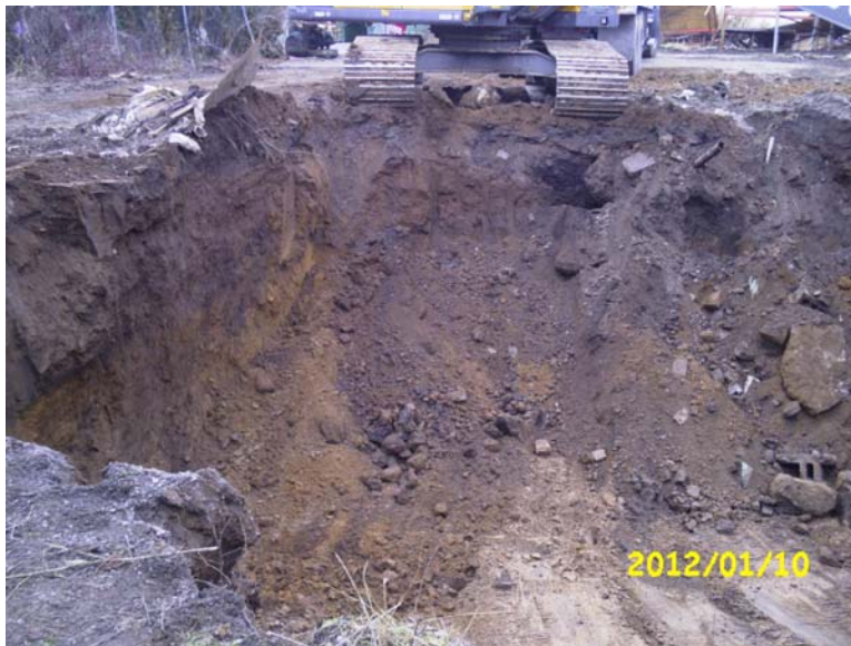
View of the eastern portion of the Operable Unit 01A (Former Drum Storage Area) excavation, following further soil removal.
