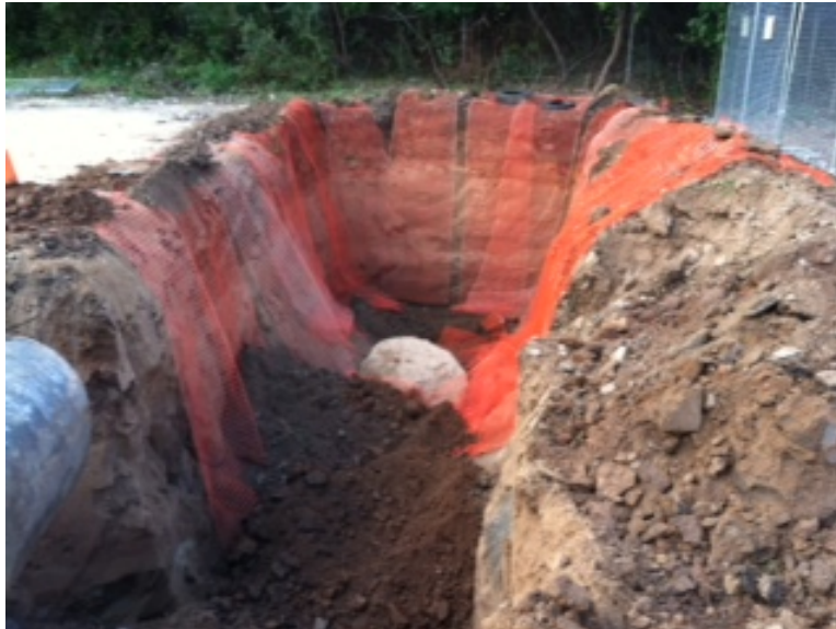
View of Operable Unit 01C (Outside Disposal Area) extended excavation in September 2012, looking south, with demarcation barrier placed and backfilling started.
