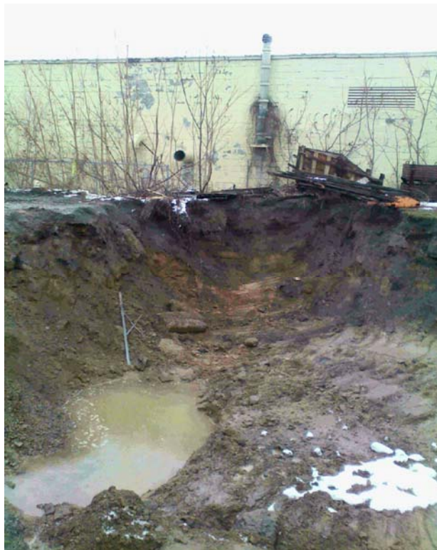
View of the northern extent of the Operable Unit 01A (Former Drum Storage Area) excavation.
