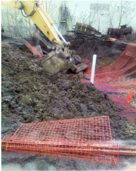
View of backfilling in the Operable Unit 01A (Former Drum Storage Area) excavation. Note the snow fence placed as demarcation barrier.
