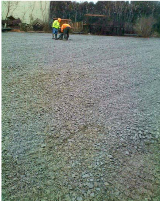
View of Operable Unit 01A (Former Drum Storage Area) backfilled. Crew is covering the well pad of INJ-1 to protect from forecasted rain.
