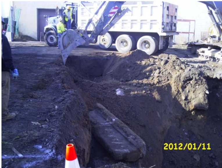
View of the southwestern portion of the Operable Unit 01A (Former Drum Storage Area) excavation. An example of the concrete that was located in the excavation is exhibited.
