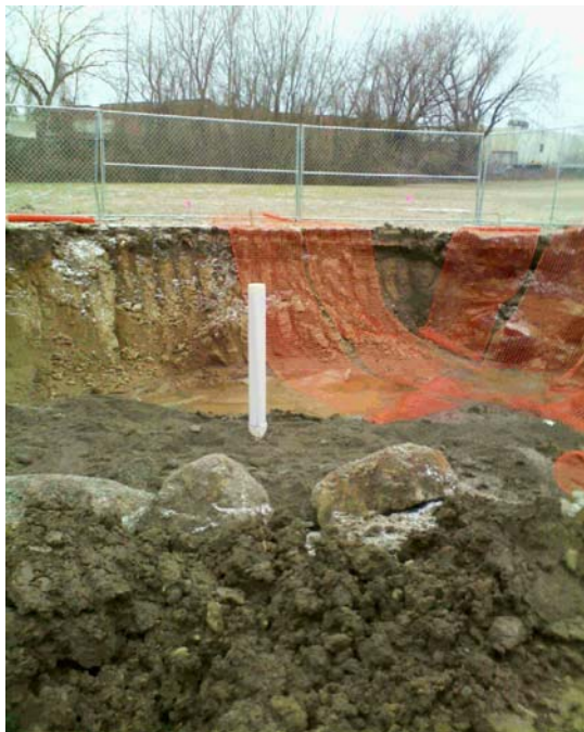
View of Injection Well INJ-2.
