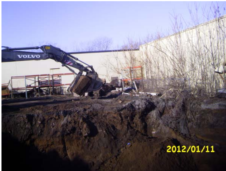
View of concrete being removed from the excavation. The concrete was set aside, and was backfilled into the excavation upon approval of completed excavation.
