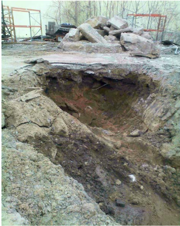
View of stockpiled concrete from the Operable Unit 01A (Former Drum Storage Area) excavation.
