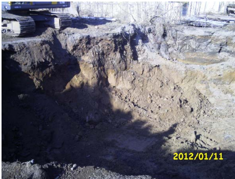
View of the northwestern portion of the Operable Unit 01A (Former Drum Storage Area) excavation, following further soil removal.
