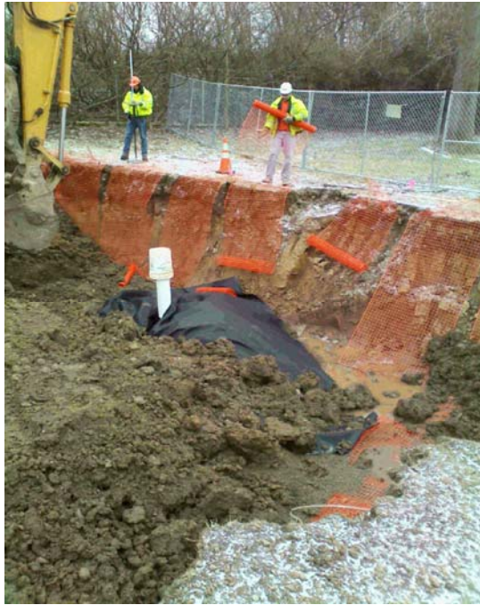
View of Operable Unit 01C (Outside Disposal Area) during backfill. Note INJ-2 and placement of demarcation barrier.
