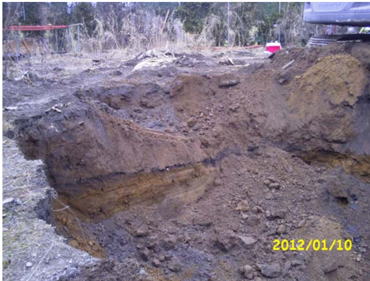
View of the eastern portion of the Operable Unit 01A (Former Drum Storage Area) excavation.
