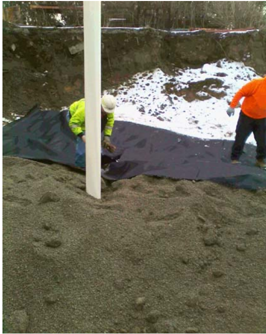
Construction of Injection Well INJ-1 within Operable Unit 01A (Former Drum Storage Area) excavation.
