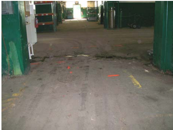
Photo No. 3. Floor drain and piping in doorway of Press Room, looking west.
