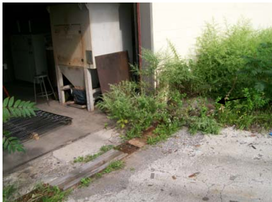
Photo No. 21. Trench drain and Southeast collection pit, southeast corner of Loading Dock.
