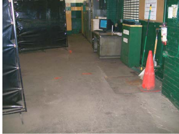
Photo No. 2. Catch basin and piping along east wall of Welding Room, looking
