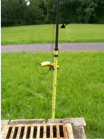
Photo No. 19. South collection pit and piping looking west.
