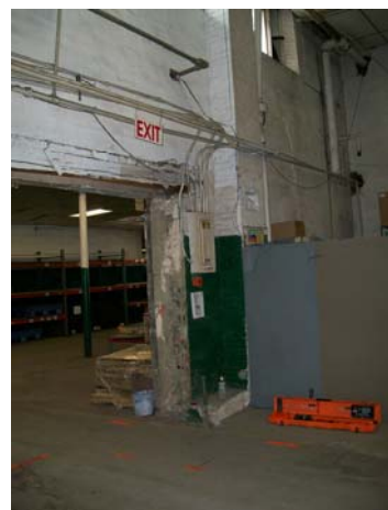
Photo No. 6. Pipes in doorway of Grinding Room and SVE system pipes north.
