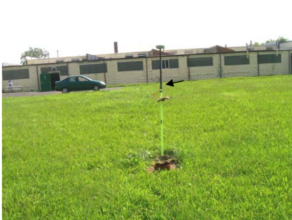
Photo No. 17. Central collection pit, piping and cleanout looking east.
