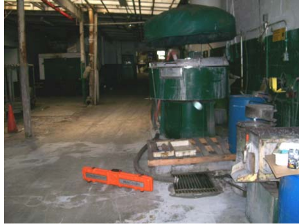
Photo No. 8. Catch basin for tumbler looking south.
