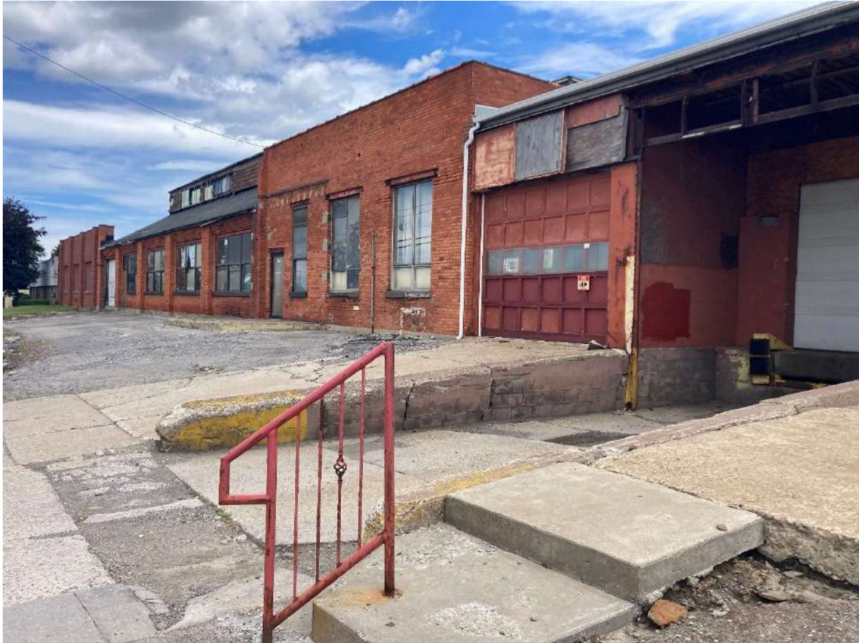
Photo 5 – Approximate location of USTs. Block wall is overturning, cracked, and fragmented (taken 7/26/22)
