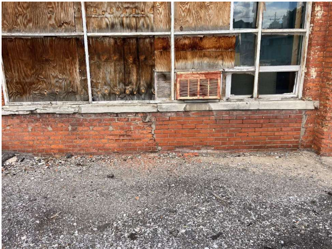
Photo 3 – Deteriorated brick and broken windowpanes on southern wall, brick debris at base (taken 7/26/22)
