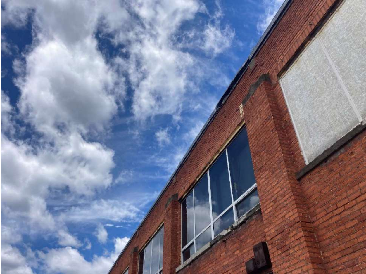
Photo 4 – Spalled portion of parapet and cracked second story window (taken 7/26/22)
