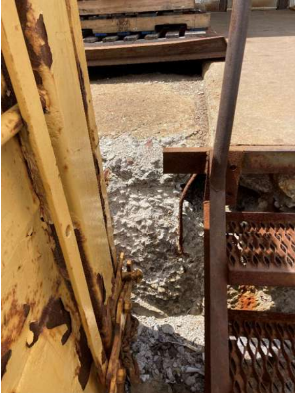
Photo 8 – Spalled conc. Loading dock (taken 7/26/22)
