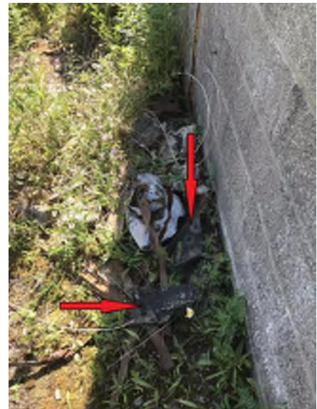
Photo 12 Black asbestos-containing debris located on the ground of the exterior of the building
