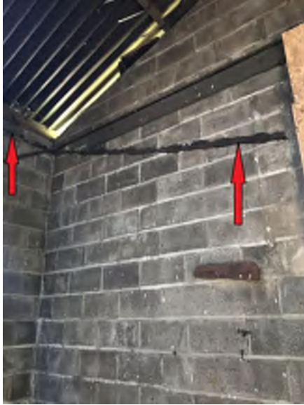
Photo 9 Black asbestos-containing roofing cement located along the CMU blocks on the interior of the building
