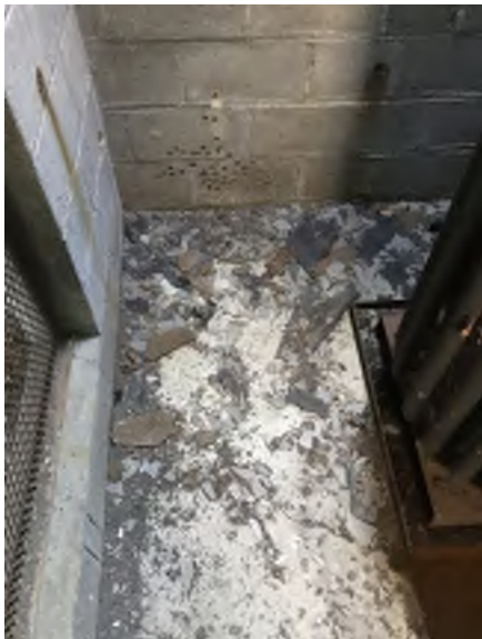
Photo 11 Black asbestos-containing debris located on the ground of the interior of the building
