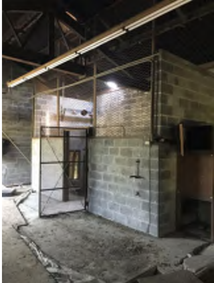
Photo 1 Building 8 interior and transformer room, looking north
