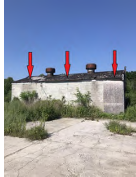
Photo 10 Black asbestos-containing tar paper located on the metal roof
