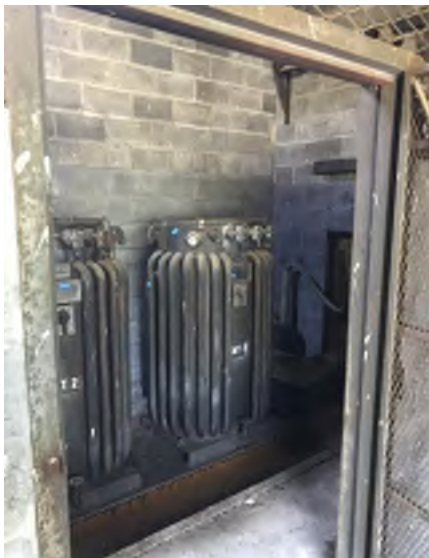
Photo 3 Transformer room interior
