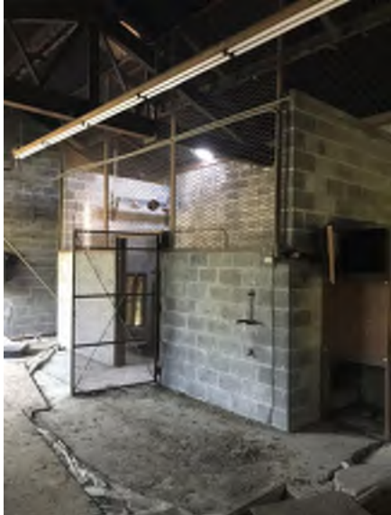
Photo 1 Building 8 interior and transformer room, looking north
