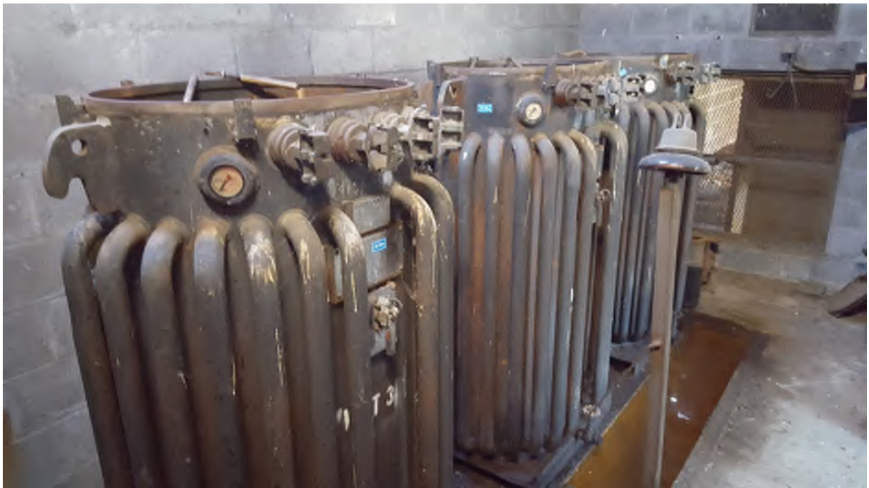
Transformers within Building #8
