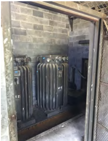
Photo 3 Transformer room interior
