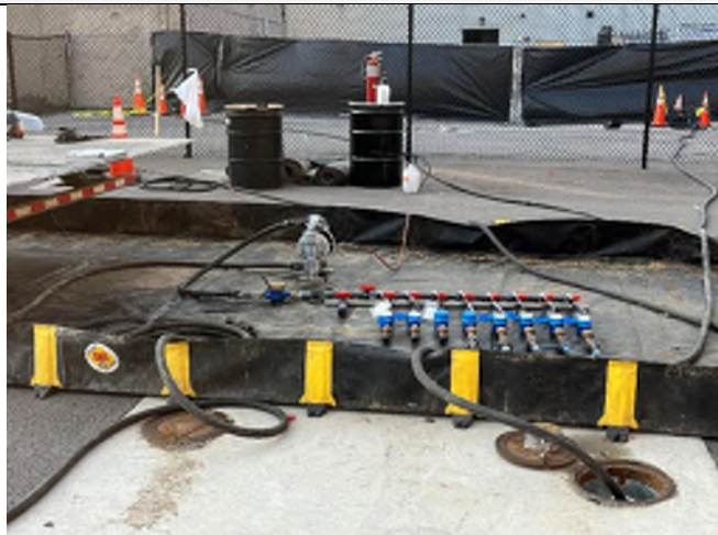
Injection well set-up
