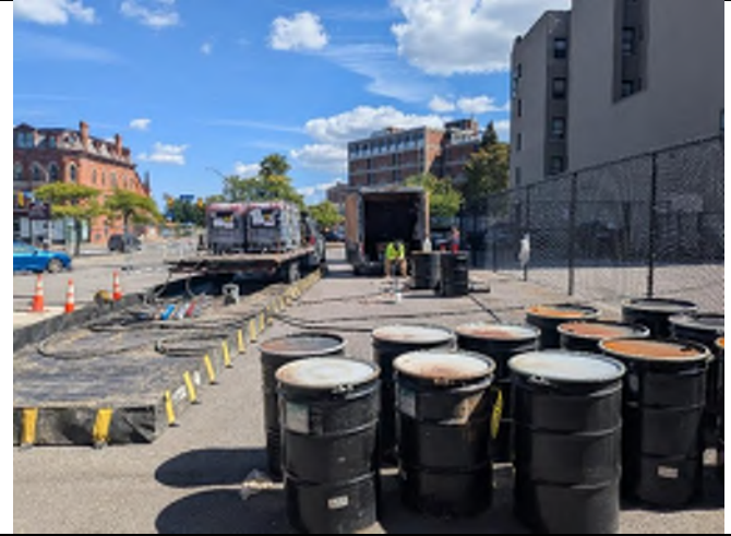
Injection setup with secondary containment.
