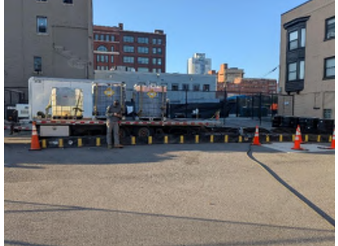
Injection setup with secondary containment.
