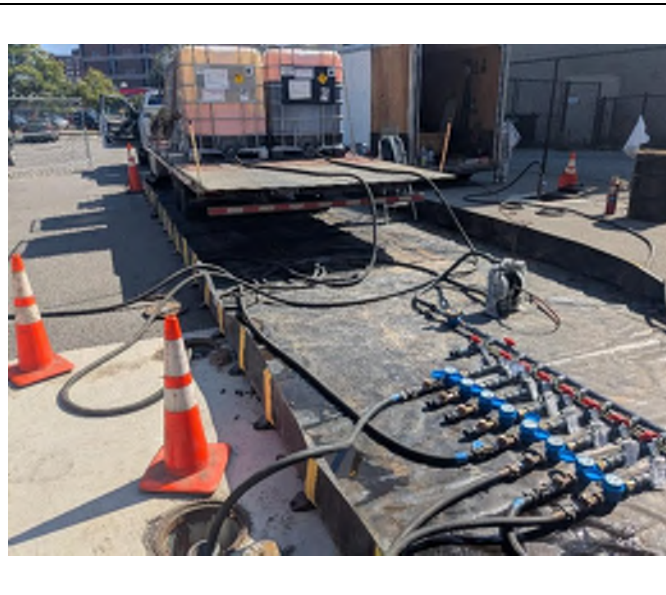
Injection manifold set-up inside secondary containment.
