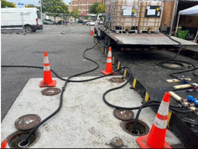
Injection setup with secondary containment.
