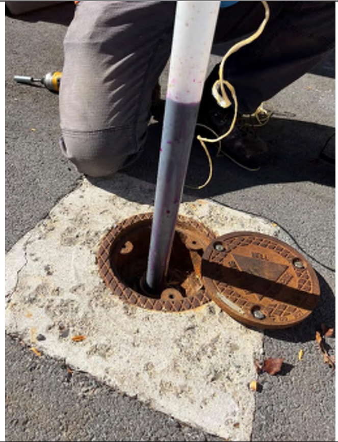
MW-3S with dark purple injection material visible.
