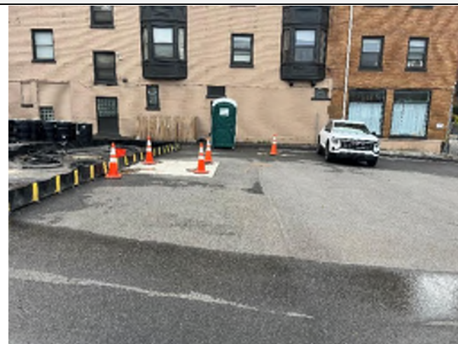
Injection setup with secondary containment.
