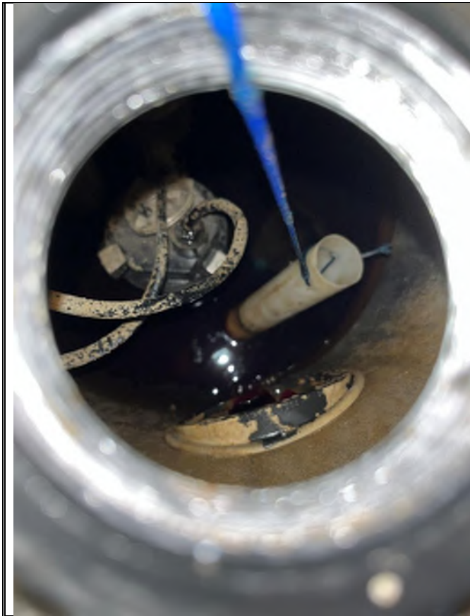
Bailer with thiosulfate crystals in sump pump.
