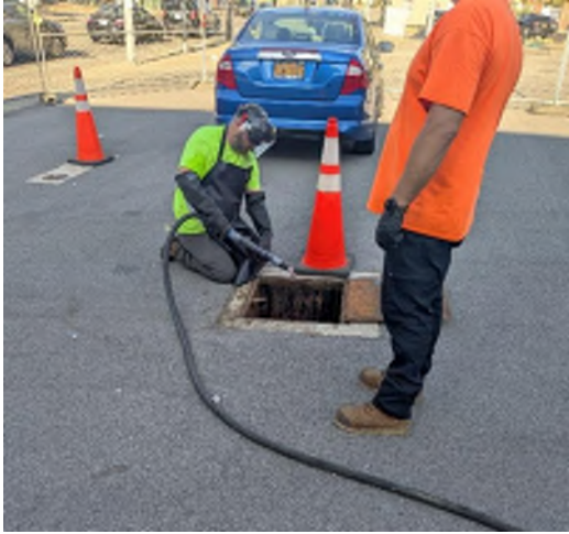
Connecting injection manifold to injection well at IW-4.
