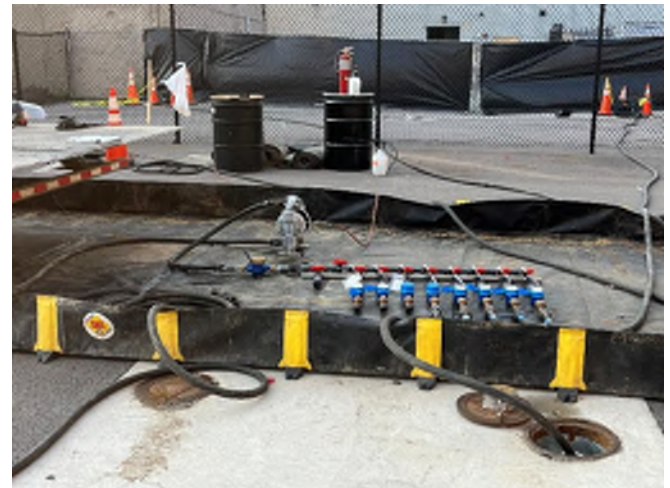
Injection manifold set-up inside secondary containment.
