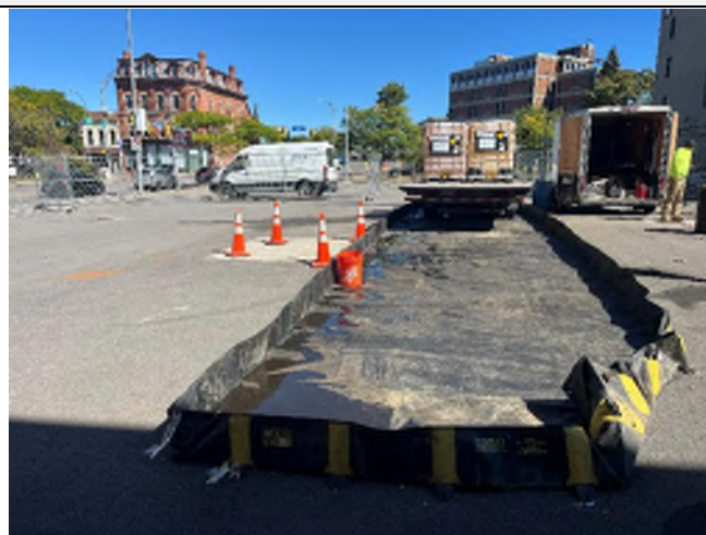
Injection setup with secondary containment.
