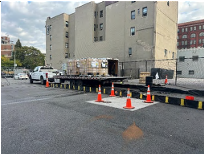
Injection setup with secondary containment.
