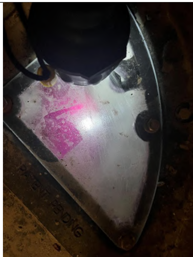
Pinkish water in sump pump in basement.
