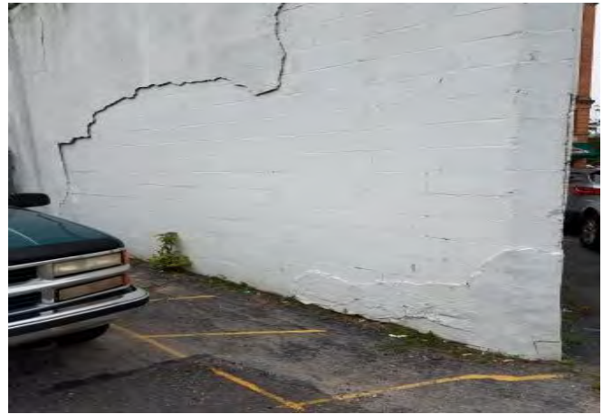
HA-32: Exterior Parge Coat
