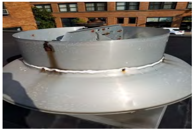
HA-49: White Repair Caulk
