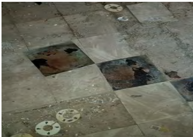
HA-25: Composite: Black Mastic and Vapor Barrier
