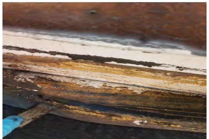
HA-47: Tan Adhesive from Rubber Roofing System
