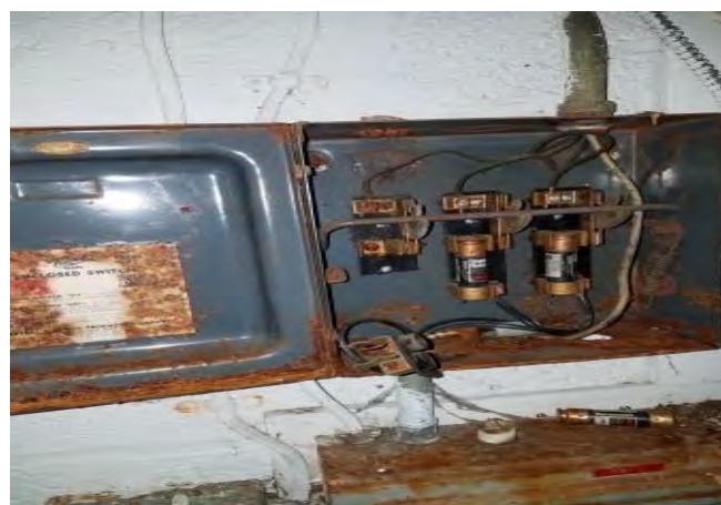
HA-26: Black Electrical Switch
