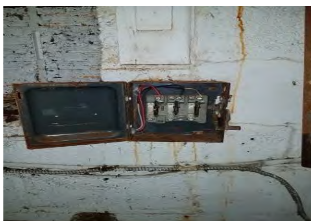
HA-27: Gray Electrical Switch
