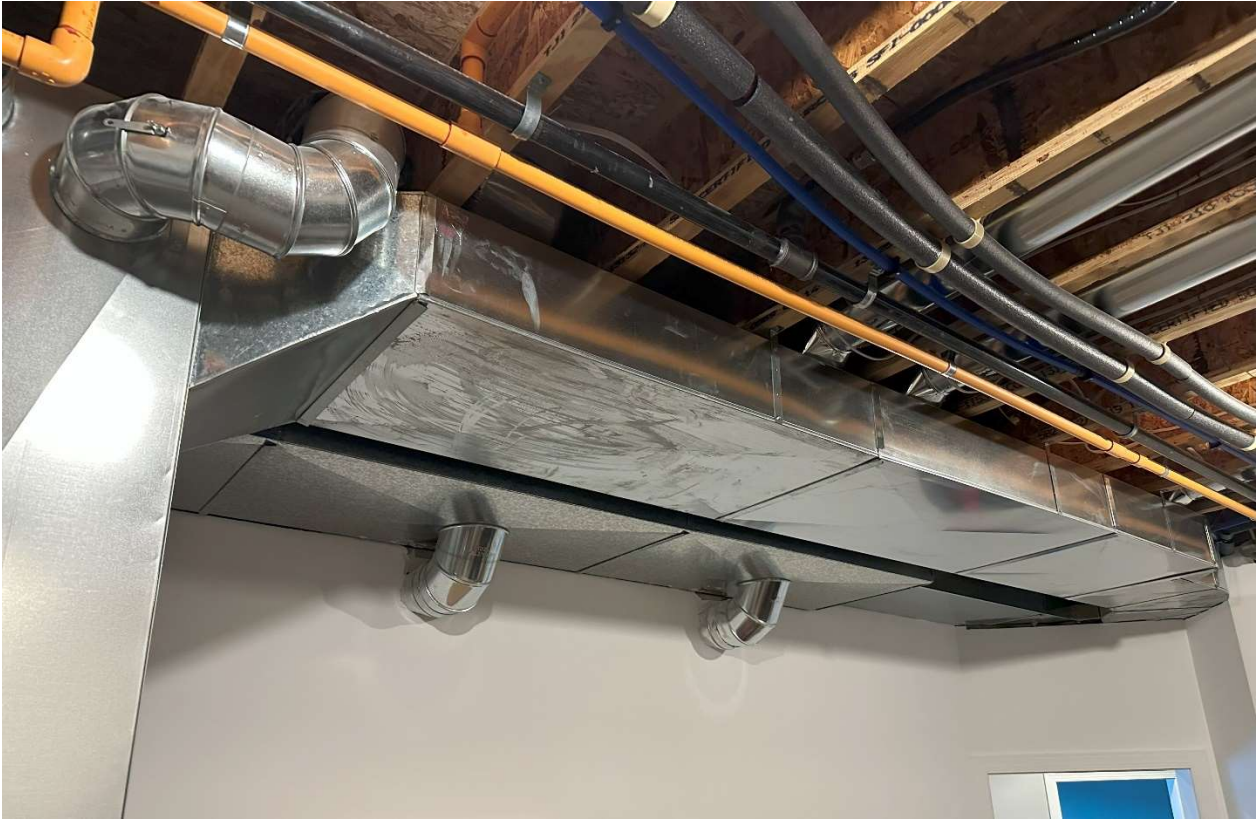
Photo 2 – HVAC Ductwork (typ.)
