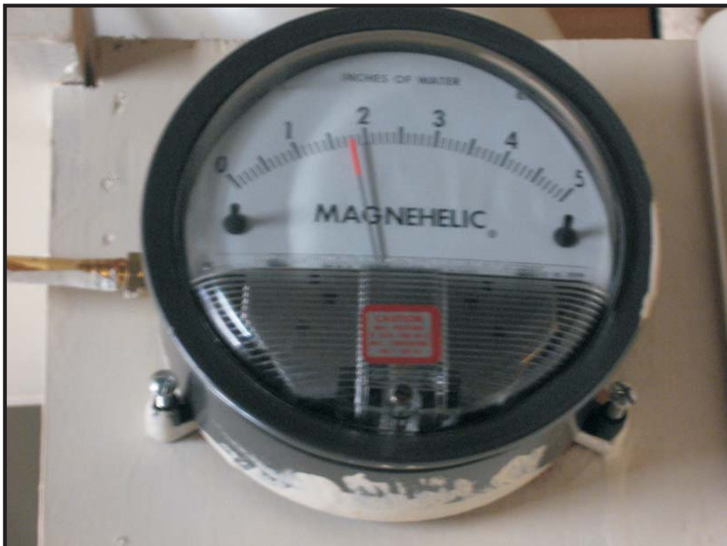
Photo 2: VFW suction point #2 magnehelic.
