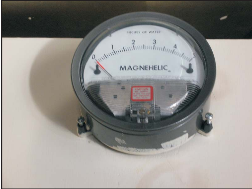
Photo 1: VFW suction point #1 magnehelic.
