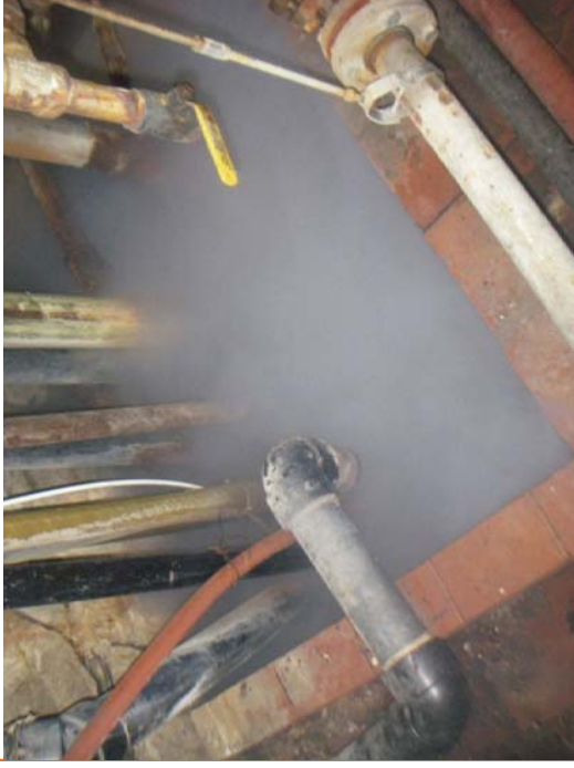
Photo 13. Outfall 005: Smoke observed at 005-001A near former Hotwell 4
