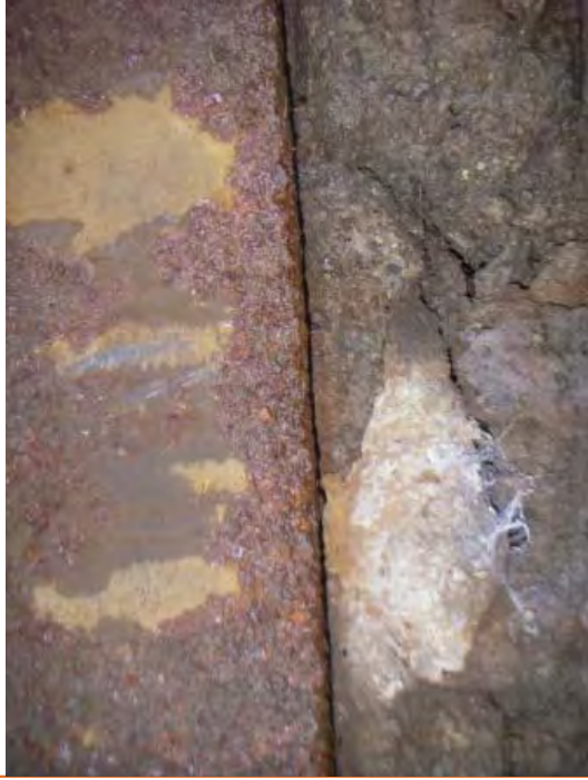
Photo 101. Outfall 004: 004-001 Manhole defects; frame/chimney seal deterioration
