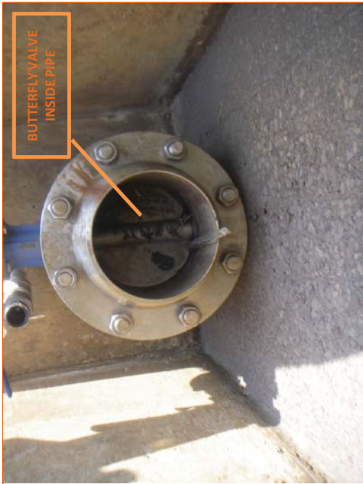
Photo 36. Outfall 010: 6" Diameter discharge point 010-000
