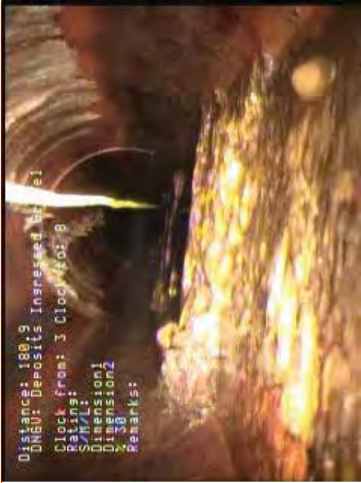
Photo 52. Outfall 004 (004-001A to 004-001): Gravel debris at 194 ft upstream of 004-001
