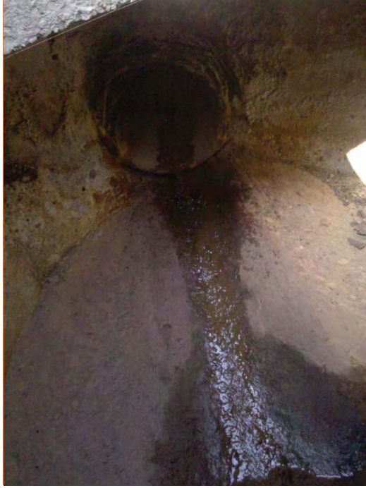
Photo 95. Outfall 001: 001-001 Pipe connections (north pipe)
