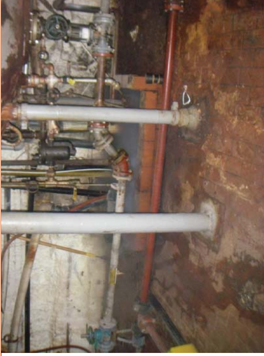
Photo 12. Outfall 005: Smoke observed at 005-001A near former Hotwell 4
