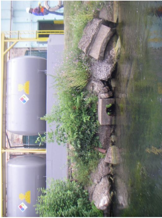
Photo 41. Abandoned historical outfall located approximately 20 ft east of Outfall 005. Seems to correspond to historical pipe No. 10. See Figure 6.
