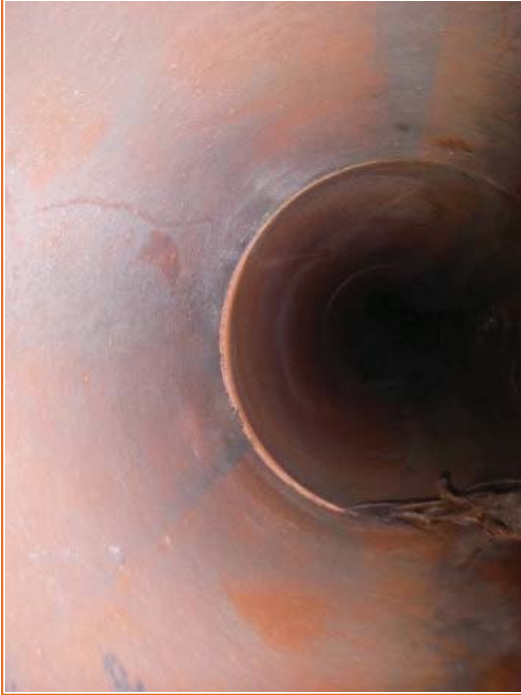
Photo 103. Outfall 004: 004-001 Pipe connections (north pipe)
