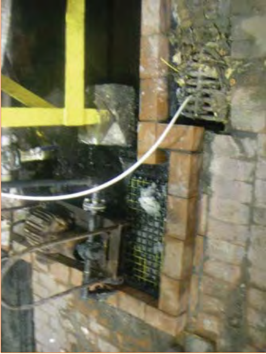
Photo 119. Outfall 004: 004-005 Floor drain in MPA Process Area
