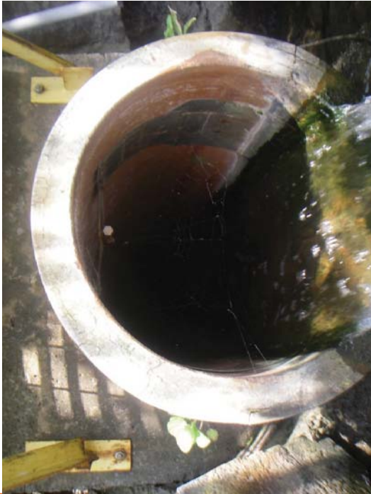
Photo 25. Outfall 004: Interior of 24" diameter discharge point 004-000 piping
