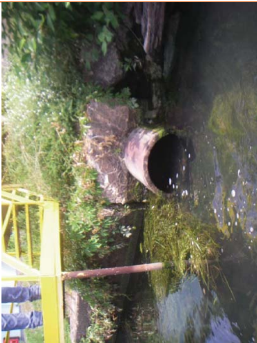
Photo 26. Outfall 005: 28" Diameter discharge point 005-000 piping
