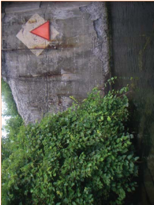
Photo 32. Outfall 007 (Historical pipe No. 18): Could not locate discharge point 007-000. It may underlie area with vegetation.
