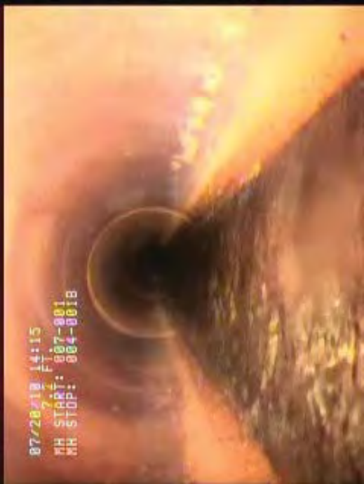
Photo 62. Outfall 004 (007-001 to 004-001B): Facing downstream (west) from 007-001
