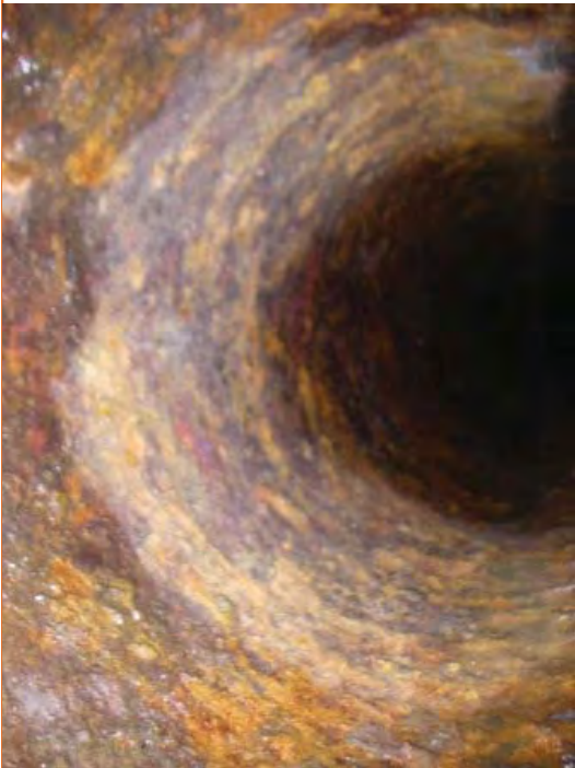
Photo 116. Outfall 007: 007-001 Pipe connections (north pipe)
