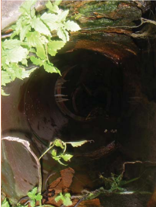
Photo 43. Abandoned historical outfall located approximately 20 ft east of Outfall 005. May correspond to historical pipe No. 10. See Figure 6.
