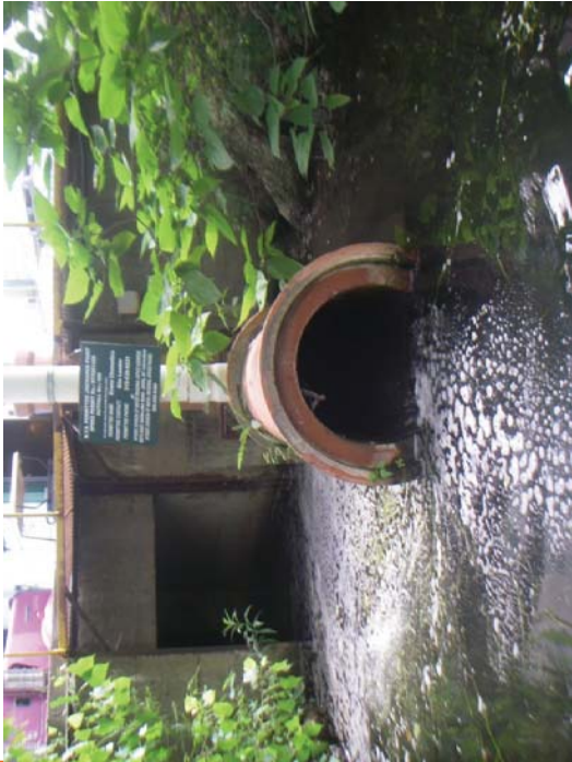
Photo 33. Outfall 008: 24" Diameter discharge point 008-000
