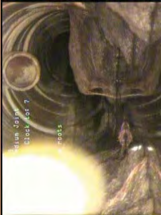
Photo 75. Outfall 008 (008-001 to 008-000): Break-in tap at 27 ft upstream of 008-000
