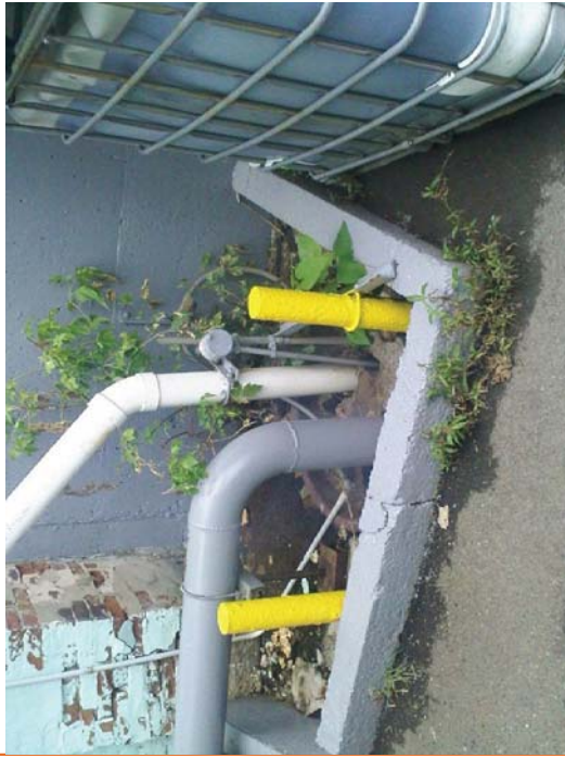
Photo 9. Outfall 005: Perforated metal plate at 005-001
