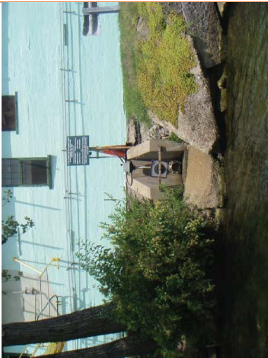
Photo 34. Outfall 009: 6" diameter discharge point 009-000. Pipe above canal water level.
