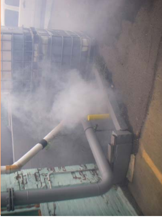
Photo 11. Outfall 005: Smoke observed at perforated metal plate at 005-001
