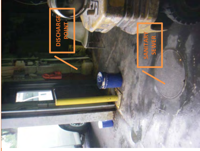
Photo 133. Building 2-A noncontact cooling water discharge point to Outfall 004 and sanitary sewer 004-008
