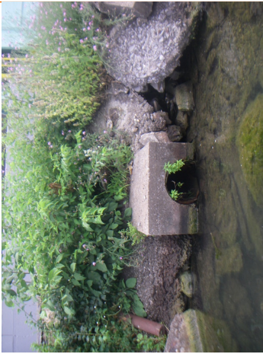
Photo 42. Abandoned historical outfall located approximately 20 ft east of Outfall 005. May correspond to historical pipe No. 10. See Figure 6.
