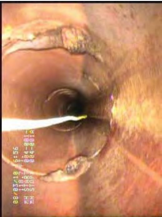
Photo 53. Outfall 004 (004-001A to 004-001): Attached deposits at 121 ft upstream of 004-001
