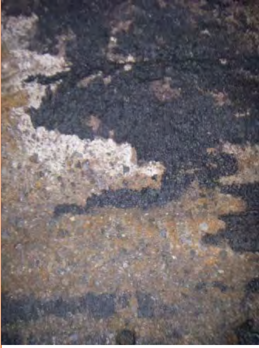
Photo 100. Outfall 004: 004-001 Manhole defects; wall deterioration
