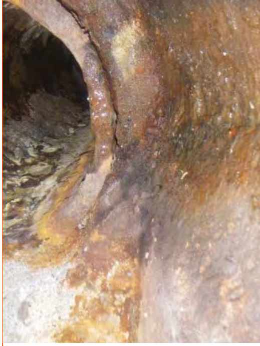
Photo 96. Outfall 001: 001-001 Pipe connections (north pipe)
