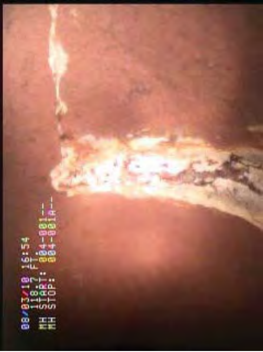
Photo 54. Outfall 004 (004-001A to 004-001): Longitudinal crack, 12 o'clock at 118 ft upstream of 004-001
