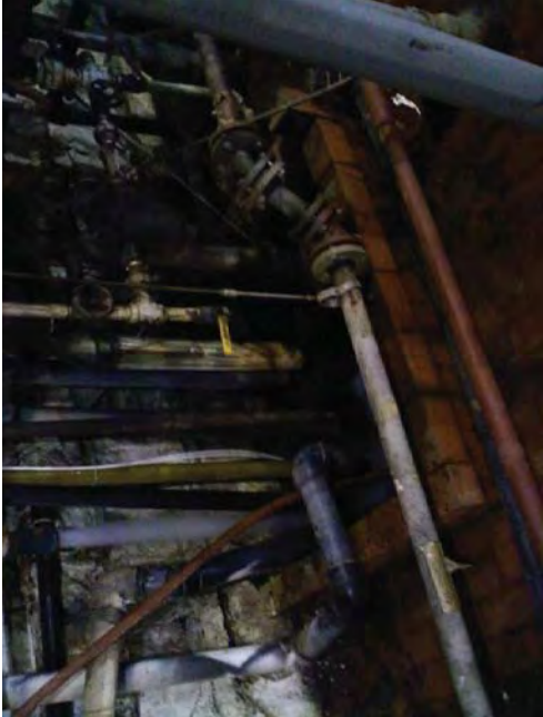
Photo 139. Former Hotwell 4; open pit with various inlet piping
