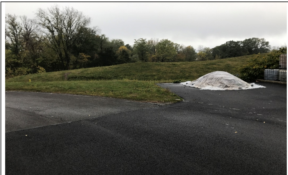
Northern side and eastern end of SWMU-1 and asphalt cap area (looking south).
