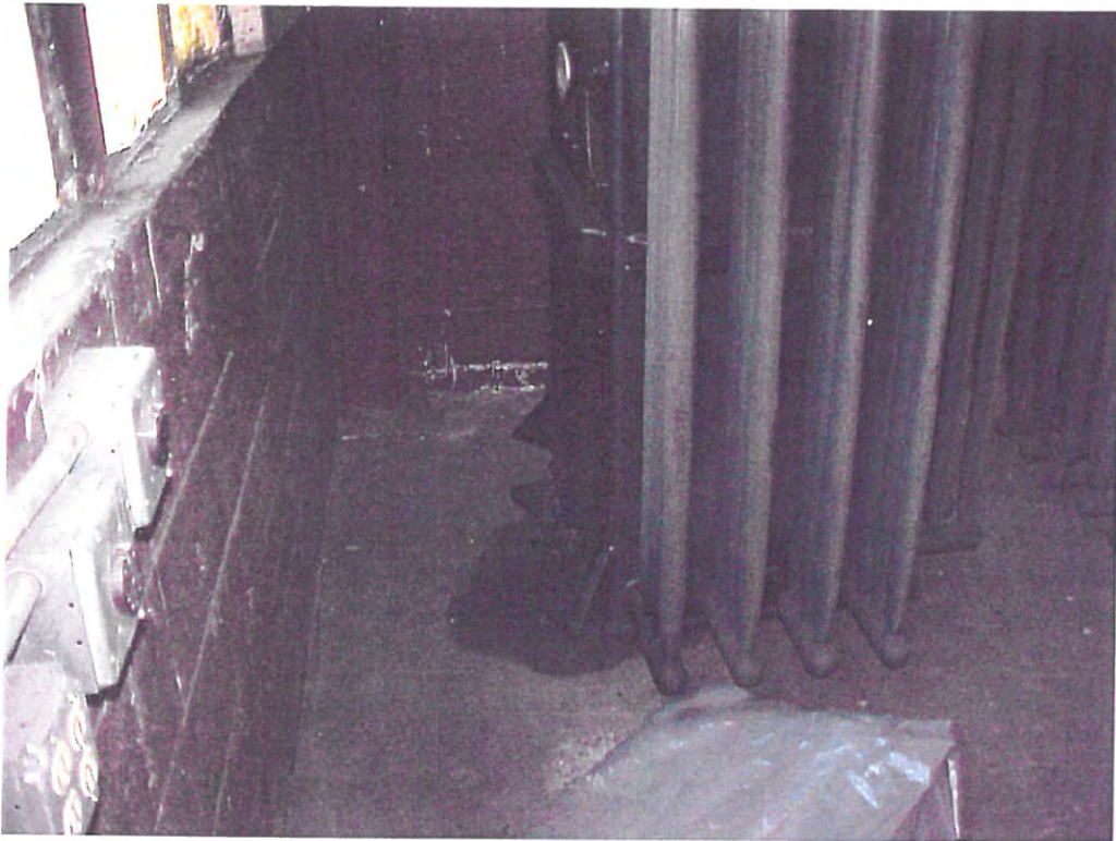
1. Transformer fluid leaking on floor in Building 8.
