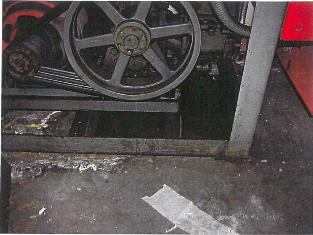
23. Closeup of hydraulic unit with tray below containing oil.
