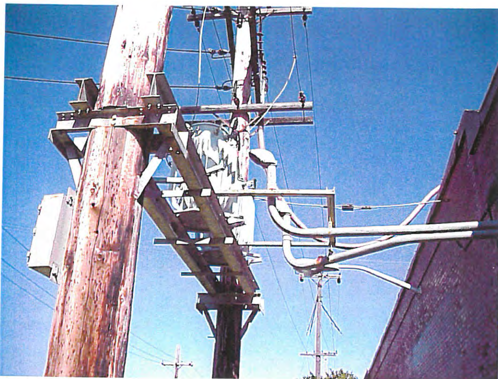
5. Substation D (disconnected).
