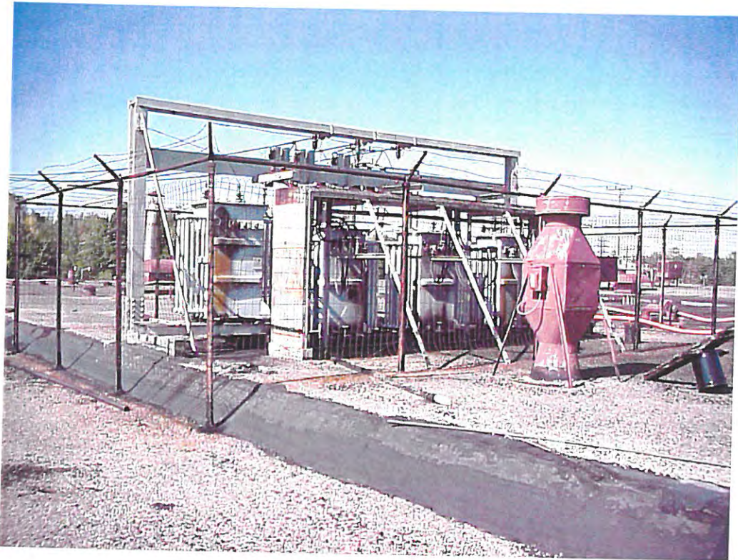
7. Another view of Substation F with three original transformers and fourth (to the left) added later.
