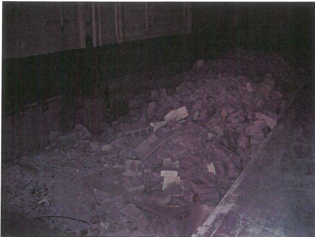
9. Debris-filled pit formerly used to house annealing ovens in Building 11A.
