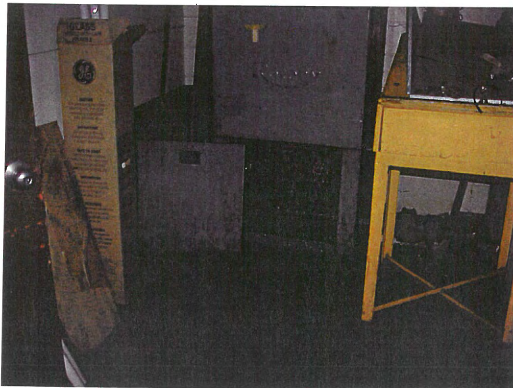
26. Hydraulic unit in Building 10 with panel removed.
