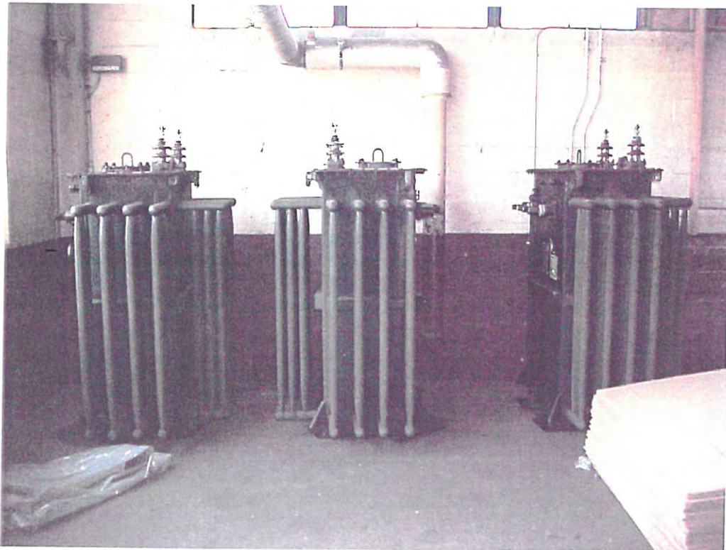
2. Three offline transformers stored in Building 8.
