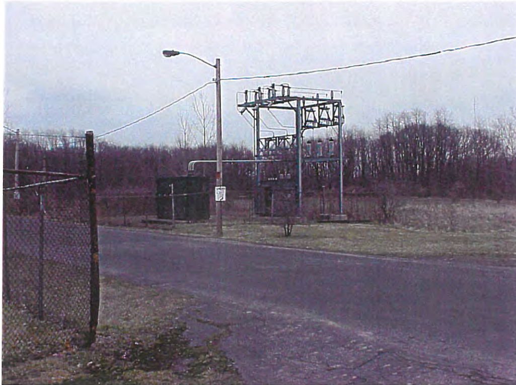
15. Substation Z as seen from across the road.
