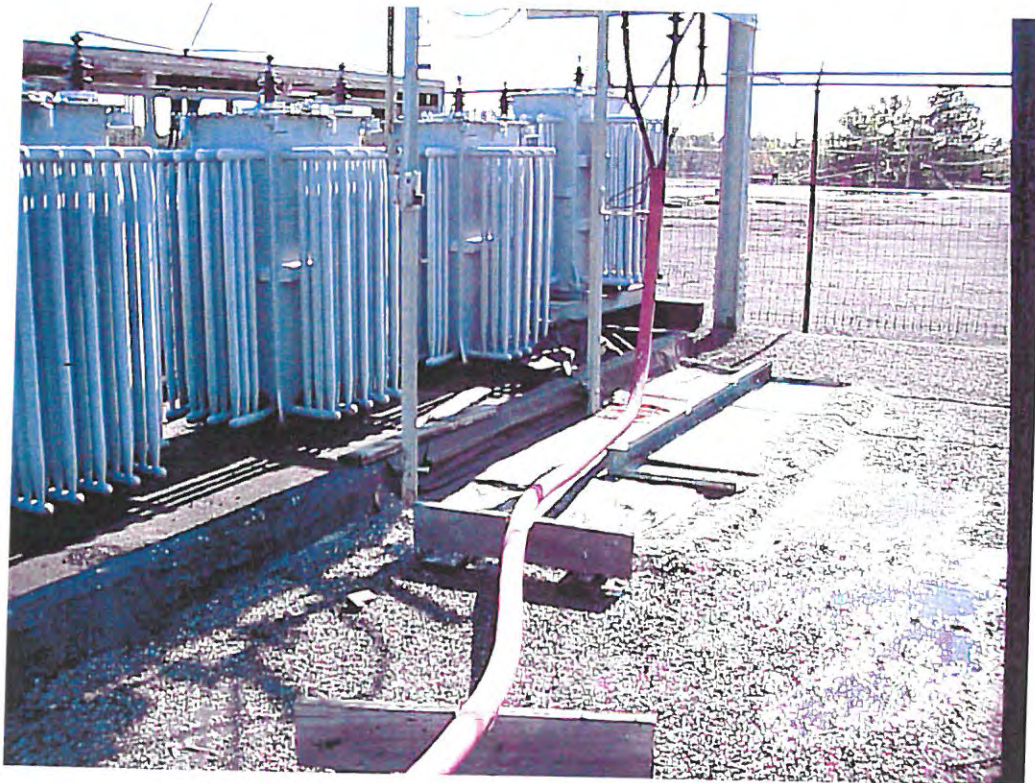
8. Back side of Substation F with oily staining in containment.
