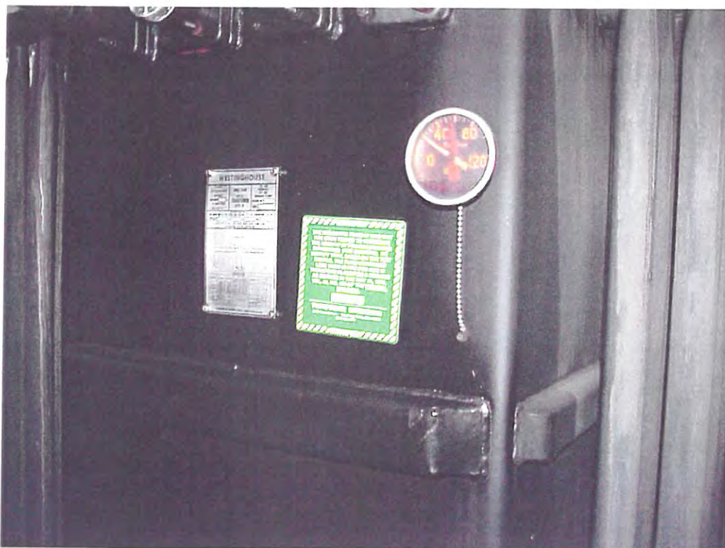
3. Non-PCB label on side of offline transformer.
