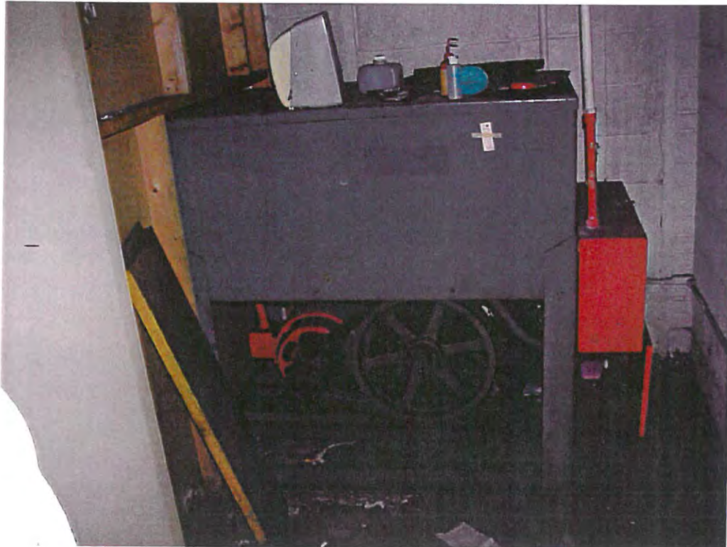
22. Hydraulic reservoir and motor for elevator in Building 2.
