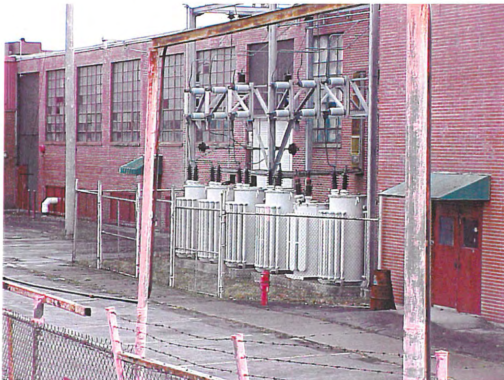
16. Substations H and J.
