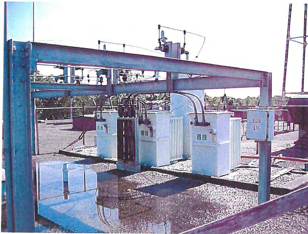
10. Non-PCB labels on transformers at Substations K and L.
