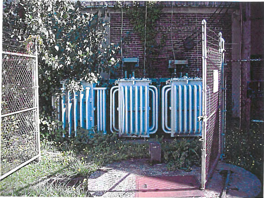
11. Substation C in courtyard.
