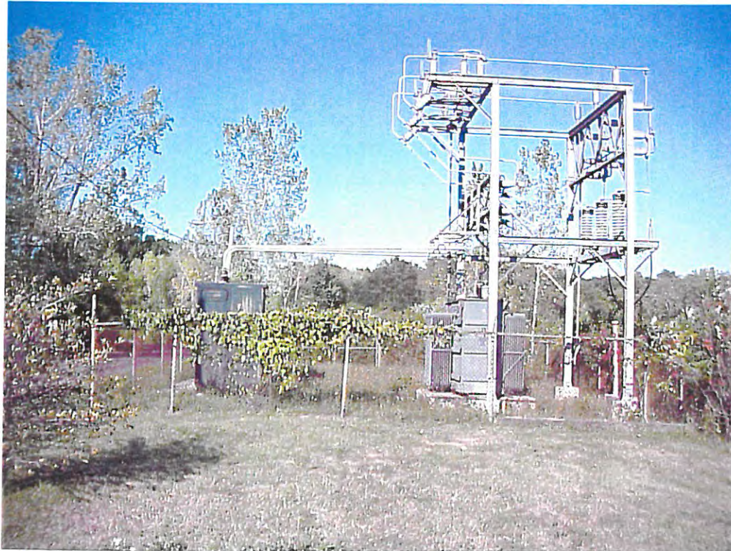
14. Substation Z located southeast of Building 13 (may be owned by NYSE&G).
