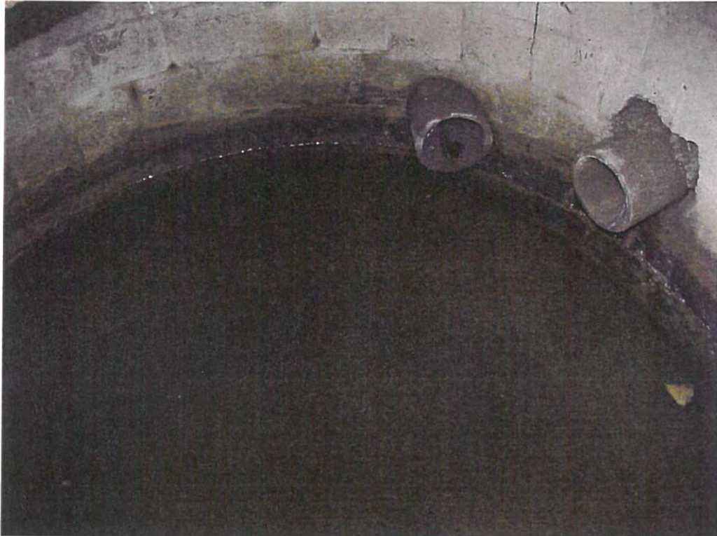
5. Cistern in the courtyard (note frog living in pipe).
