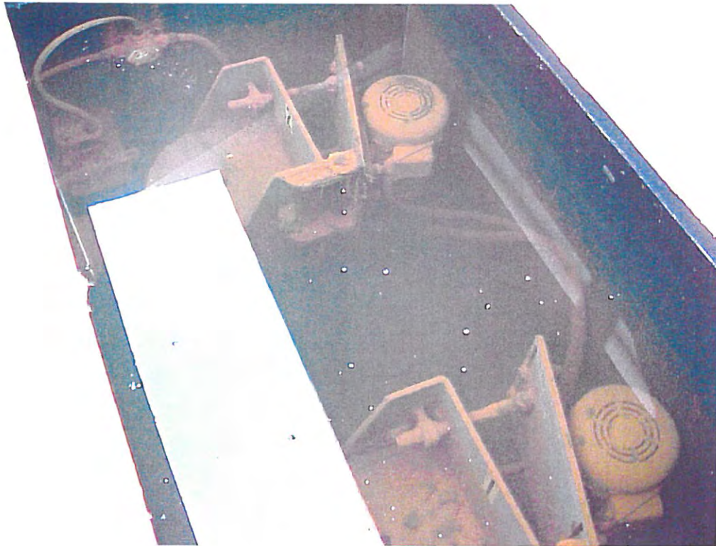
1. Sprinkler pumphouse pit full of water.
