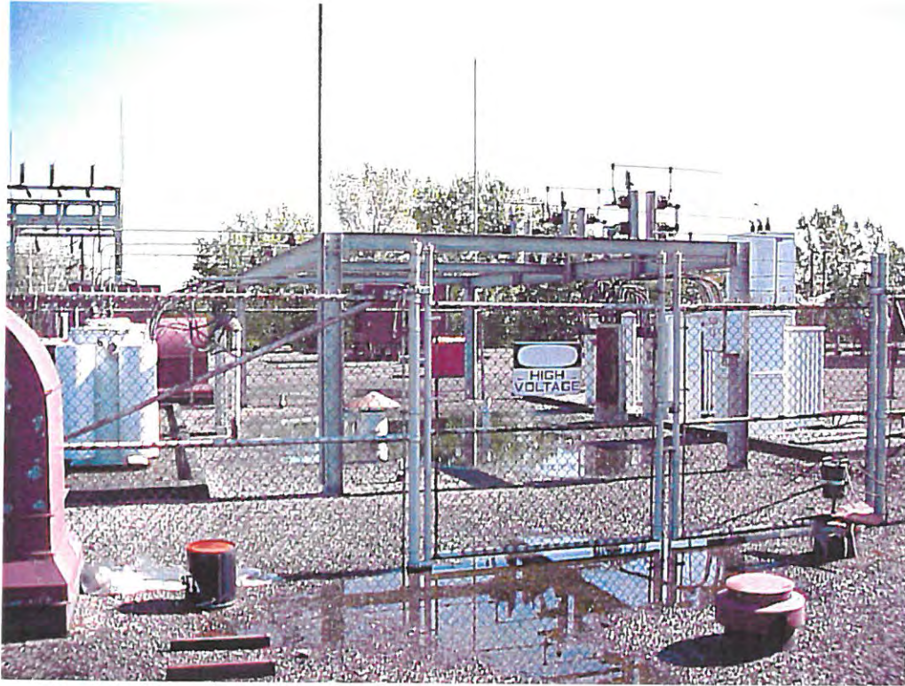
9. Substations K and L.
