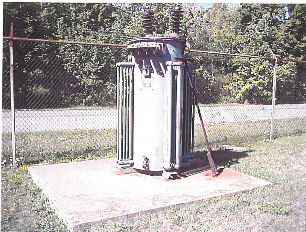
4. Offline transformer stored on former oxygen pad outside of Building 8.
