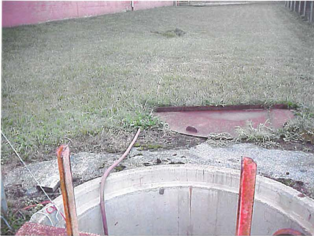
17. Hose leading to catch basin from sanitary lift station.
