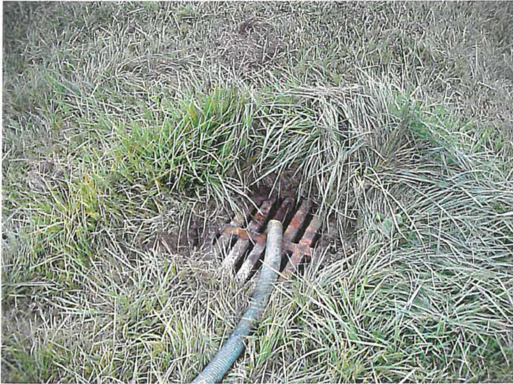
19. Hose that discharges to catch basin.
