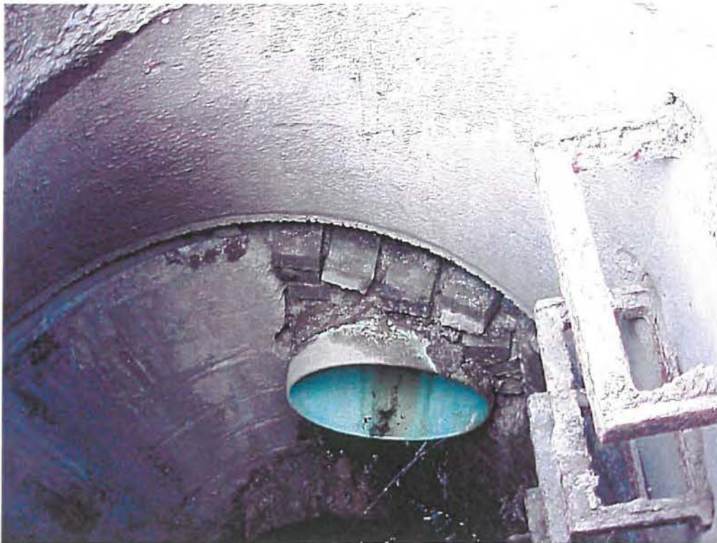
20. Example of a storm sewer where the PVC pipe tie-in is not cemented in well.
