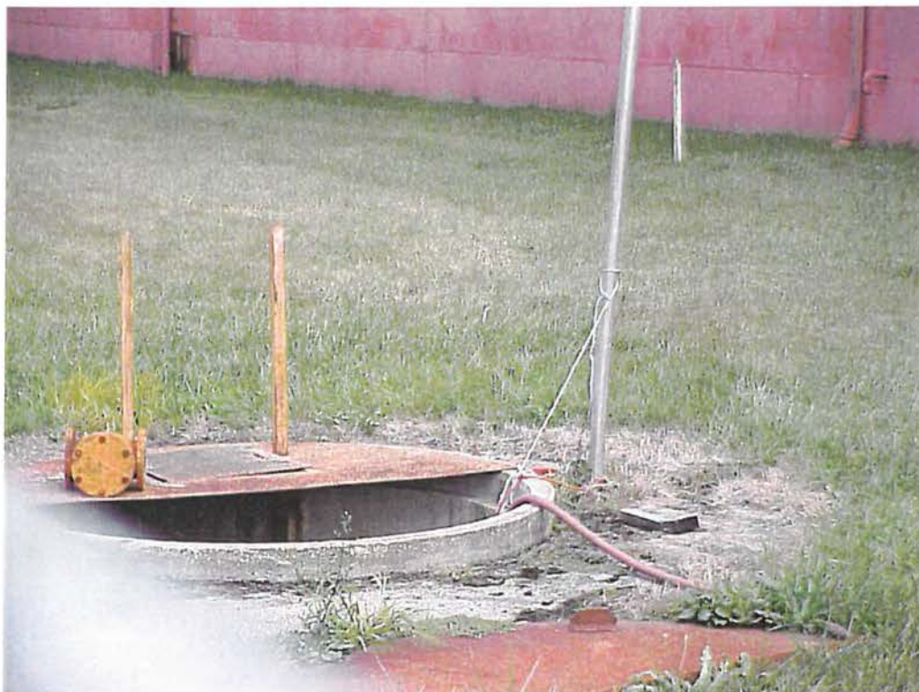
7. Sanitary sewer lift station north of Building 10A.
