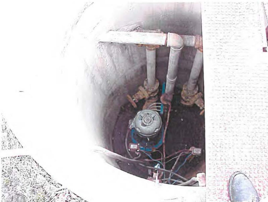
16. Looking down into sanitary lift station –sump pump and hose to pump out groundwater.
