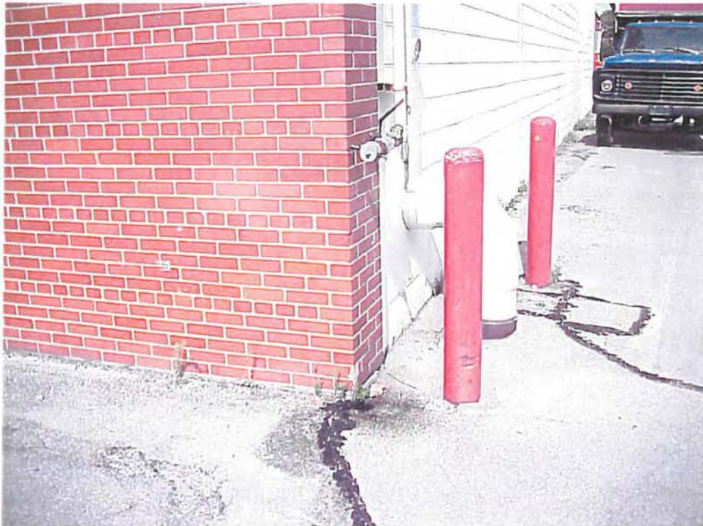
1. Former TCE standpipe with locking cover and valve, located on the corner of Building 11A.
