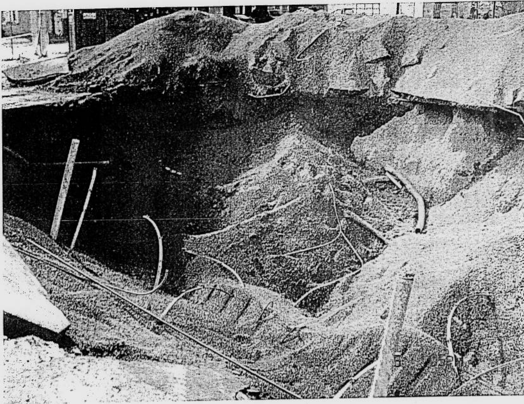
Photo 3: View Southwest of gasoline tanks excavation after removal of gas tanks. Pea stone was dry with no evidence of contamination.
