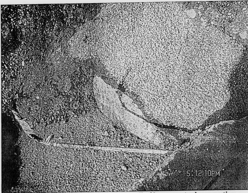
Photo 8: View Northwest of north wall of kerosene tank excavation (south end of abandoned-in-place steel kerosene tank visible).
