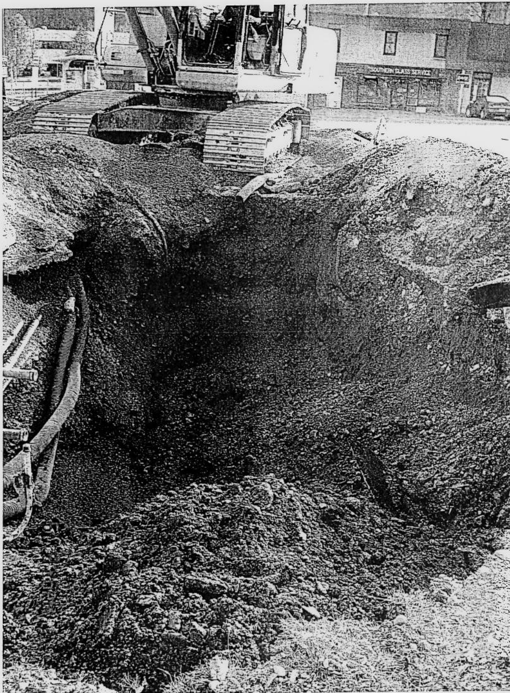
Photo 7: View South of kerosene tank excavation after south wall was scraped to native soils. Walls and bottom of excavation show no evidence of contamination.
