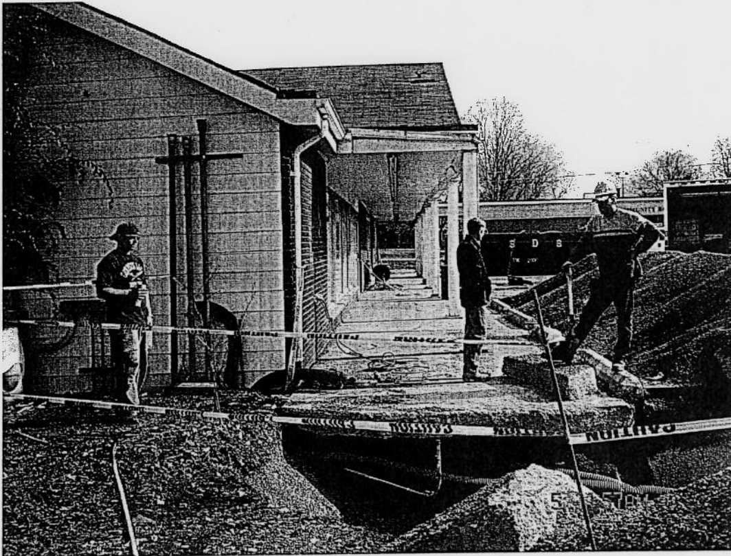
Photo 1: View East, along front of store. Kerosene tank excavation area in foreground.
