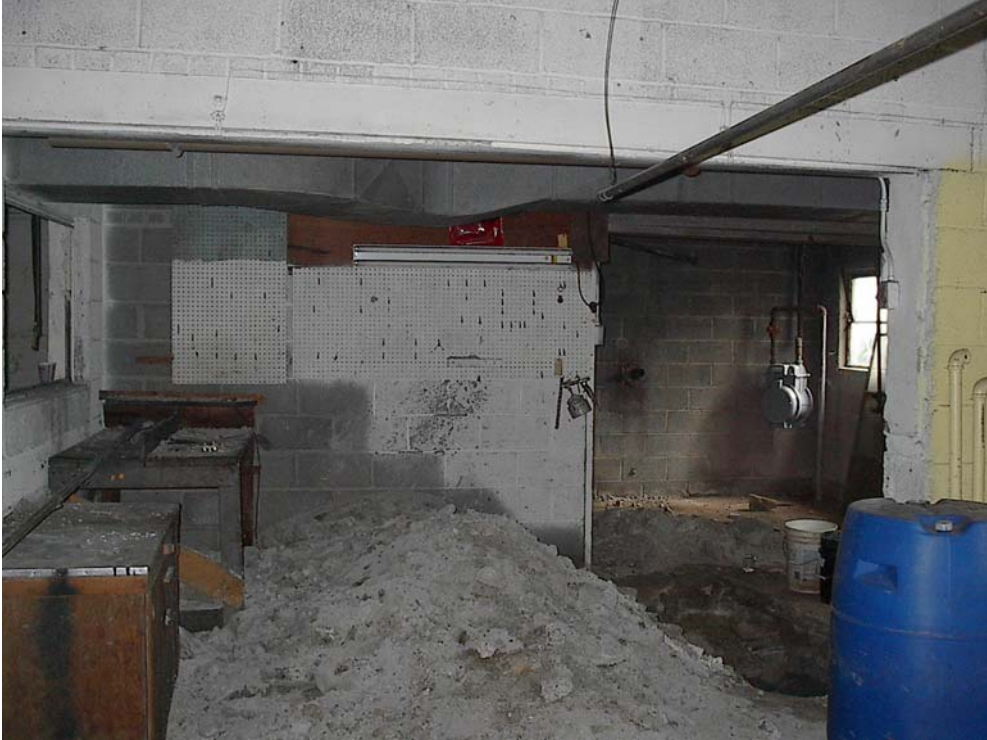
Looking north at northeast corner of Site Building. (Hole for excavation/sampling of former solvent/fuel tank by United Environmental Group, Inc.). Building soil sample collected from below this underground tank.
