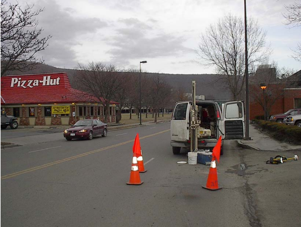
Looking east along East Pulteney Street, across from Loohn's Corning Site. Geoprobe is set up to collect soil gas sample GV-2.
